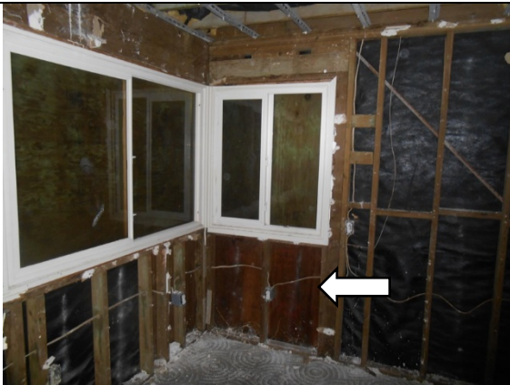
PA1CD.4: Building paper missing at interior face of wall sheathing.
