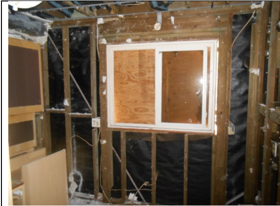
PC1CD.1: Missing opening king post.
