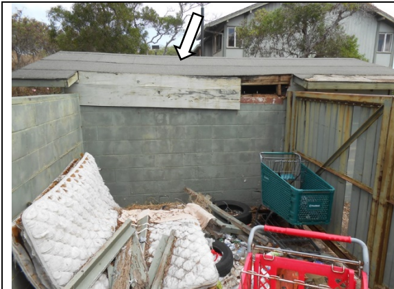
PTESB4: Damaged storage building roof.
