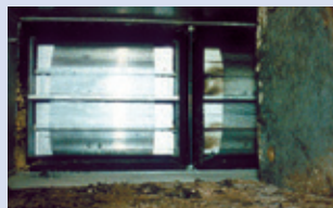
Photo 4C: Moldy air duct
