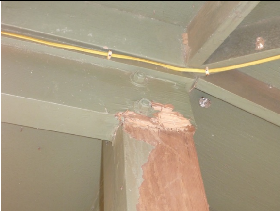
RCRD.1: Moderate termite damage present at beam to column connection at Gridlines '5-D'.
