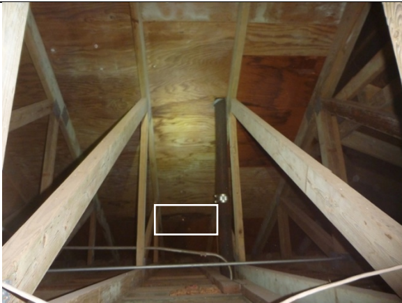
RCRD.2: Region of damaged plywood sheathing.
