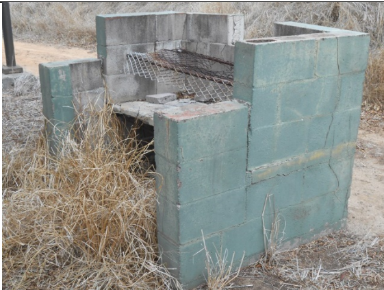
PBP2: Damaged concrete masonry unit barbecue pit. Missing blocks, cracked masonry, and warped concrete fire slab.
