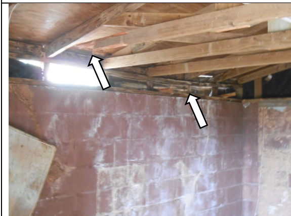
PTESB6: Collapsed storage building south wood framed stem wall. Damaged truss bottom chord.
