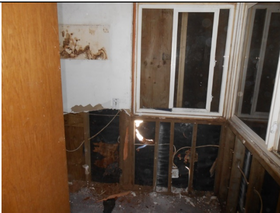
PB1D.2: Siding dry rot.
