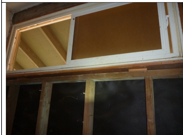
RC1CD.2: At various locations, windows are supported on spaced blocks.
