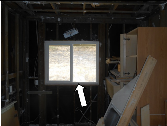
PC2CD.3: Missing opening sill plate.
