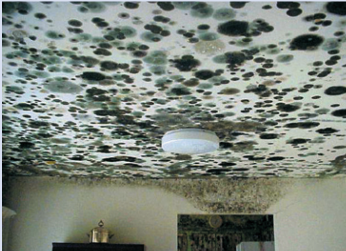
Photo 2: Extensive mold contamination of ceiling and walls
