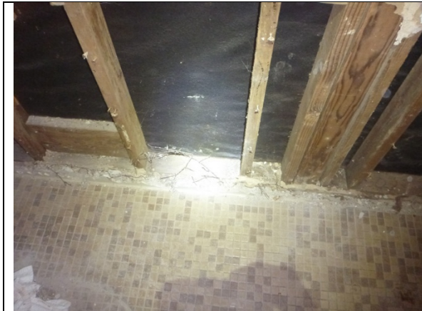
RC1CD.1: At various locations, sole plate anchor rods are installed at more than 32 inches on-center or missing.
