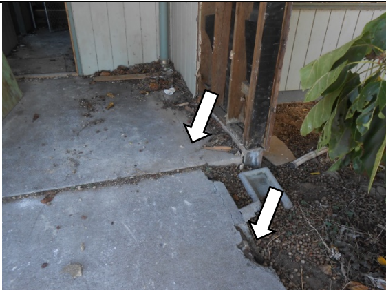
PA1D.5: Cracked exterior slab at rusting drain-pipe.
