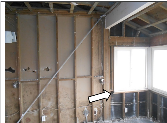
PC2CD. 1: Missing opening king post.
