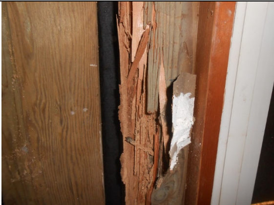
PB1D.3: Post termite damage.
