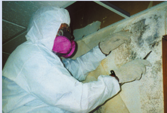
Photo 7: Remediation worker with limited PPE
