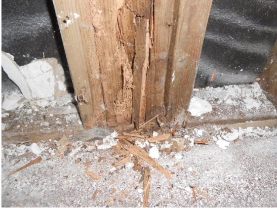
PC1D.4: Post termite damage.
