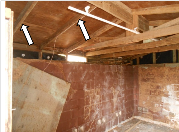
PTESB7: Damaged trusses. Missing truss framing.
