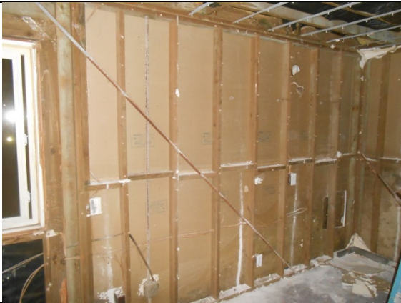
PB1D.6: Rusting steel wall braces.
