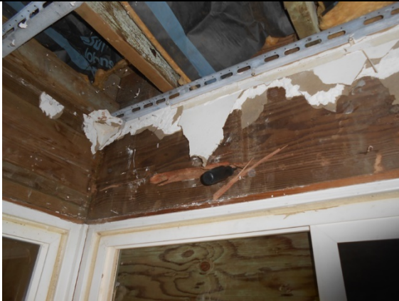
PB1D.5: Beam termite damage.
