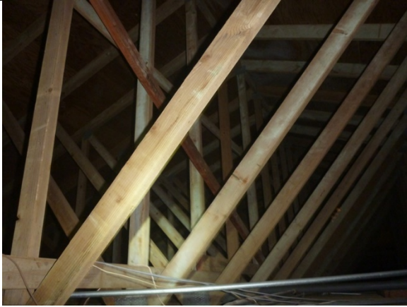
RCRCD.1: Web bracing missing.
