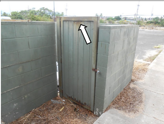
PTESB3: Rusting trash enclosure door.
