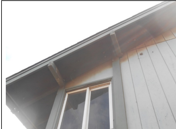
PCRD.1: Beam overhang dry rot.
