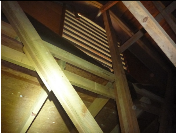
RCRCD.2: Gable end wall missing stud wall framing.
