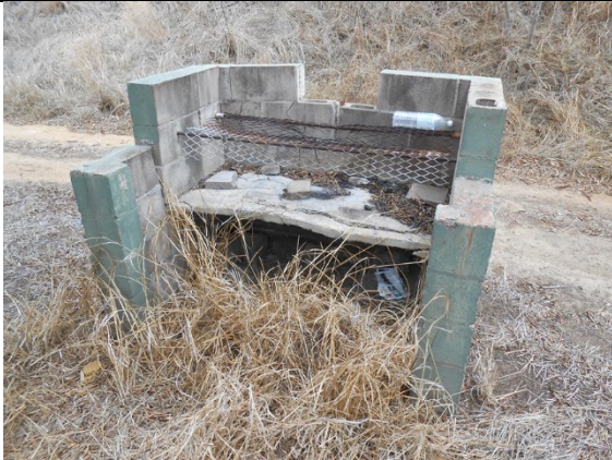
PBP1: Damaged concrete masonry unit barbecue pit. Missing blocks, cracked masonry, and warped concrete fire slab.
