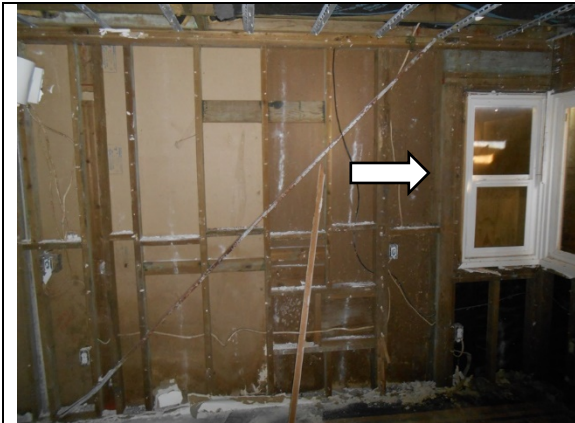
PA1CD.6: At various locations, openings missing king jamb post(s).
