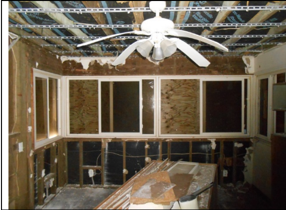
PB2CD.2: Missing blocking
