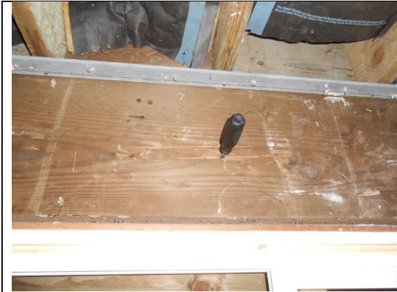
PC2D.1: Beam termite damage.
