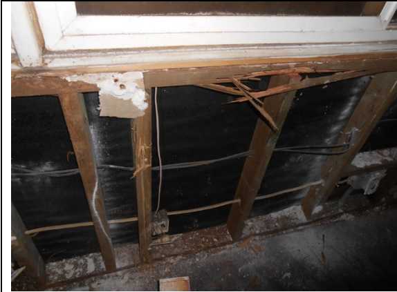
PB1D.4: Stud termite damage. Sill plate termite damage.
