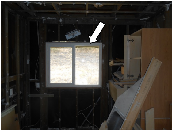
PC2CD.4: Missing opening header.
