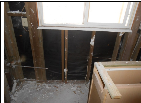
PB2CD.1: Missing wall blocking.
