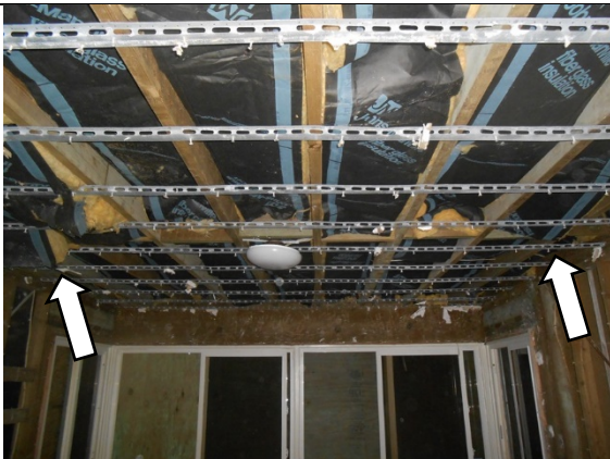
PA2CD.3: Missing wall blocking.
