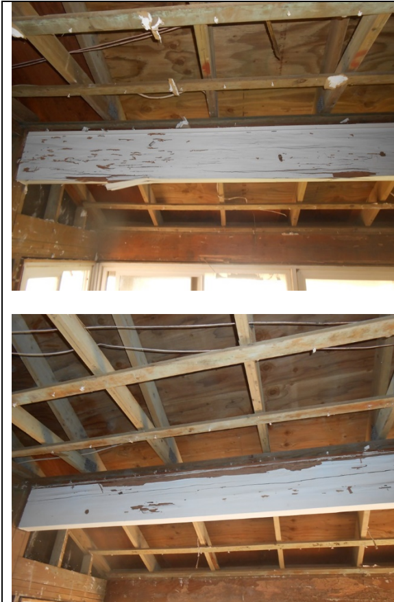
PBRD.1: Beam termite damage.
