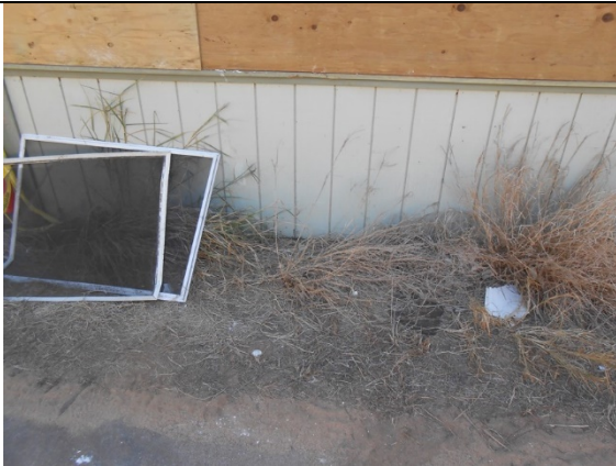
PB1CD.4: Vegetation against building façade.
