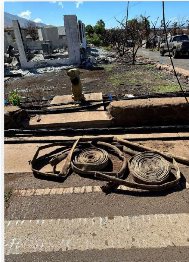
Fire hydrants, water meters, and water laterals will need to be replaced
