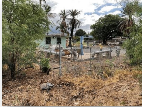
P.S. 4 – extensive wind and fire damage
