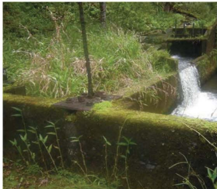
Figure 34: The sluice gate mechanism is a threaded shaft type that is inoperable due to corroded and missing parts. The gate once operated by turning a handwheel that advanced the formerly threaded vertical steel shaft up and down, moving the metal panel. The handwheel is missing and corrosion has destroyed the threads on the steel shaft. Some of these mechanisms have become inoperable due to lack of use. When necessary, however, they can be serviced to make the adjustments. This threaded shaft gate is located at EMI stream diversion at Kolea Power House, on Kolea, a tributary of Punalau, which is ordered to be restored as a "Habitat Stream " by CWRM . View facing S. (Source: MAI, 2018 .)
