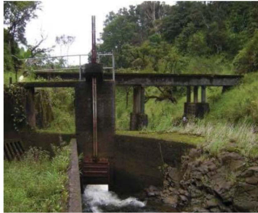
Figure 21: Typical sluice gate. Note the vertically sliding panel at the lower end that is operated by the mechanism above. This ratchet-operating gate is located at EMI stream diversion at Wailuaki East, which is ordered to be restored as a "Habitat Stream" by CWRM. (Source: MAI, 2018.)
