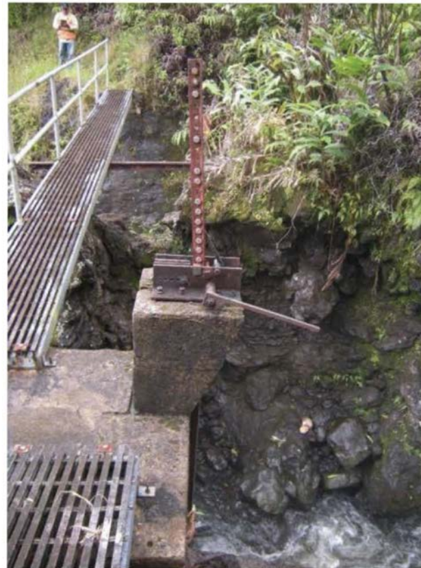
Figure 25: This sluice gate mechanism is a ratchet type. The concrete pedestal and platform it is mounted on is typical of ratchet type gate mechanisms. This ratchet-operating gate is located at EMI stream diversion at Makapiipi, which was fully restored in 2008. View facing SE. (Source: MAI, 2018.)
