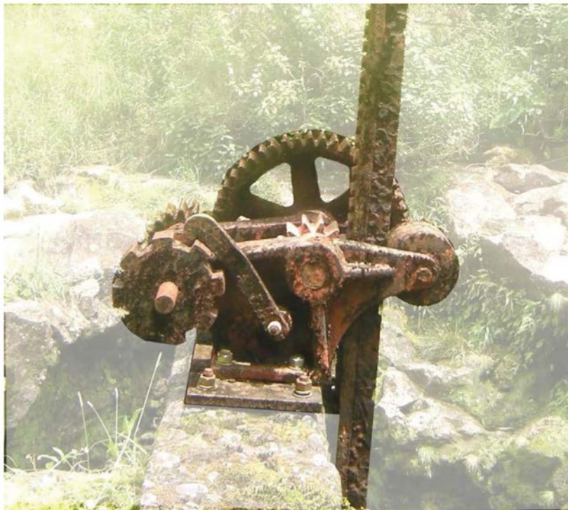
Figure 27: This typical geared type sluice gate operating mechanism is located at EMI Honomanu Stream diversion , which is ordered to be restored as a "Habitat Stream" by CWRM. View facing SE. (Source: MAI, 2018.)
