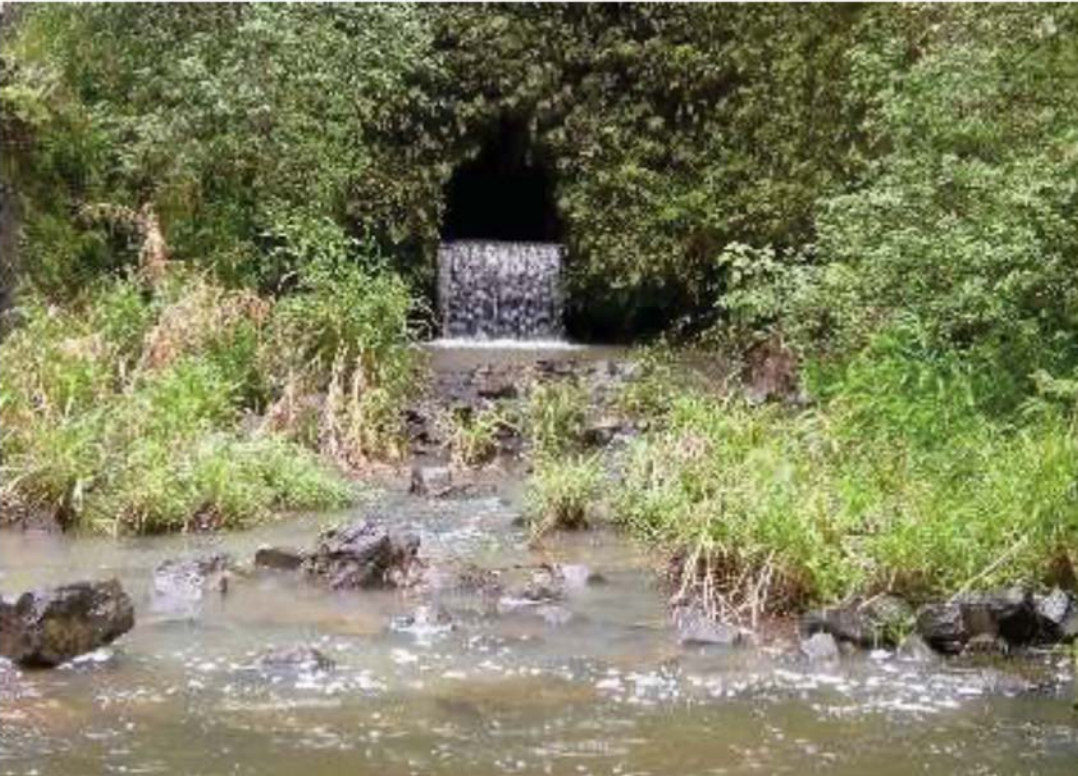
Figure 13: Tunnel near Kopiliula stream diversion carries water underground at ditch gradient. View facing SE. (Source: MAI, 2018.)
