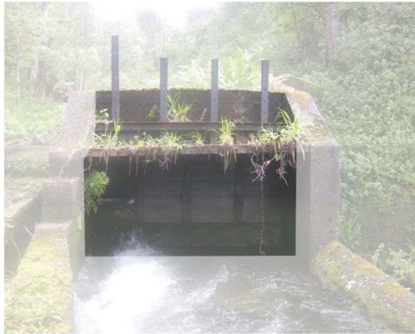
Figure 30: This typical board adjusted type sluice gate operating mechanism is located at EMI Kolea Power House stream diversion on Kolea, a tributary of Punalau, which is ordered to be restored as a "Habitat Stream" by CWRM. View facing SW. (Source: MAI, 2018.)
