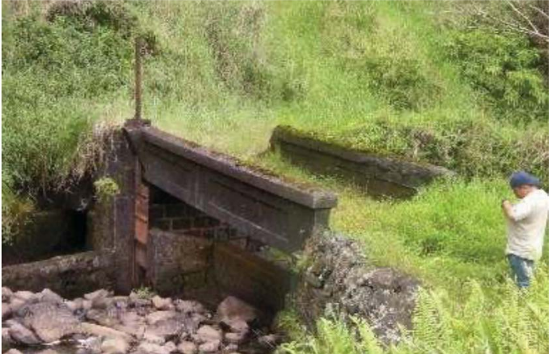
Figure 6: Bridge at Banana Intake stream diversion carries an access trail over the stream. (Source: MAI, 2018)
