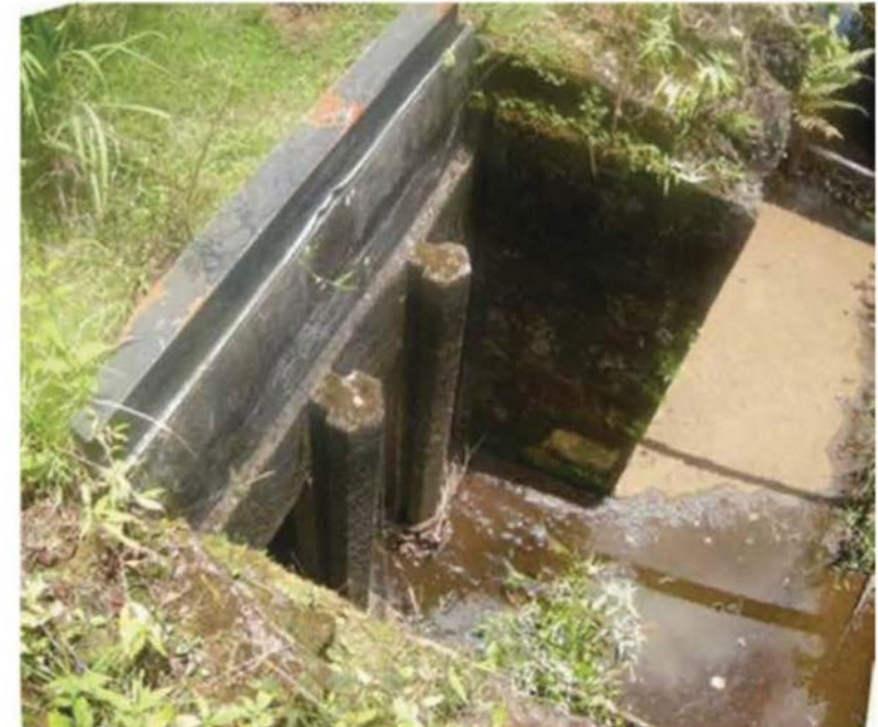
Figure 31: Board adjusted sluice gate with no boards installed. Note that this gate is about 5'wide in total, with three vertical spaces for boards . This board adjusted gate is located at EMI throw-out gate at Piinaau, which is ordered to be a "Fully Restored " stream by CWRM. View facing NE. (Source : MAI, 2018.)
