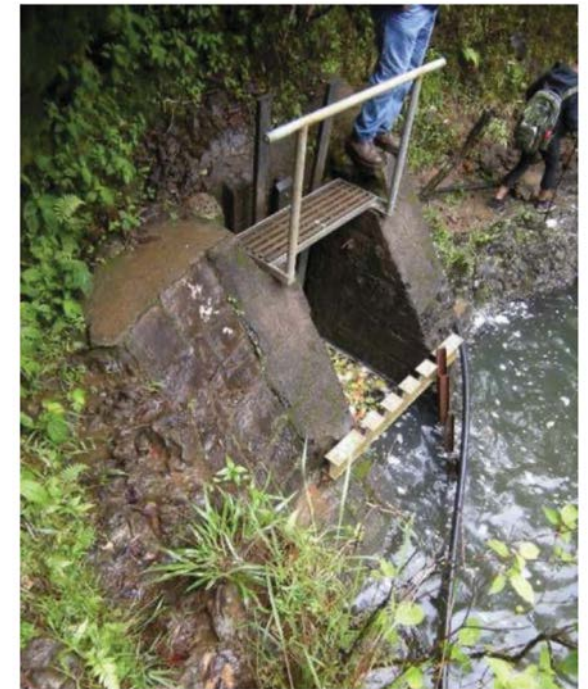
Figure 22: Typical configuration of sluice gates in a concrete dam. These sluice gates are located at EMI stream diversion at Kopiliula, which is ordered to be restored as a "Habitat Stream" by CWRM. View facing N. (Source: MAI, 2018.)
