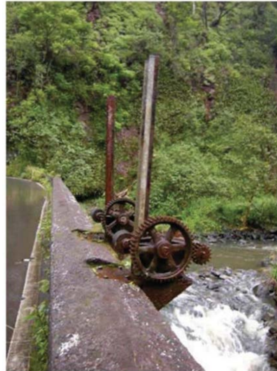
Figure 29: View of the same geared mechanism at right.
