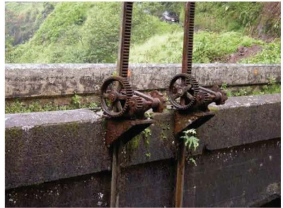
Figure 28: This sluice gate mechanism is a geared type. It operates by attaching a crank to the shaft of the small pinion gear. Revolving the crank operates the geared mechanism and advances the gear rack, to raise or lower the gates . This geared-operating gate is located at EMI stream diversion at Kopiliula, which is ordered to be restored as a "Habitat Stream" by CWRM. View facing E. (Source: MAI, 2018.)
