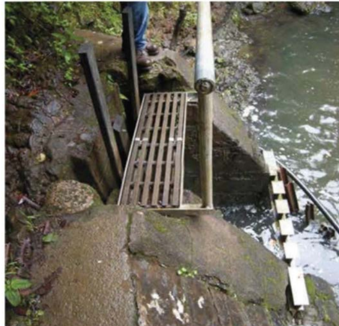
Figure 32: Board adjusted sluice gate with plastic boards installed . Boards are in the closed position , preventing water from passing through the gate. At about 2'-6" wide, this gate is typical width for board adjusted gates seen at EMI during the field survey. This board adjusted gate is located at EMI stream diversion at Waiohue , which is ordered to be a "Fully Restored" stream by CWRM . View facing SE. (Source: MAI, 2018.)
