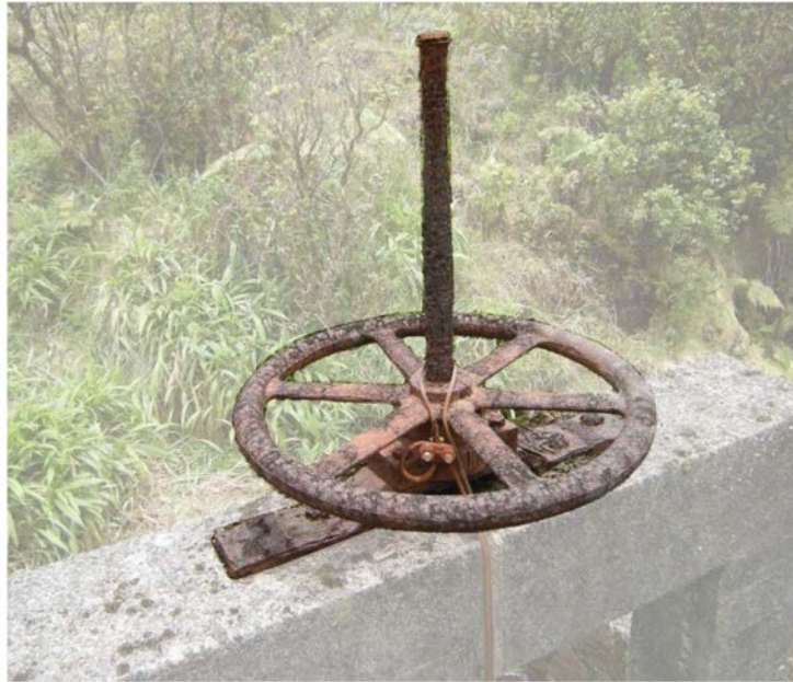
Figure 33: This threaded shaft type sluice gate operating mechanism is located along an irrigation ditch on the Big Island. It is very similar to the threaded shaft mechanism observed at EMI Kolea Power House stream diversion, on Kolea, a tributary of Punalau , which is ordered to be restored as a "Habitat Stream" by CWRM. The single example surveyed was too damaged to properly illustrate its configuration. (Photo: MAI, 2017.)
