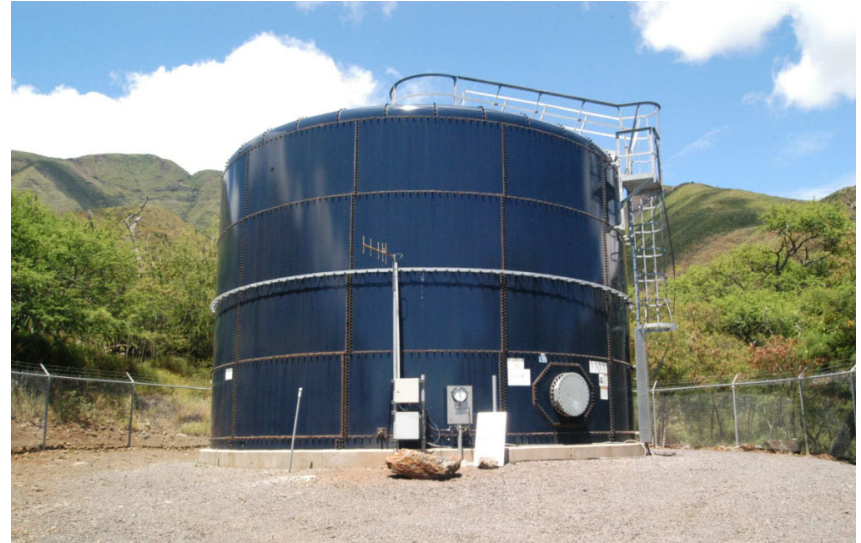
LWC Tank 2 50,000 gallons
