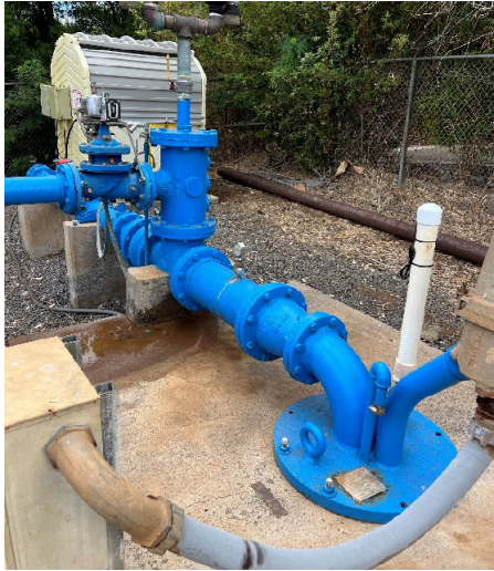
LWC Well 1 State Well no. 6-5138-01 Capacity: 500 GPM / 125 HP
