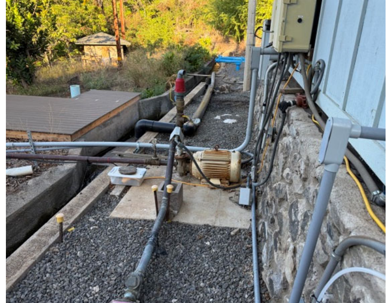
NP Booster Pump 120 GPM / 25 HP
