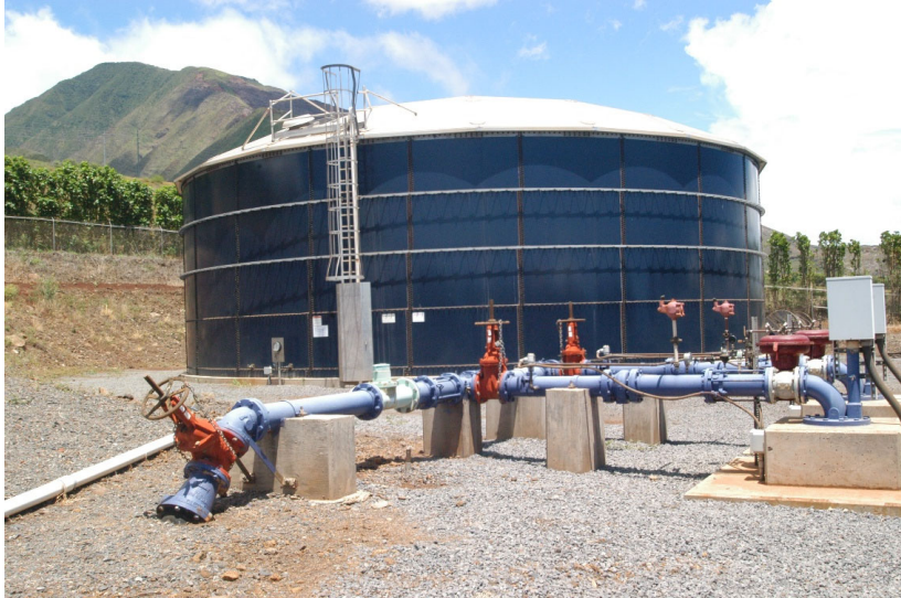
LWC Tank 1 400,000 gallons with 2 Booster Pumps
