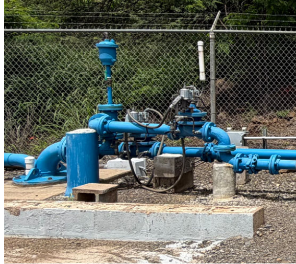
LWC Well 2 State no. 6-5137-01 Capacity: 100 GPM / 40 HP
