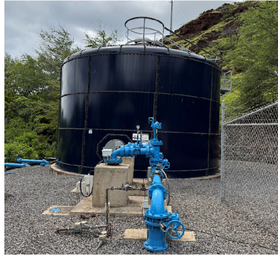
OWC Tank 1 50,000 gallons Booster Pumps Two - 250 GPM / 20 HP
