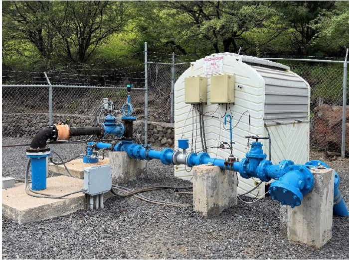
OWC Well 1 State Well no. 6-4936-001 Capacity: 250 GPM / 25 HP Average Daily Pumping: 78,217 GPD (CWRM GWUPA)
