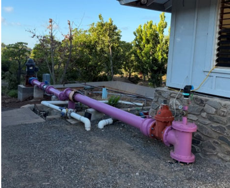
Mid-Level Booster Pump 500 GPM / 40 HP
