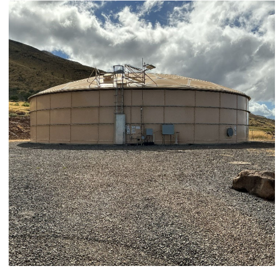
OWC Tank 2 500,000 gallons
