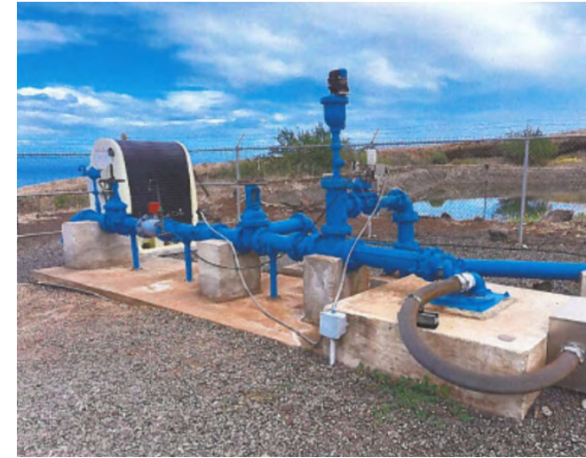
LWC Well 3 State Well no. 6-5238-01 Capacity: 500 GPM / 150 HP
