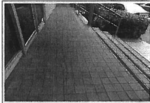
NOTE CRACKED AND LIFTED TILES
