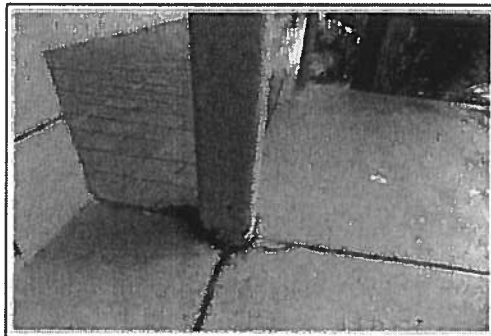
RUSTED SUPPORT POST
