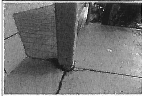
RUSTED SUPPORT POST
