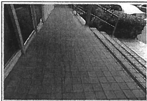
NOTE CRACKED AND LIFTED TILES
