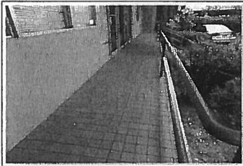
EVIDENCE OF SPALLING ON PORCH
