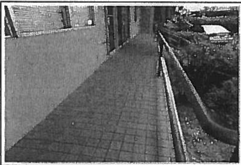
EVIDENCE OF SPALLING ON PORCH
