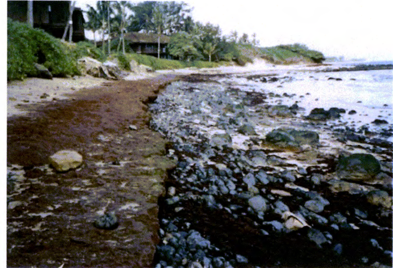
June 1989: beach is gone eroded clay, rocks, and sand bags
