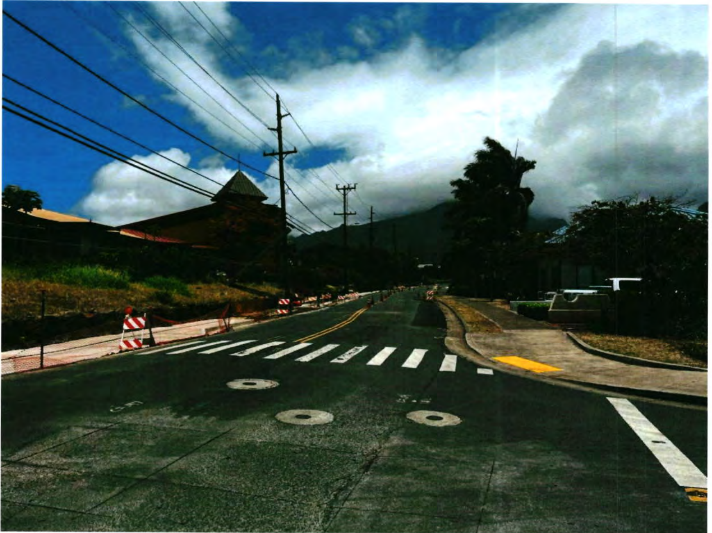
5 5-Mill Street Date Taken: 7/14/2022 Taken By: Kevin Frost Mill street incline -sewer repairs at bottom of incline
