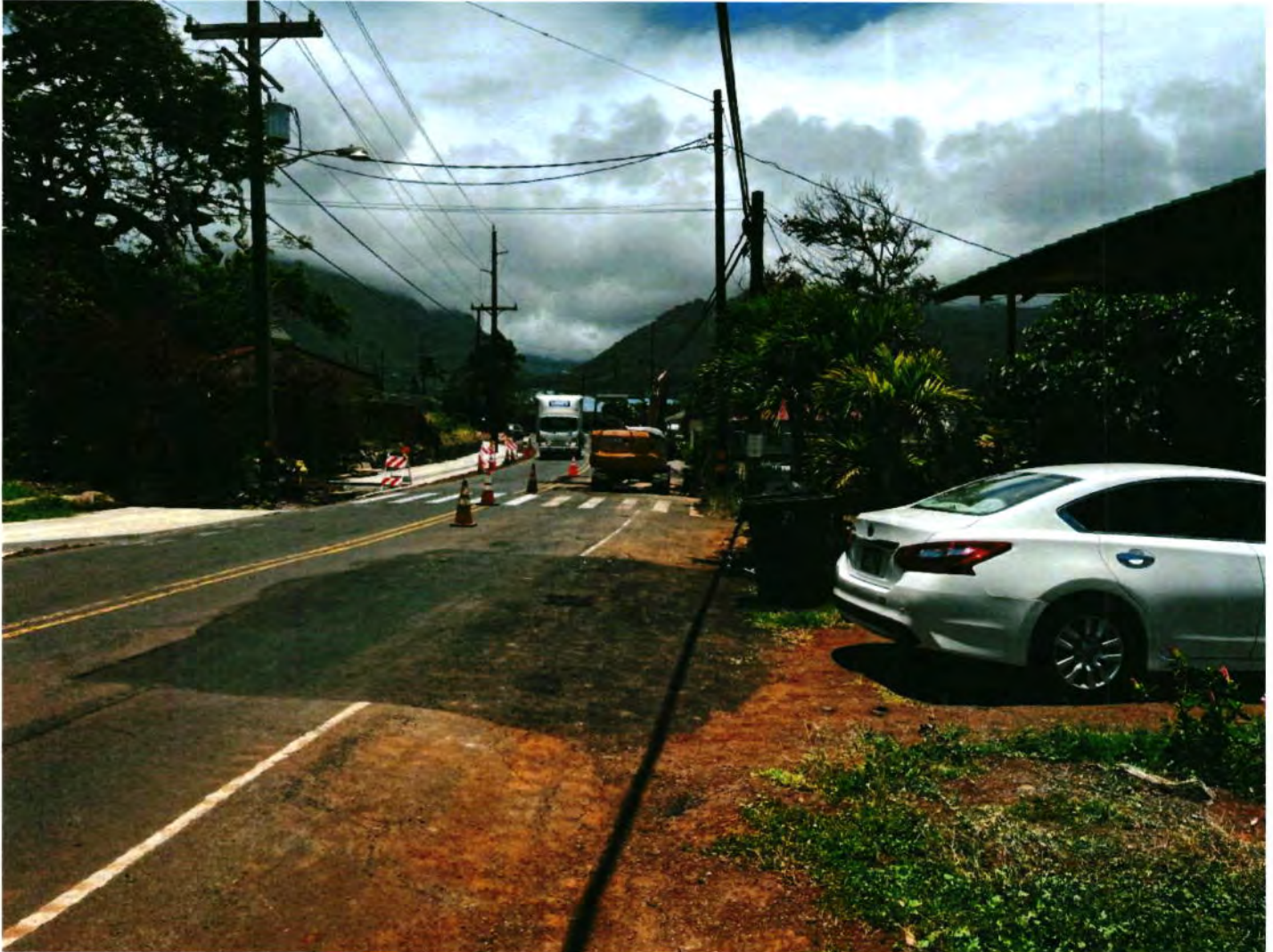
7 7-Loss Location Date Taken: 7/14/2022 Sewer repairs completed immediately in front of loss location
