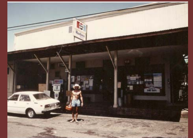
During the rehabilitation of Mā'alaea General Store, the missing parapet wall was reconstructed using historic photos. (photo source unknown)
