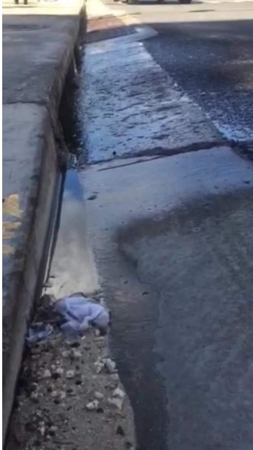
Storm drain backflow
