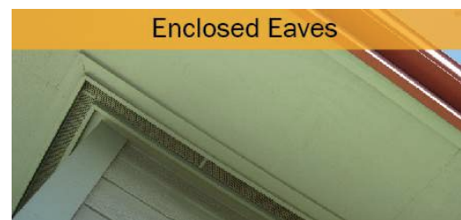
Figure 8. Make sure your eaves are enclosed with non-combustible materials to prevent ember entry.
