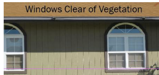
Figure 7. Keep windows free of vegetation to reduce likelihood of heat-caused breakage that lets embers into your home.
