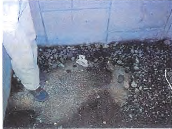
Sediment and Gravel in Culverts
