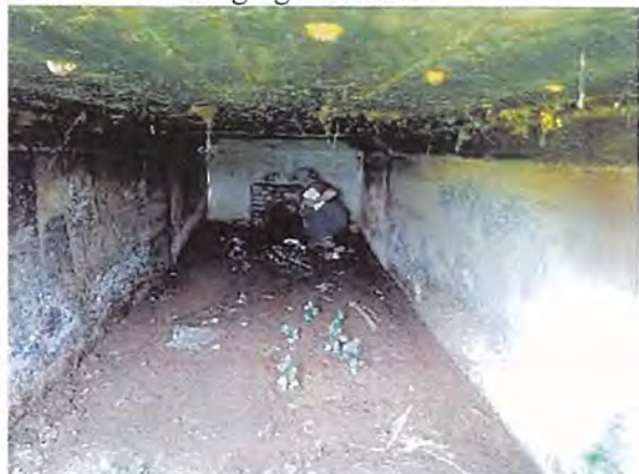
Substantial Sediment Deposition in Culvert
