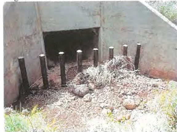
Sediment and Gravel at Culvert Entrance
