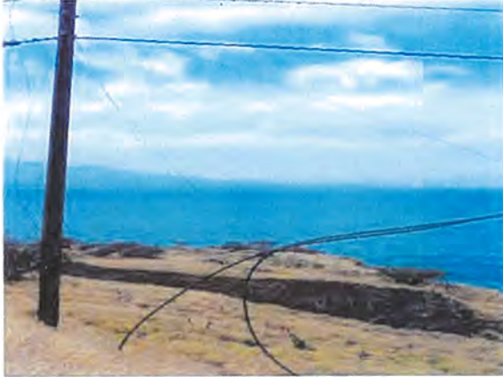
Downed Communications Lines
