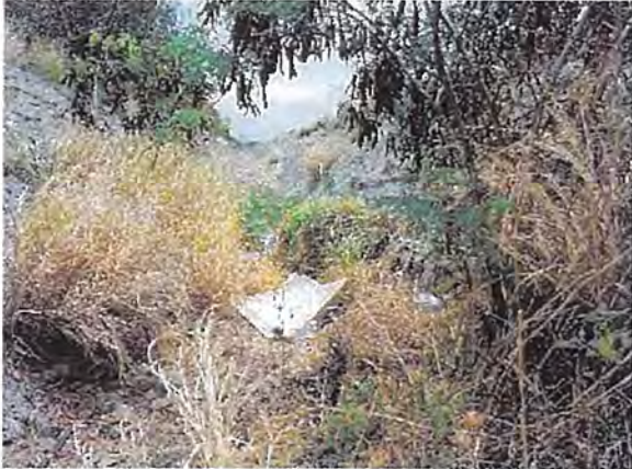
Vegetation and Rubbish in Ditch
