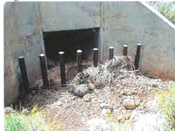
Sediment and Gravel at Culvert Entrance
