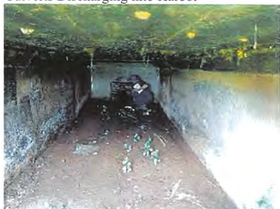
Substantial Sediment Deposition in Culvert
