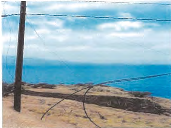
Downed Communications Lines
