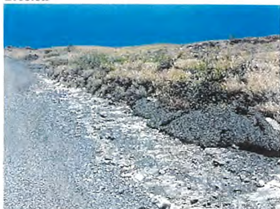
Gravel Loss in Swale
