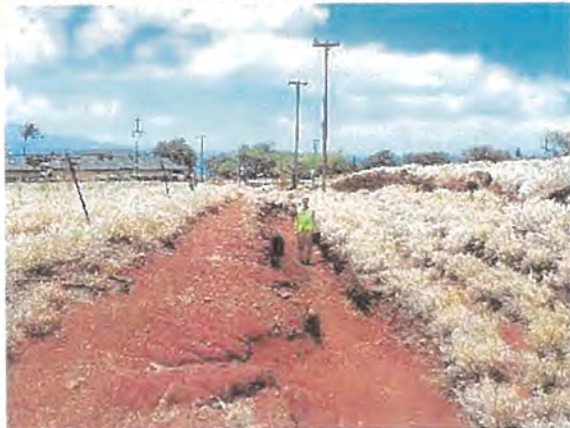
Distribution Lines and Failed Roads
