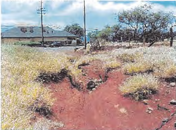
Failed Road with Channelization and Erosion
