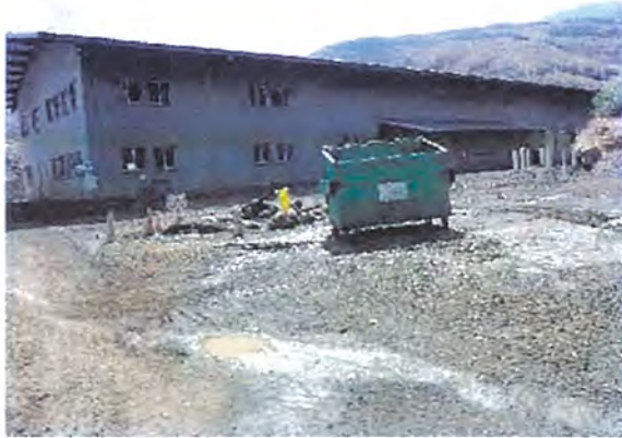
Gravel Roads with Mud and Erosion
