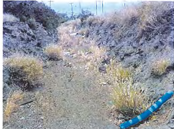
Rubbish in Ditch
