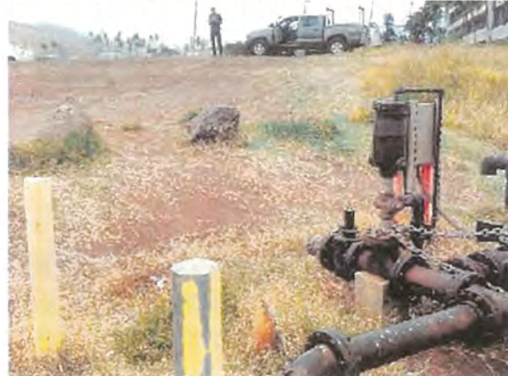
Dirt Lots with No BMPs in Place
