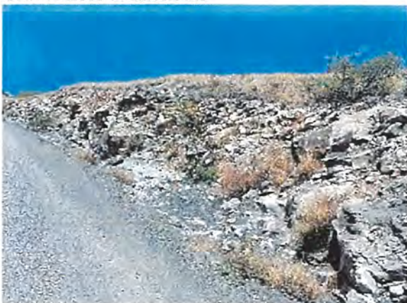
Channelization and Gravel Loss in Swale
