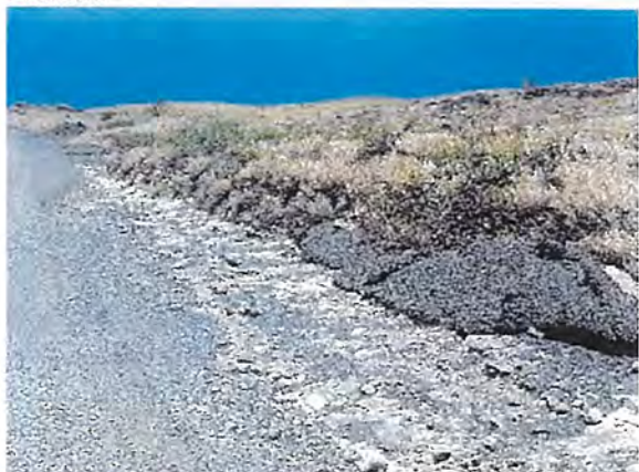
Gravel Loss in Swale
