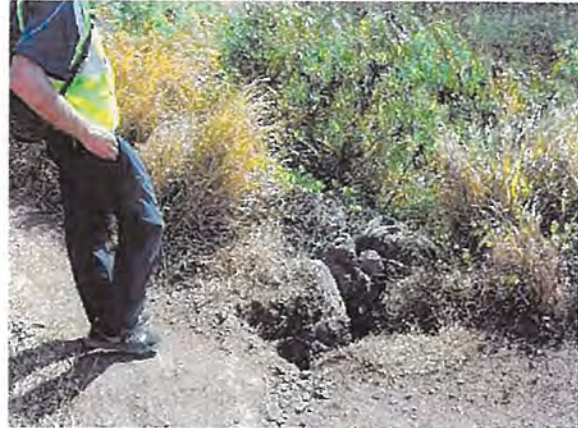
Erosion and Discharge from Road
