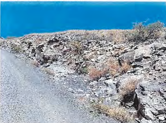
Channelization and Gravel Loss in Swale
