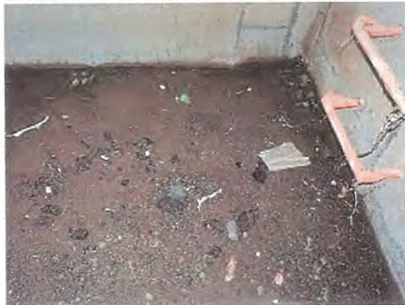
Sediment and Gravel in Culverts
