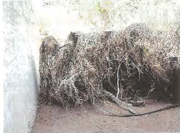
Vegetation at Entrance to Culvert
