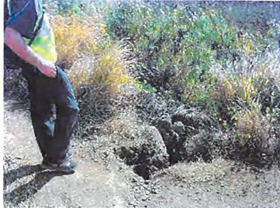
Erosion and Discharge from Road
