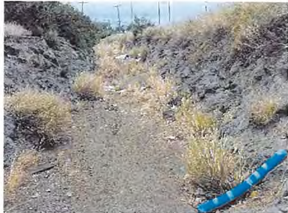
Rubbish in Ditch
