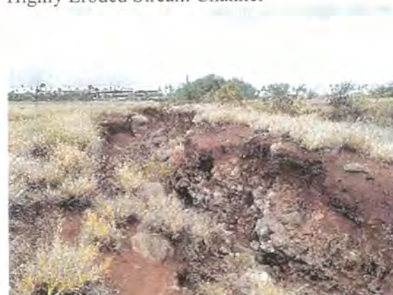
Highly Eroded Stream Channel
