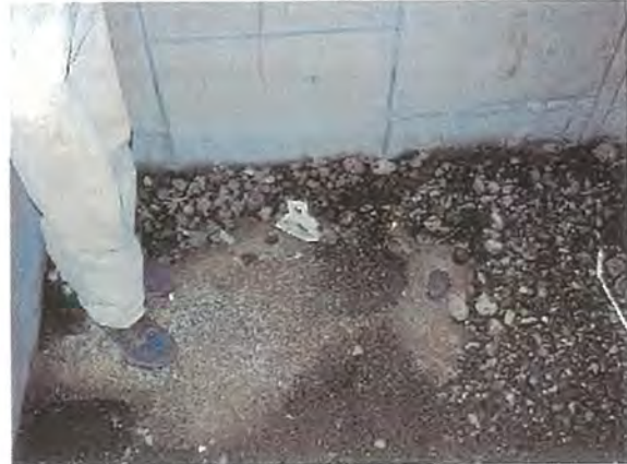
Sediment and Gravel in Culverts
