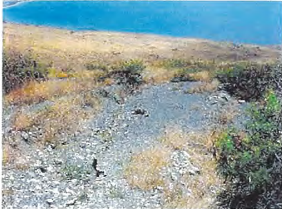
Gravel Loss at Kickouts
