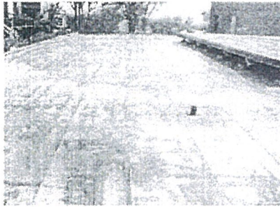
Picture at left Roof material at the end of life expectancy and opening to atrium on second floor – Roof life can be extended by applying a waterproof roof sealant and new atrium roof designed into renovation
