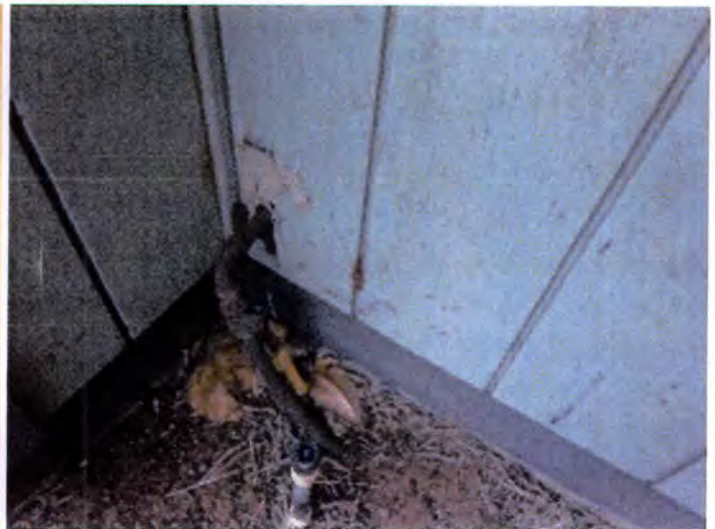
Copper supply plumbing
