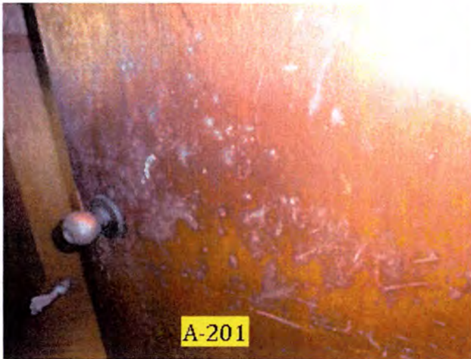
Visible mold observed at interior doors.
