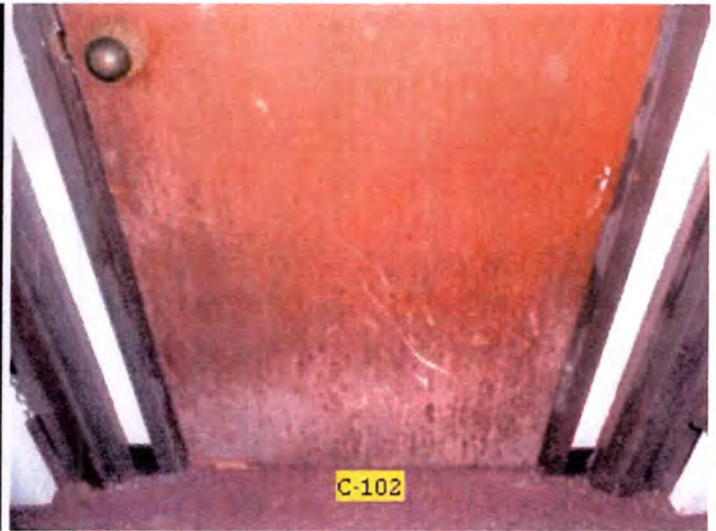
Visible mold observed at interior doors.
