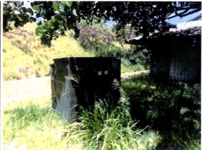
Transformers were located: rear center of property.
