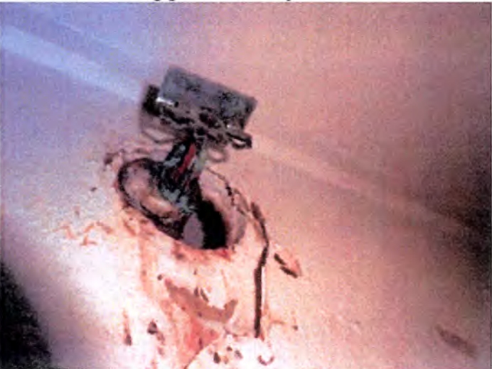
C-101: Sprinkler head was leaking when inspected.
