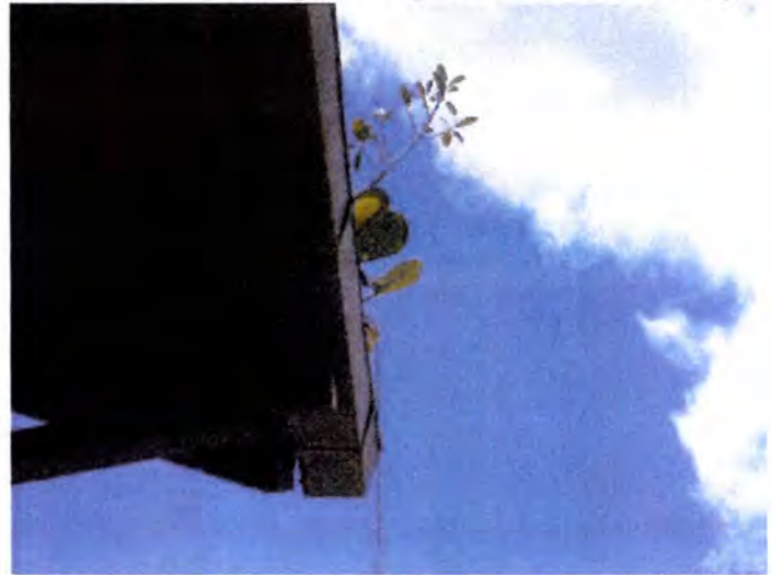
Vegetation growth observed in gutters. Recommend clearing.
