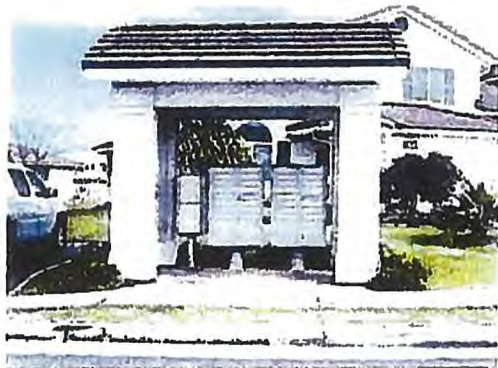
Centralized equipment installed by Developer
