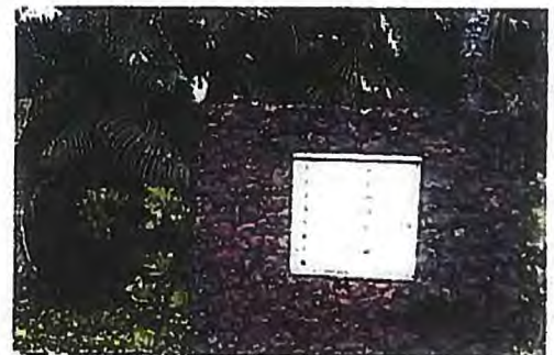
Custom Box installed by Developer
