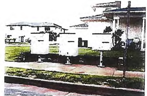
Centralized equipment installed by Developer
