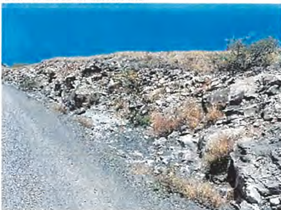
Channelization and Gravel Loss in Swale
