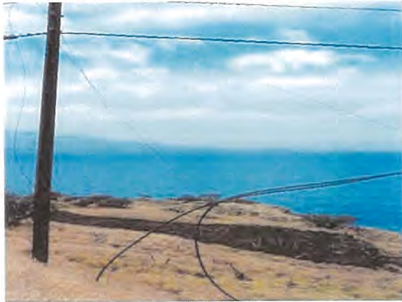
Downed Communications Lines
