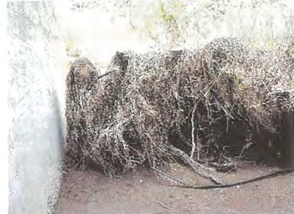
Vegetation at Entrance to Culvert
