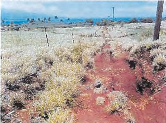
Failed Road with Channelization and Erosion
