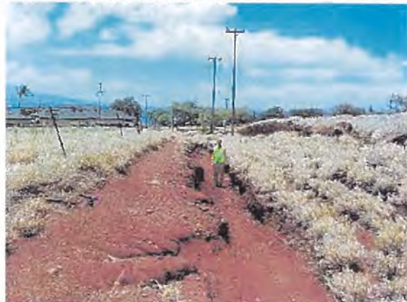
Failed Road with Channelization and Erosion
