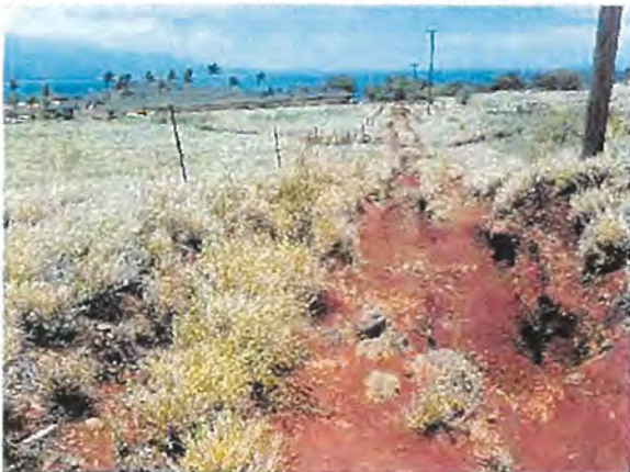
Failed Road with Channelization and Erosion
