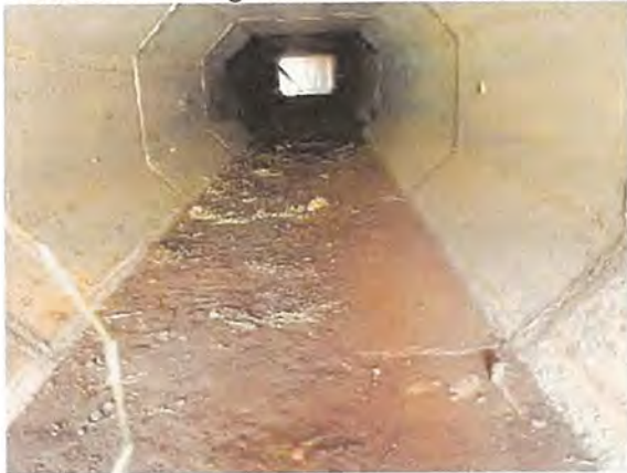
Sediment in Culverts
