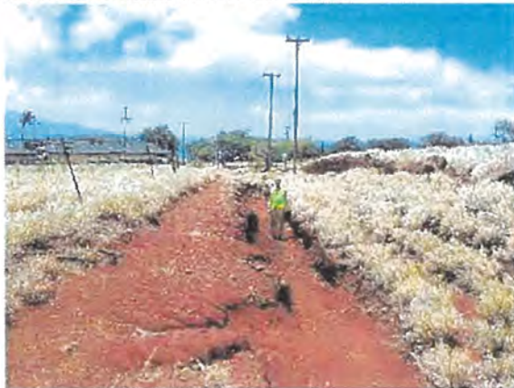
Distribution Lines and Failed Roads
