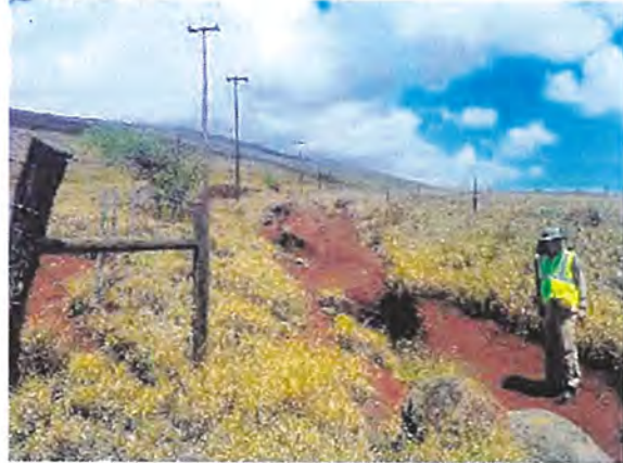
Channelization and Erosion
