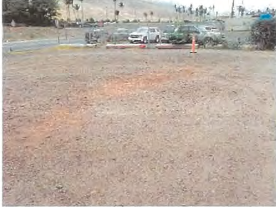
Dirt Lots with No BMPs in Place
