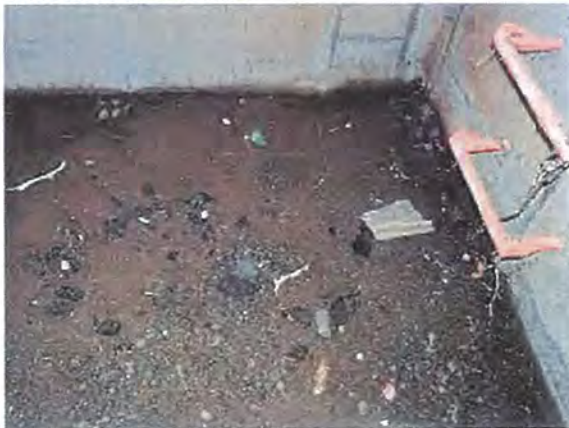
Sediment and Gravel in Culverts
