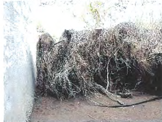
Vegetation at Entrance to Culvert
