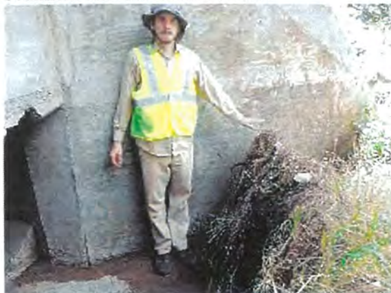
Extent of Vegetation at Entrance to Culvert
