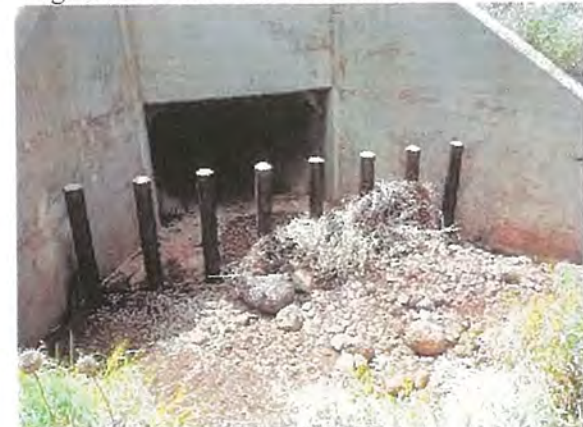
Sediment and Gravel at Culvert Entrance
