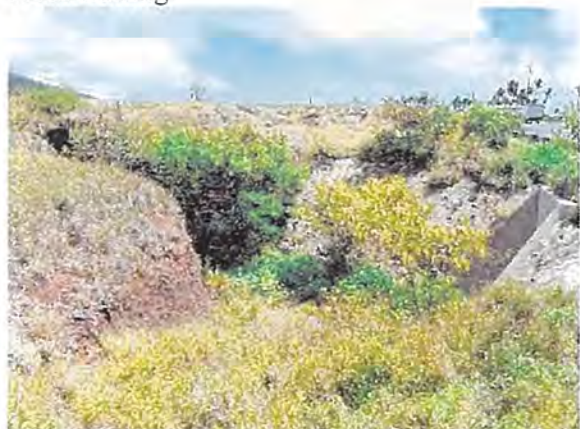
Culvert Backwall and Head Cutting
