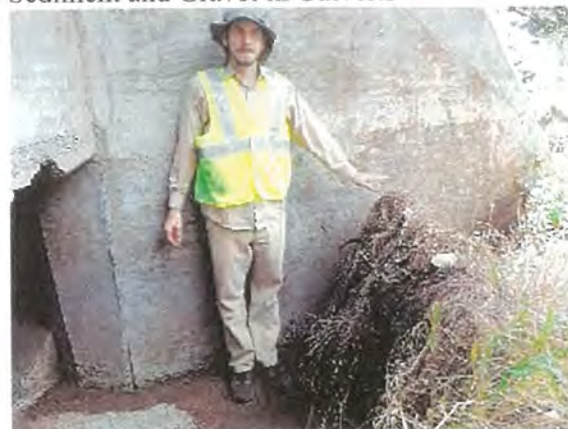
Extent of Vegetation at Entrance to Culvert
