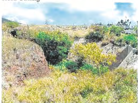
Culvert Backwall and Head Cutting
