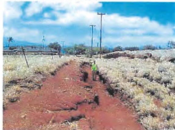
Failed Road with Channelization and Erosion
