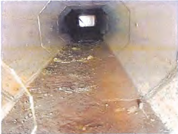
Sediment in Culverts
