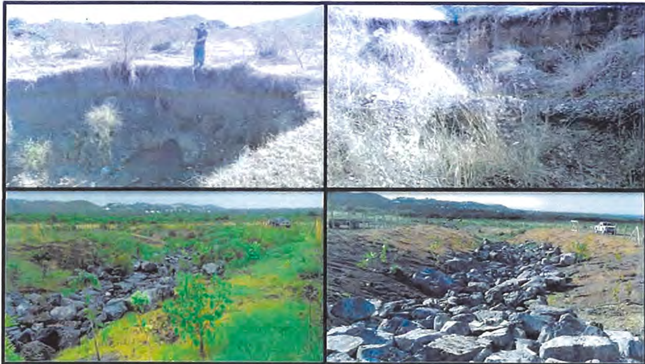
Figure 22. Examples of Head Cutting and Stabilization
