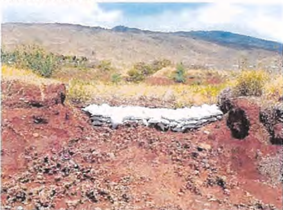
Failed Control Structure
