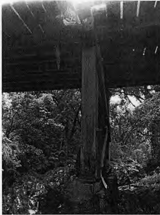
PHOTO 9 SEVERE DECAY AT UPSTREAM END OF TIMBER PIER CAP BEAM
