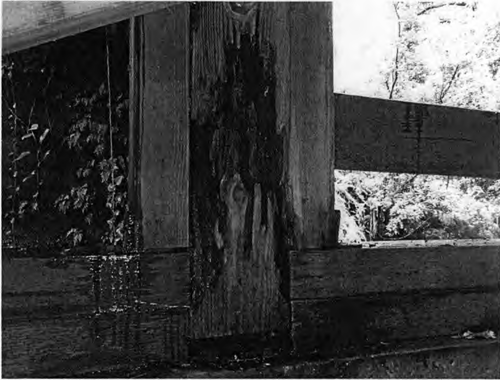
PHOTO 11 DECAYED TIMBER COLUMN AND BEARING PLATE AT BASE OF CENTER TIMBER PIER COLUMN
