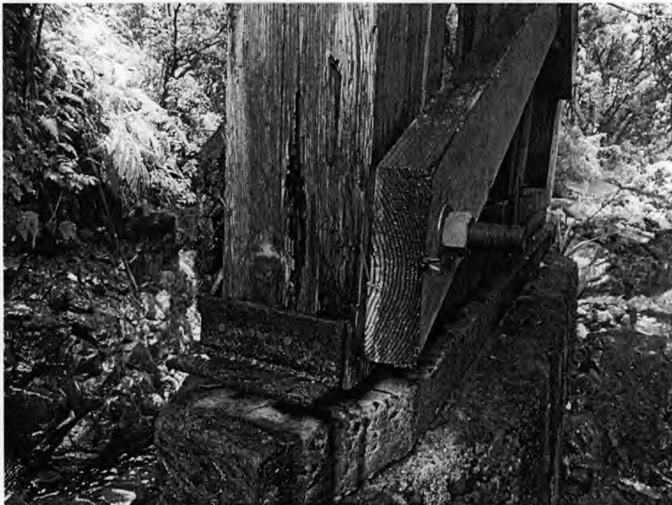
PHOTO 10 DECAYED UPSTREAM TIMBER PIER COLUMN
