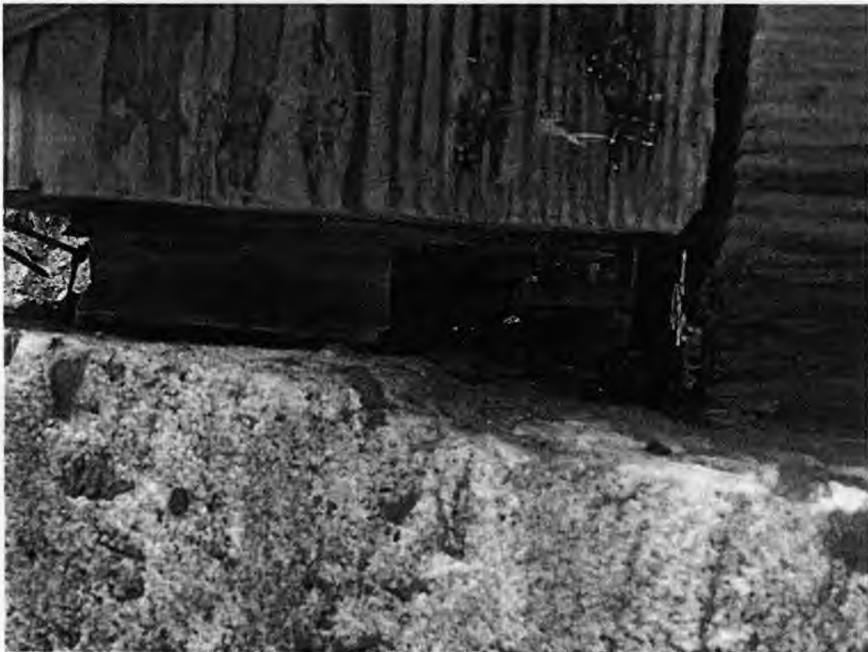
PHOTO 12 DECAYED TIMBER BEARING PLATE AT BASE OF UPSTREAM TIMBER PIER COLUMN
