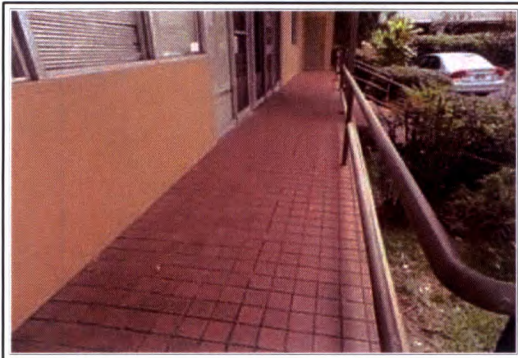
EVIDENCE OF SPALLING ON PORCH
