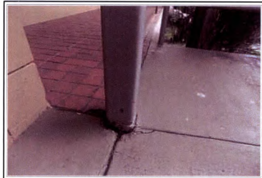
RUSTED SUPPORT POST
