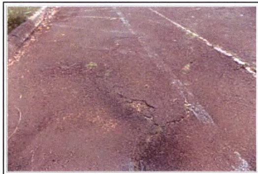
WORN PARKING AREA
