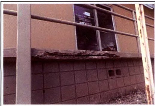
EVIDENCE OF SPALLING
