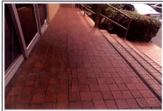
EVIDENCE OF SPALLING ON PORCH
