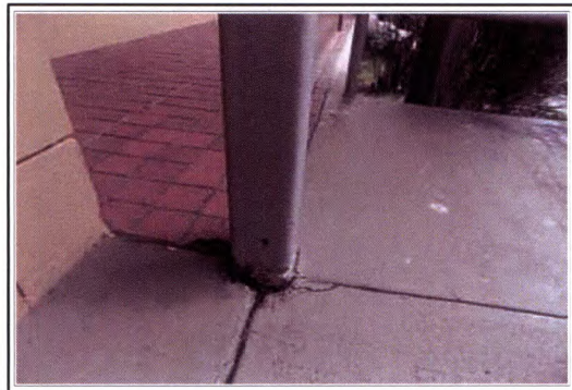
RUSTED SUPPORT POST
