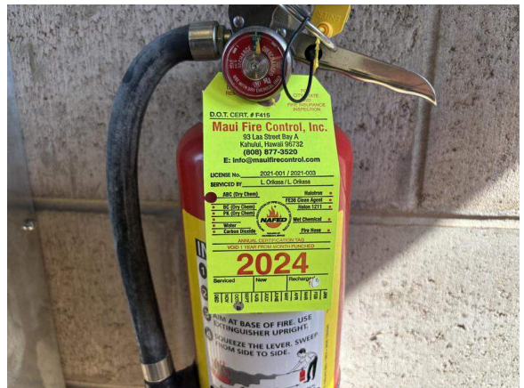
40 Typical fire extinguisher
