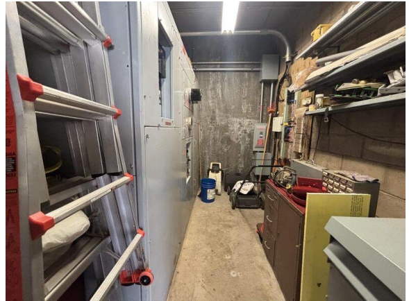
38 Main electrical room
