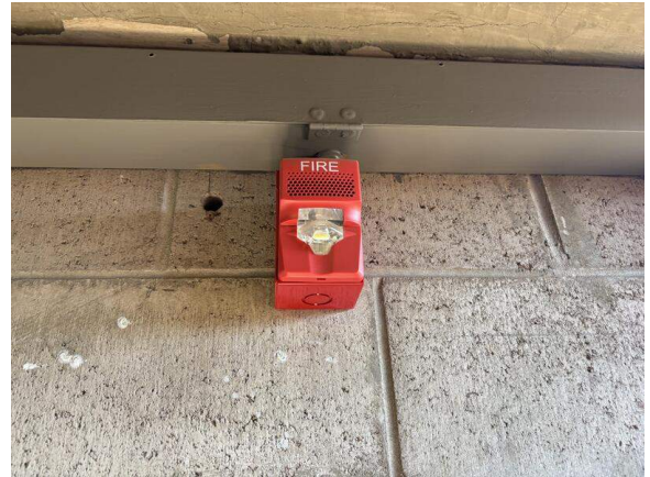
44 Fire alarm device
