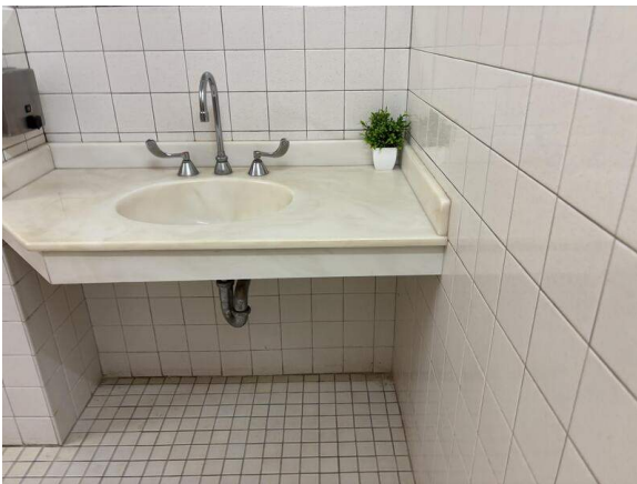
27 Typical sink at restrooms on each floor
