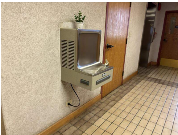
23 Typical drinking fountain on each floor
