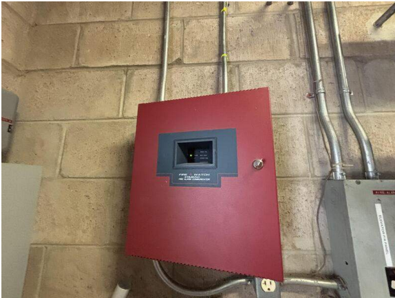
43 Main Fire alarm panel
