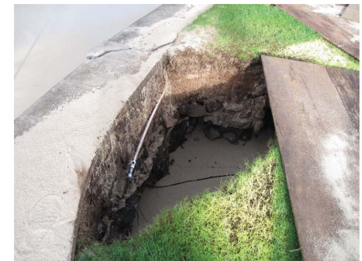
Photo 30: Typical sink hole behind seawall (1/10/2011).
