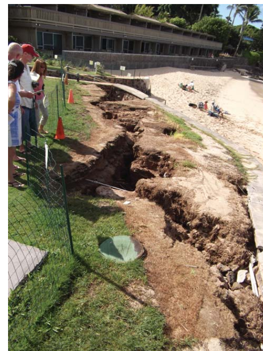
Photo 29: Sink holes behind seawall (10/10/2011).
