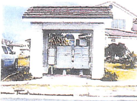
Centralized equipment installed by Developer
