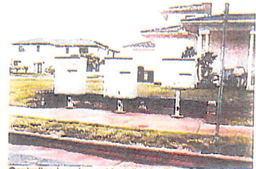
Centralized equipment installed by Developer
