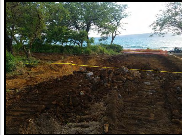
(2) 2-1-005:108 (ATC Makena) Graded an easement on ATC parcel without an SMA permit.
