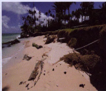
Beach and Land Erosion Causing Pollution at Project Beach, 4 August 2009 - before geotube groins
