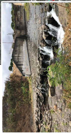
Existing head cut at upstream lined channel; proposed location of pre-formed scour hole
