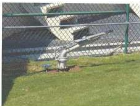
3. Aboveground irrigation gun used for athletic field irrigation
