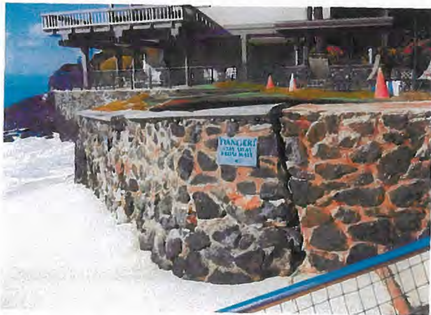
Figure 3. The wall seen in the photo above is shown with the recent damage caused by sinkholes in this February 2012 photo by Engledow. Signs, fencing and plywood covering sinkholes keep people out of the area.
