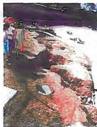
Photo 29: Sink holes behind seawall (10/10/2011).
