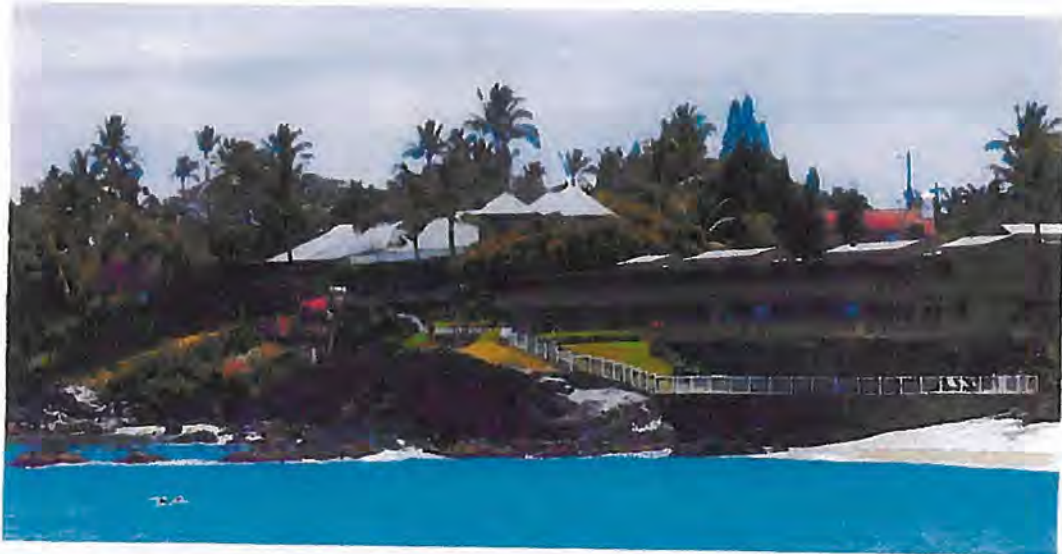
Fig. 2. Kahana Sunset condominium. This photo was taken by Engledow in April 2009. The area now in need of repair is the stone seawall at the right of the photo, topped with a white fence.
