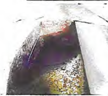
Photo 30: Typical sink hole behind seawall (1/10/2011).
