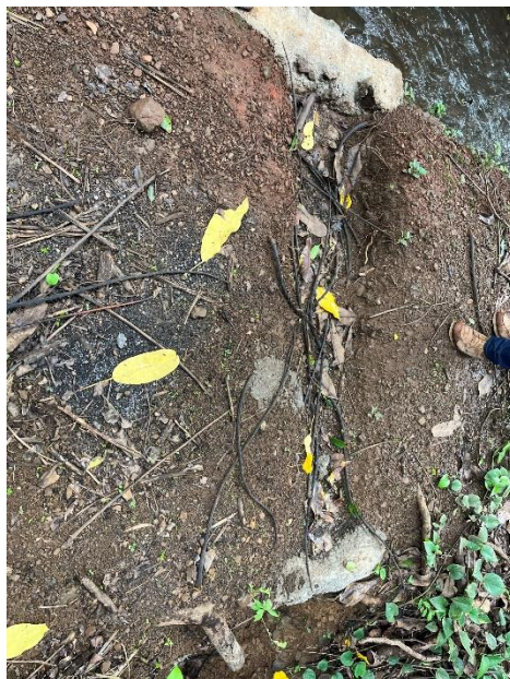
F) Damage indicated along Lowrie Ditch before siphon across East Kuiaha Gulch
