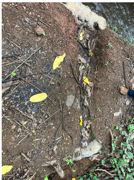
F) Damage indicated along Lowrie Ditch before siphon across East Kuiaha Gulch
