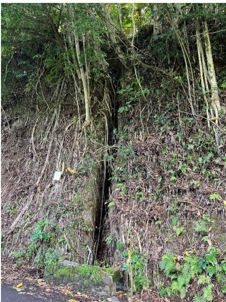
E) Vertical channel cut into the hillside along Ha'ikū Rd on the east side of East Kuiaha Stream Bridge
