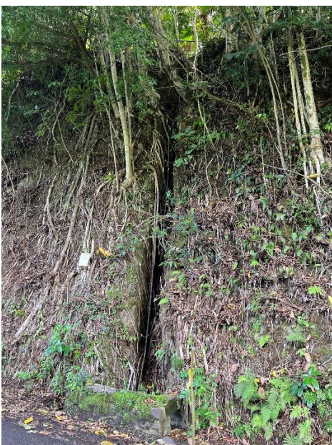
E) Vertical channel cut into the hillside along Ha'ikū Rd on the east side of East Kuiaha Stream Bridge
