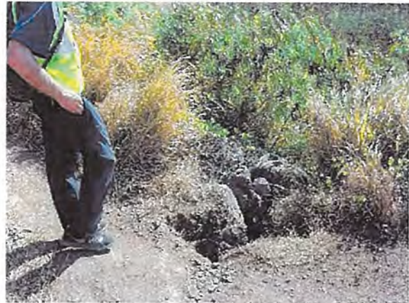
Erosion and Discharge from Road
