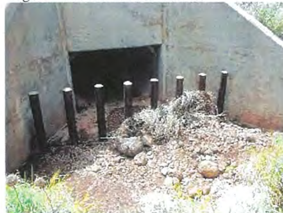
Sediment and Gravel at Culvert Entrance
