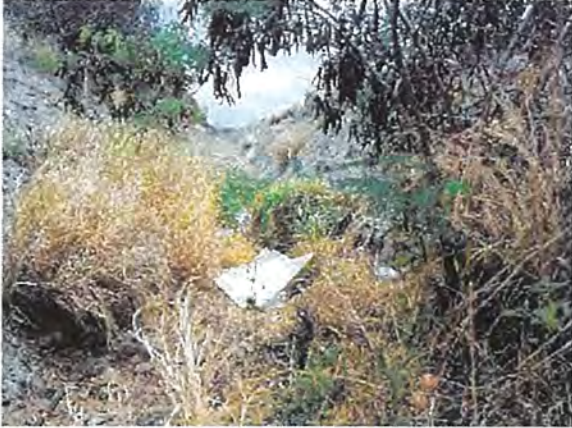
Vegetation and Rubbish in Ditch
