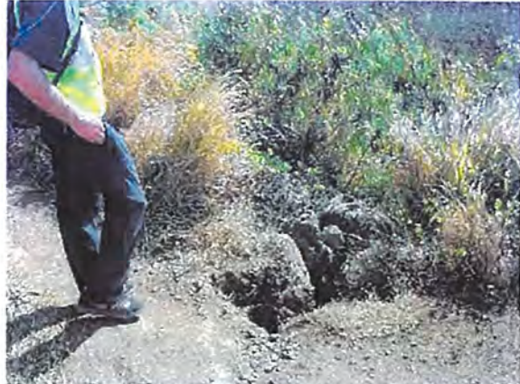
Erosion and Discharge from Road
