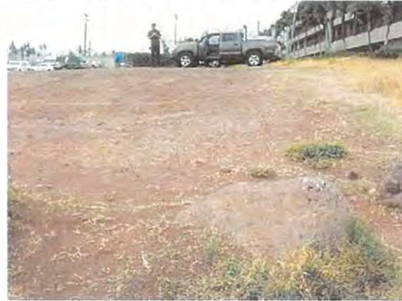
Dirt Lots with No BMPs in Place
