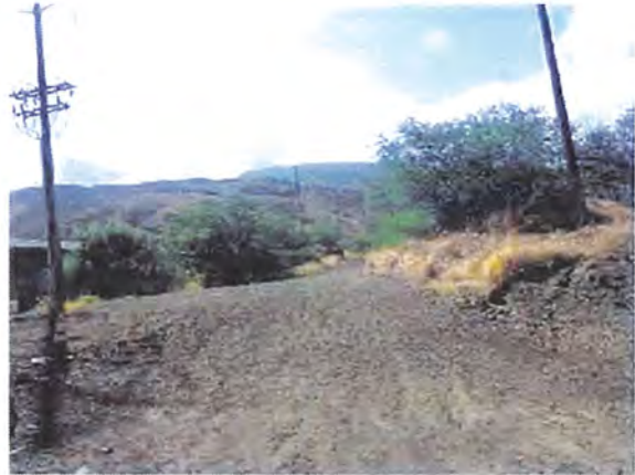
Gravel Roads Near Ditches
