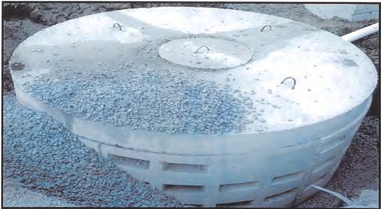
Figure 28. Stormwater Infiltration Well
