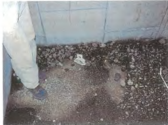
Sediment and Gravel in Culverts
