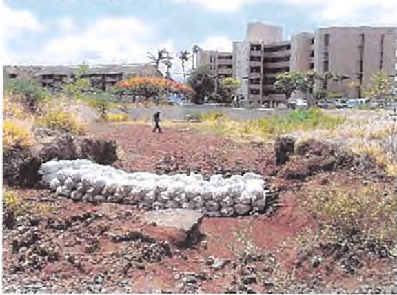
Sand Bags at Failed Control Structure
