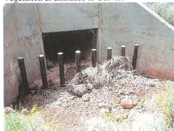
Sediment and Gravel at Culvert Entrance
