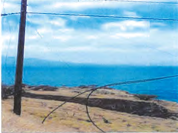
Downed Communications Lines
