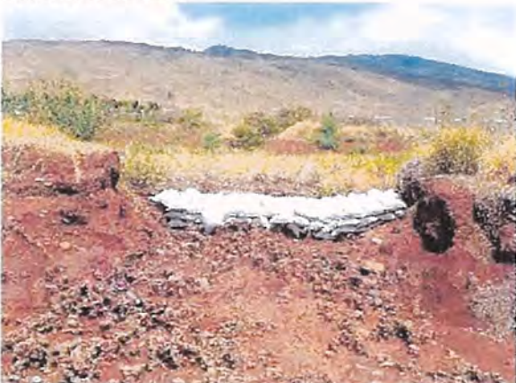
Failed Control Structure
