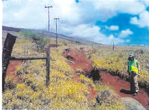
Channelization and Erosion
