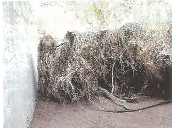
Vegetation at Entrance to Culvert
