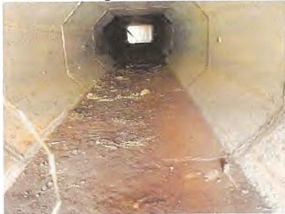
Sediment in Culverts
