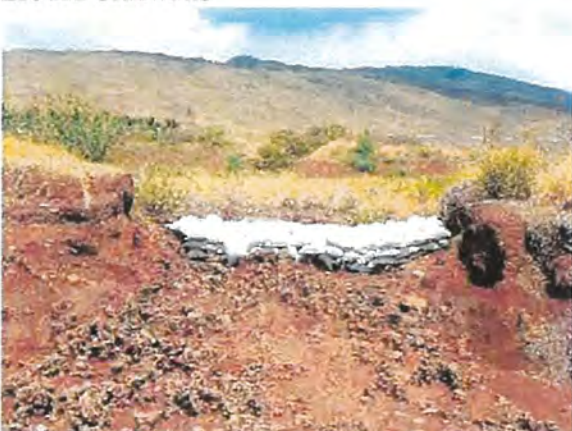
Failed Control Structure
