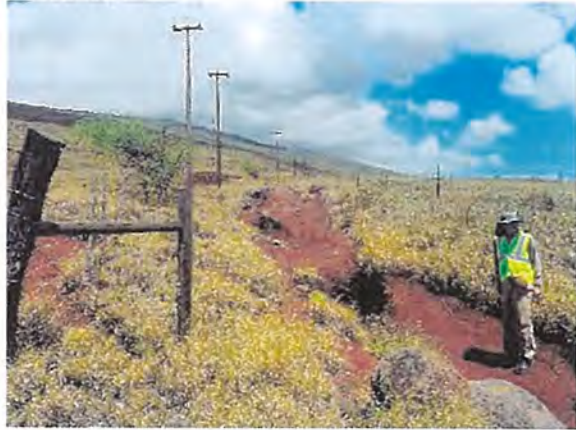
Channelization and Erosion
