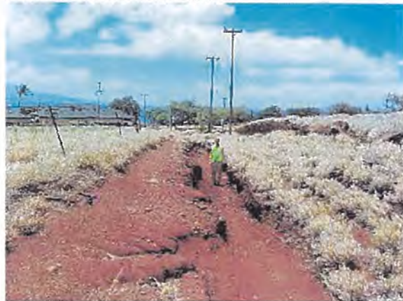
Failed Road with Channelization and Erosion
