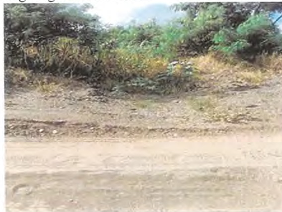
Road Crossing Pohakea Lacking BMPs
