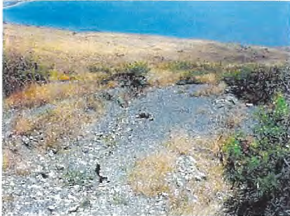
Gravel Loss at Kickouts
