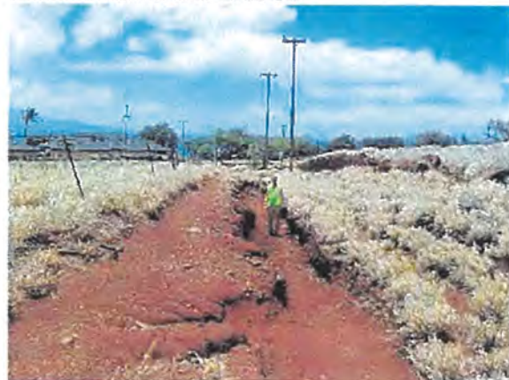
Failed Road with Channelization and Erosion
