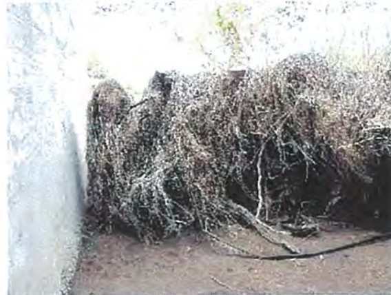
Vegetation at Entrance to Culvert
