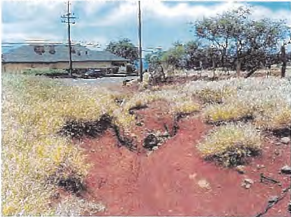
Failed Road with Channelization and Erosion
