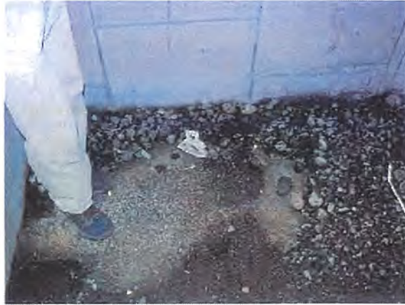
Sediment and Gravel in Culverts
