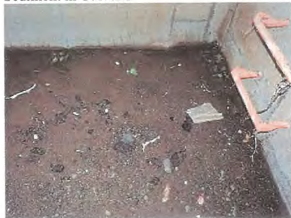
Sediment and Gravel in Culverts
