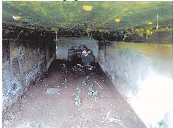
Substantial Sediment Deposition in Culvert
