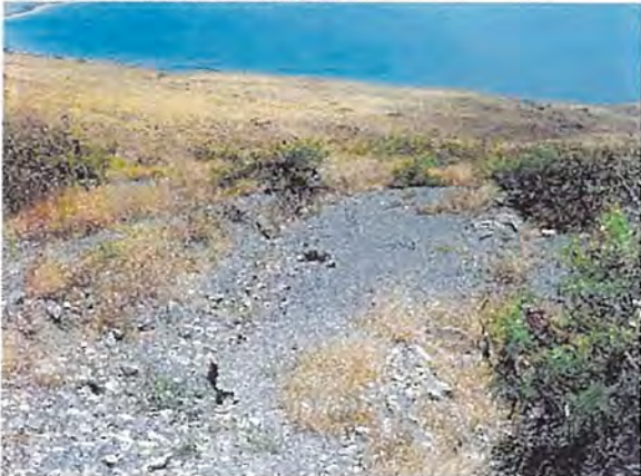
Gravel Loss at Kickouts
