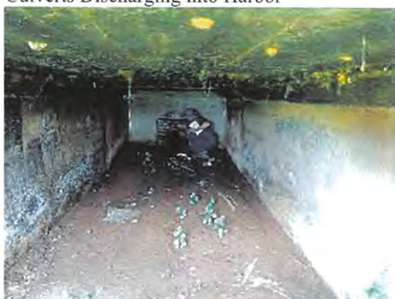
Substantial Sediment Deposition in Culvert
