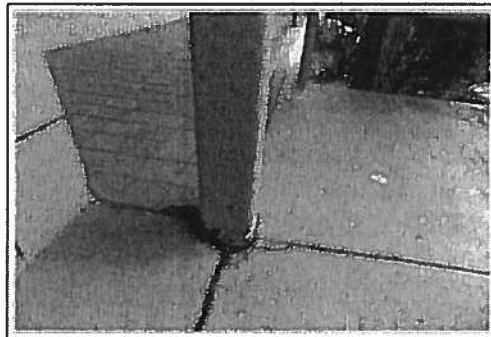
RUSTED SUPPORT POST
