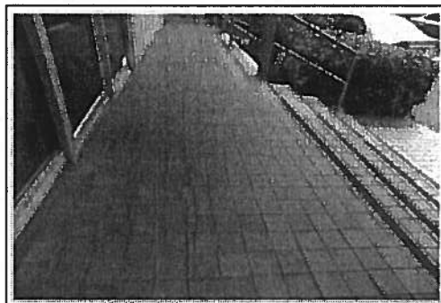
NOTE CRACKED AND LIFTED TILES
