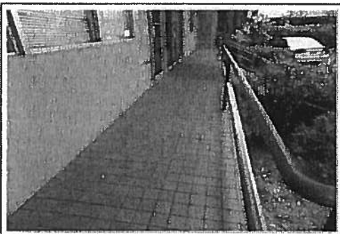
EVIDENCE OF SPALLING ON PORCH
