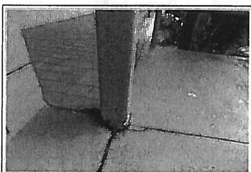
RUSTED SUPPORT POST
