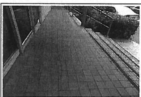
NOTE CRACKED AND LIFTED TILES
