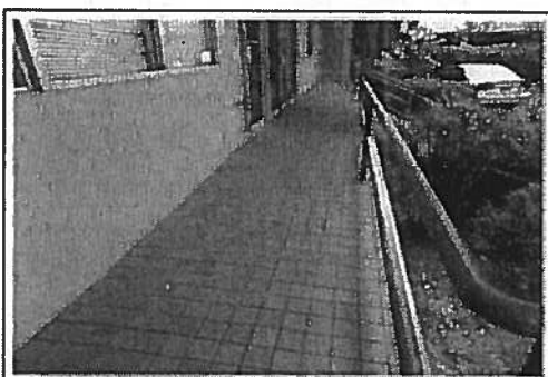
EVIDENCE OF SPALLING ON PORCH
