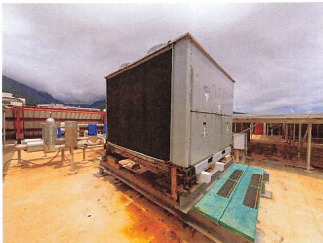
AC Chiller Requiring Replacement
