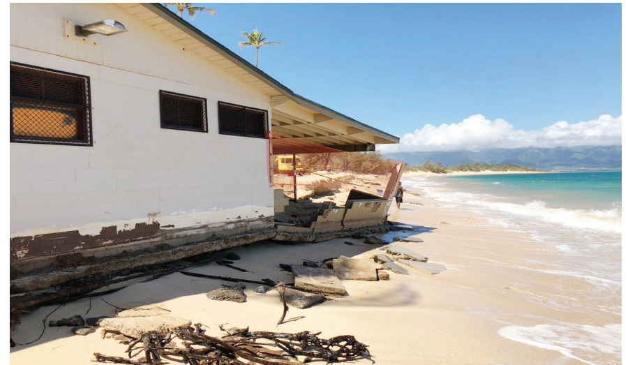
The makai side of the pavilion was undermined by high waves in September 2019, an action that will likely be more common in the future.
