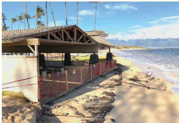
The pavilion was severely damaged in 2019, requiring that a portion of the structure be removed.
