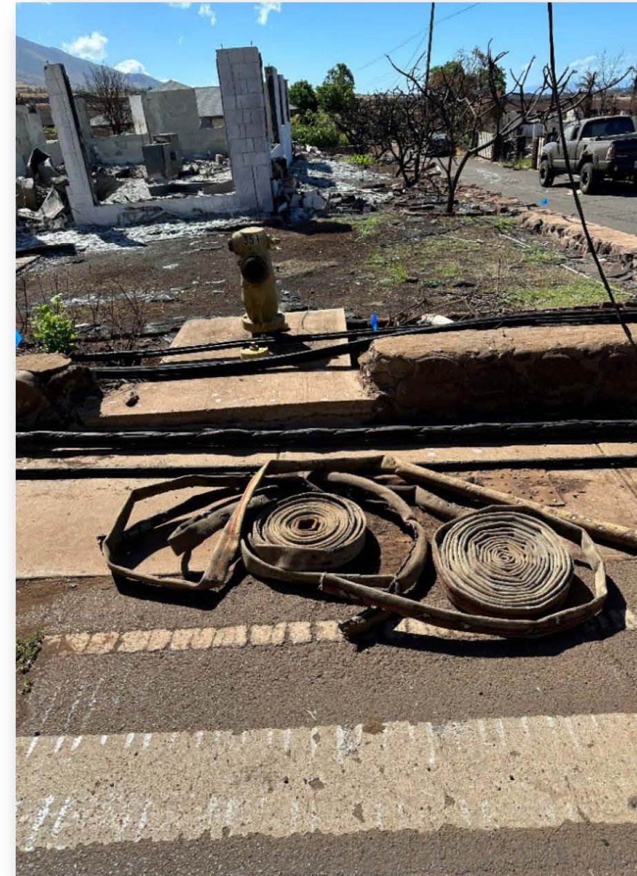
Fire hydrants, water meters, and water laterals will need to be replaced
