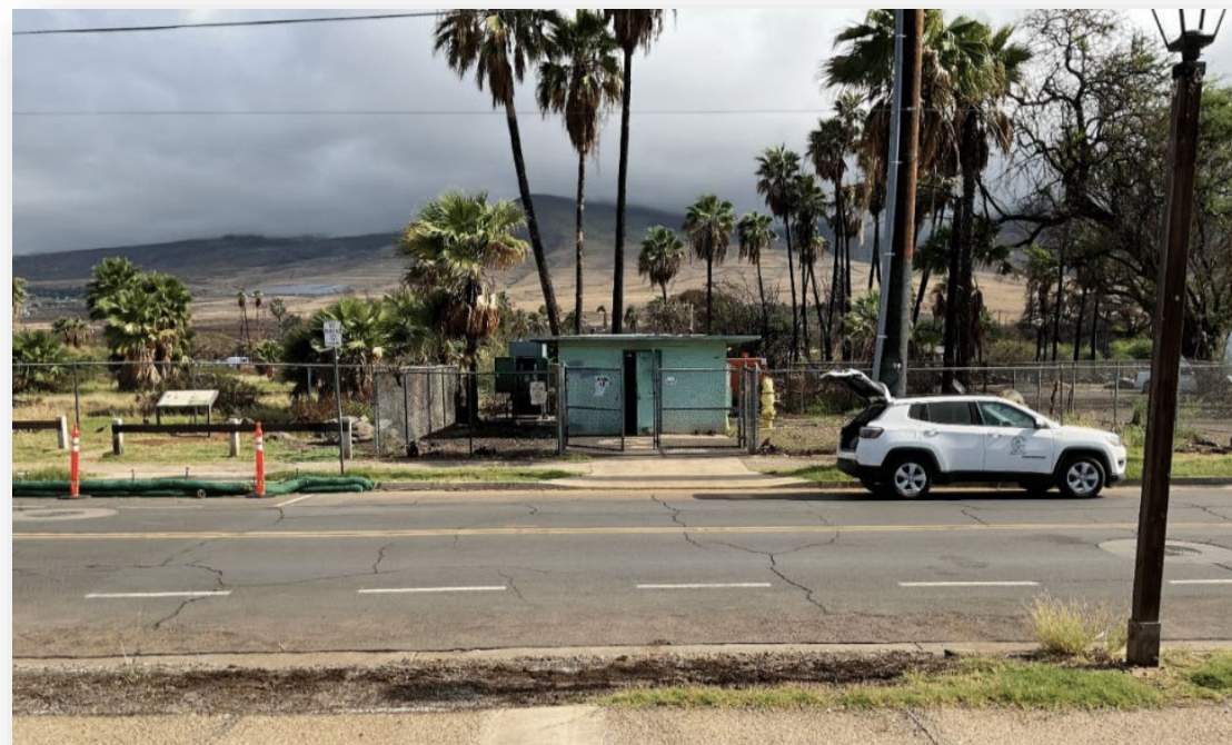
P.S. 4 – extensive wind and fire damage
