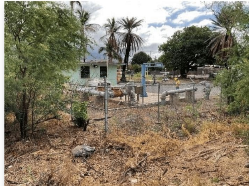
P.S. 4 – extensive wind and fire damage
