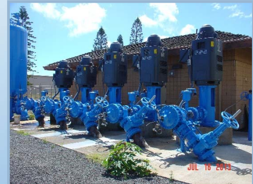
Booster Pump Stations
