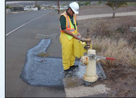
Waterlines & Fire Hydrants
