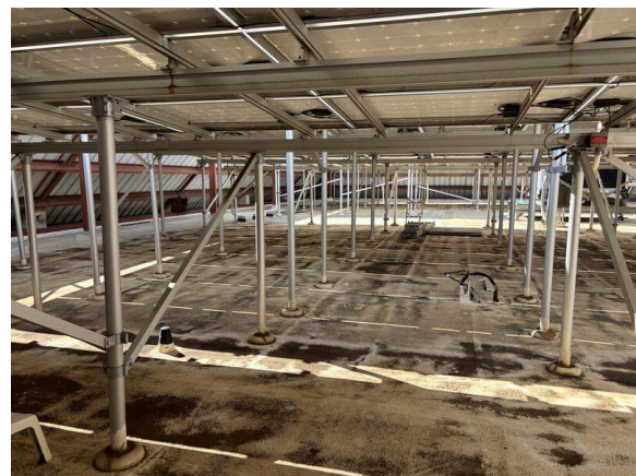
18 Underside of solar panel system at the roof
