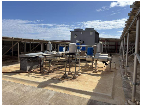
34 Main condenser at the roof
