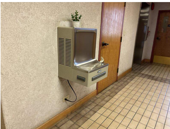
23 Typical drinking fountain on each floor
