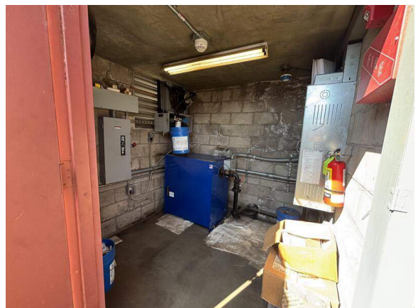
48 Elevator machine room
