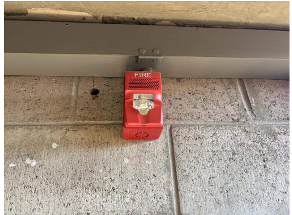
44 Fire alarm device
