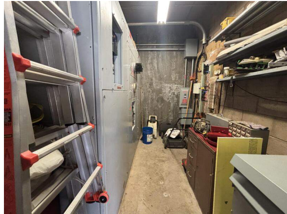
38 Main electrical room
