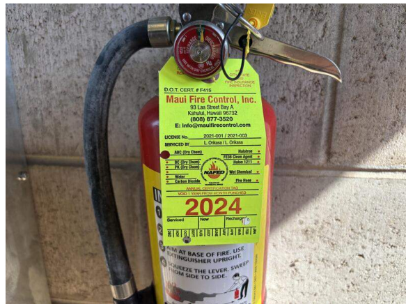
40 Typical fire extinguisher
