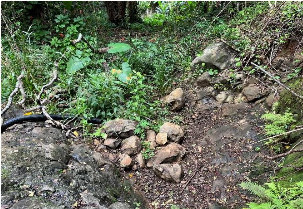
C) Unregistered stream diversion works in East Kuiaha Stream at approximately 510 ft a.s.l.
