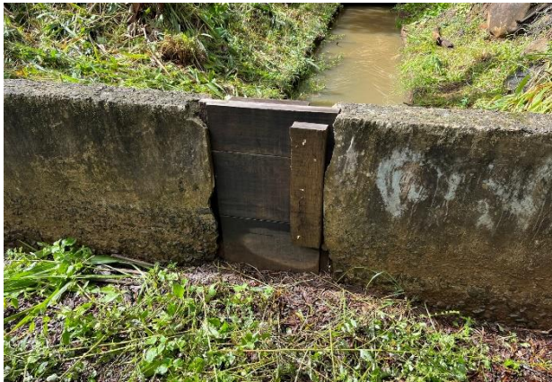
C) Closed intake on Kauhikoa Ditch diversion (KH-6) on East Kuiaha Stream.
