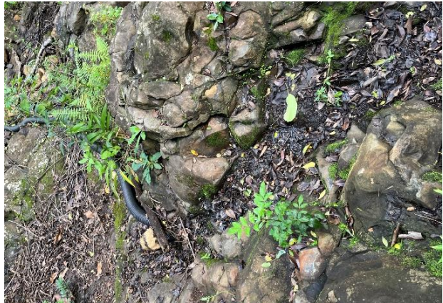
D) Unregistered stream diversion works in East Kuiaha Stream at approximately 510 ft a.s.l.
