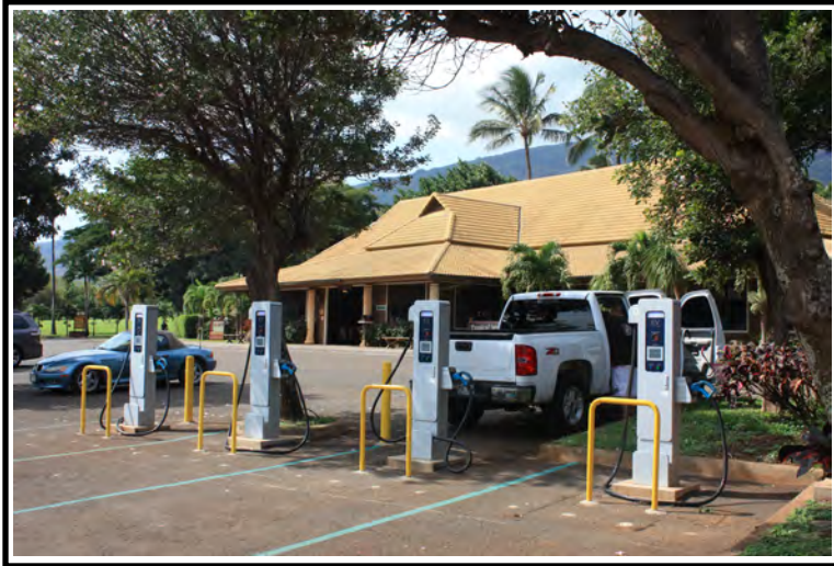
7. Existing electric vehicle recharging stations installed by JumpSmart Maui.
