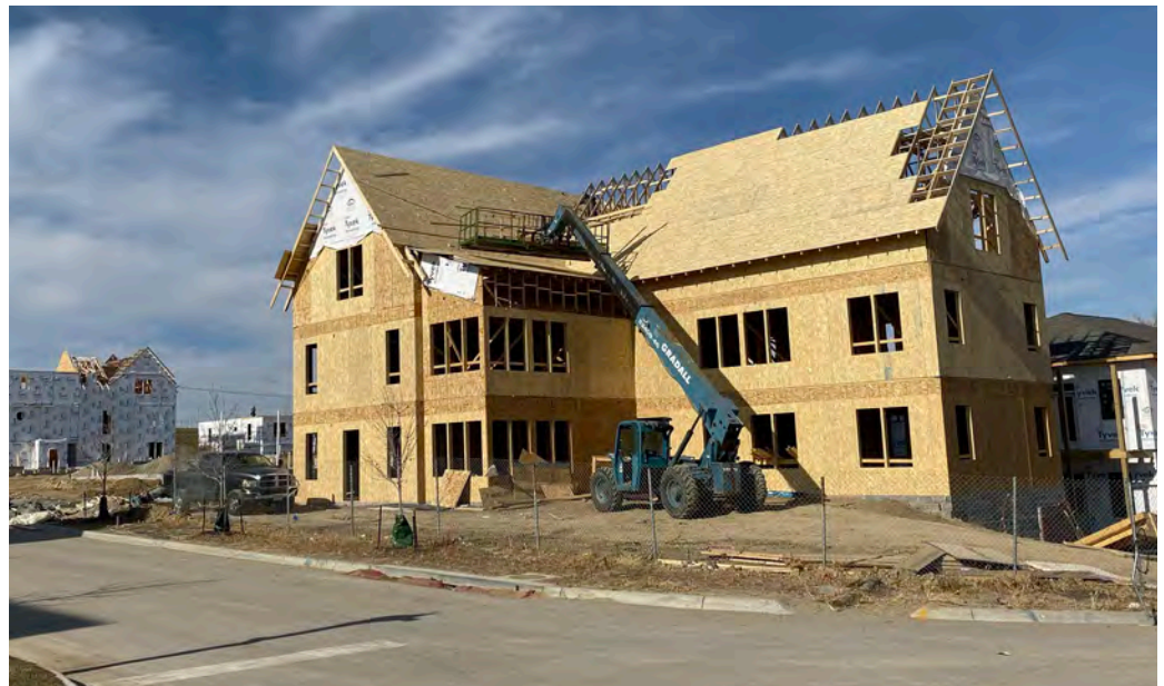
Figure 2.5 The simple forms, smaller size, and compatibility with Type V construction help maximize affordability and investment returns, and are consistent with the construction strategies familiar to most residential homebuilders, as shown in this under-construction MMH project in Papillion, Nebraska.
