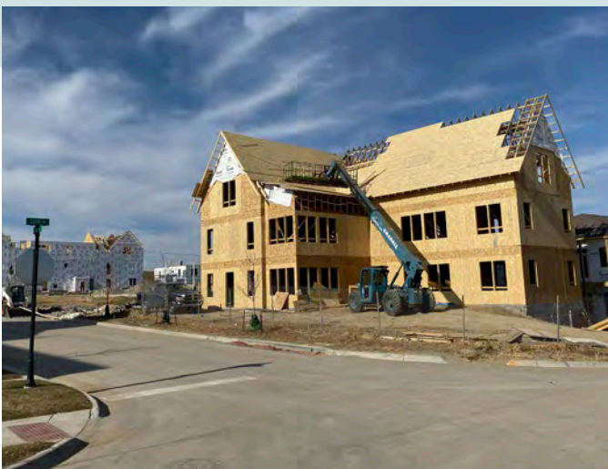
Figure 2.4 A MMH project under construction in Papillion, NE. The simple forms, smaller size, and compatibility with Type V construction help make MMH projects affordable to build compared to typical single-family homes, and such projects can be undertaken by the average residential homebuilder.
