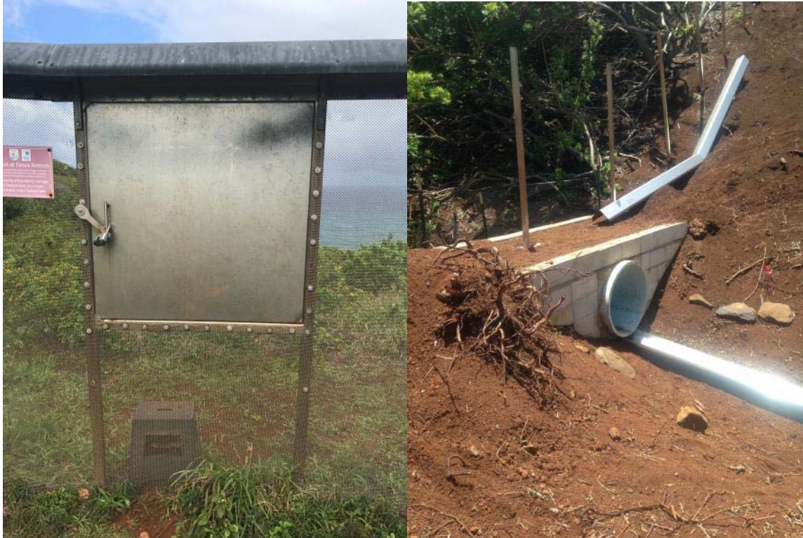
Figure 14: Nihoku pedestrian gate (left) and culvert (right). The culvert is shown during construction. Fence exterior is on the right; mesh was placed over the inside of the culvert opening to prevent debris from getting into the culvert and to prevent rodents from entering.
