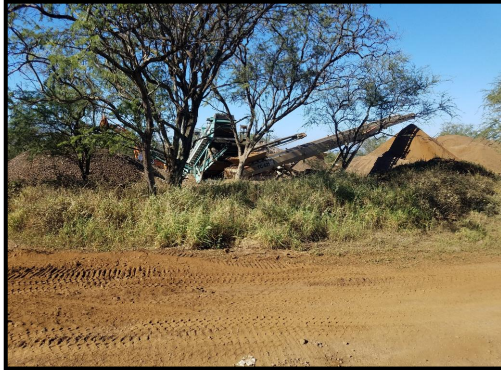
(2) 2-1-005:137 (Mo'oloa Ranch LLC) – Graded parcel for rock crushing and stockpiling without permits.
