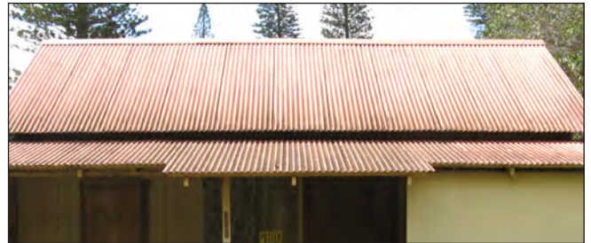
Corrugated metal is the most common roofing material in Lāna'ī City. Photo: Stanley Solamillo.
