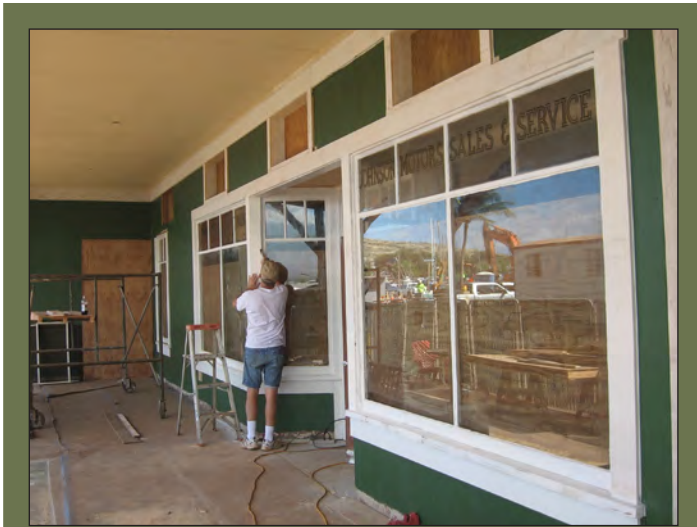
Instead of being replaced, these original storefront display windows were repaired in a way that preserved their historic character. Repair original windows when possible instead of replacing them. Photo: Stanley Solamillo.
