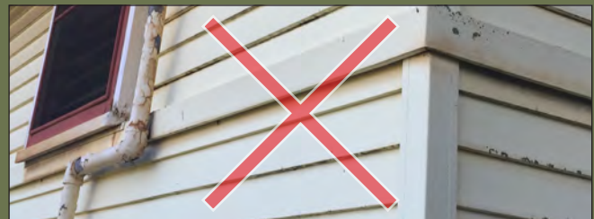
Do not cover original siding with vinyl.
