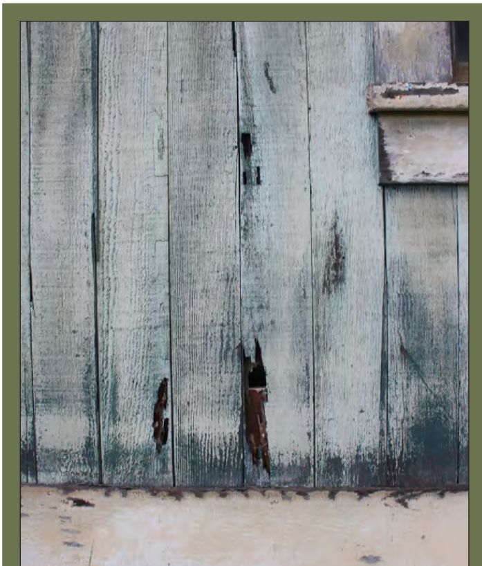
Pictured above is original tongue and groove siding. Repair original siding when possible instead of replacing or covering it.
