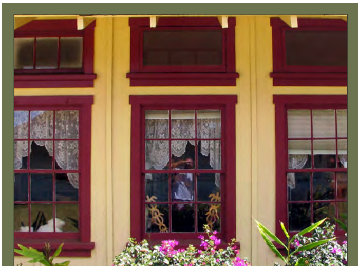
These original double-hung windows with transoms are unique and contribute to the character of this building. Photo: Chris Hart & Partners.
