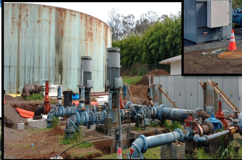
MALUHIA TANK BP STATION
