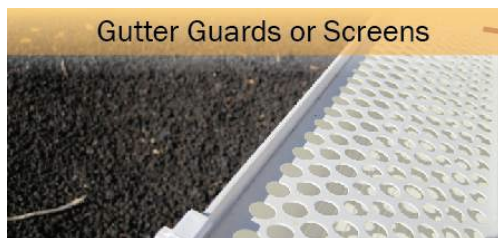
Figure 37. Rain gutters should have screens to keep leaf debris from accumulating. Maintain gutters to keep them clear and clean.
