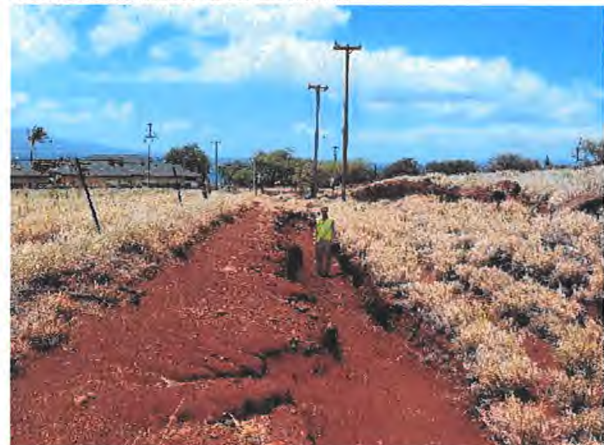
Failed Road with Channelization and Erosion
