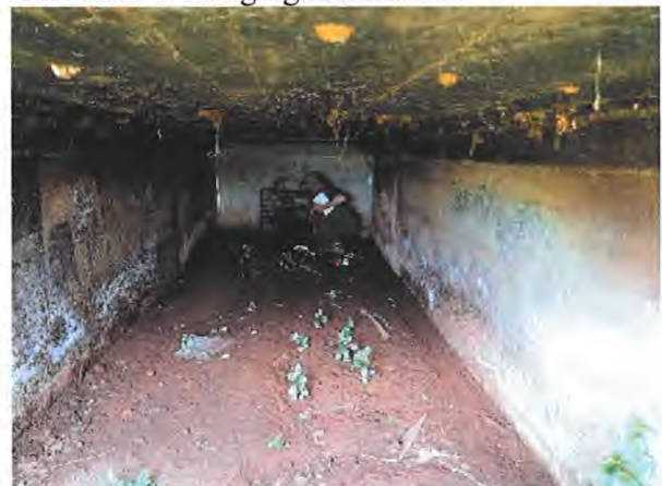
Substantial Sediment Deposition in Culvert
