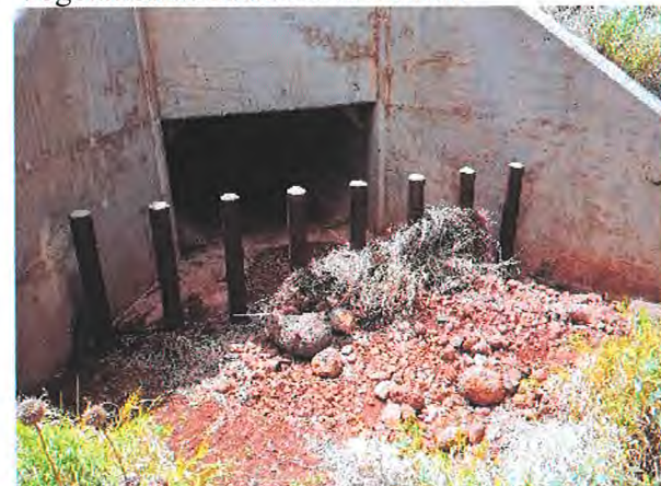
Sediment and Gravel at Culvert Entrance
