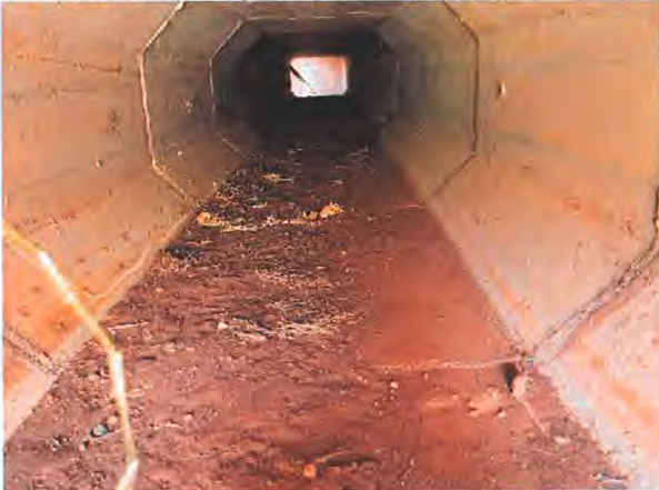
Sediment in Culverts
