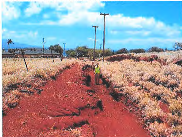
Distribution Lines and Failed Roads
