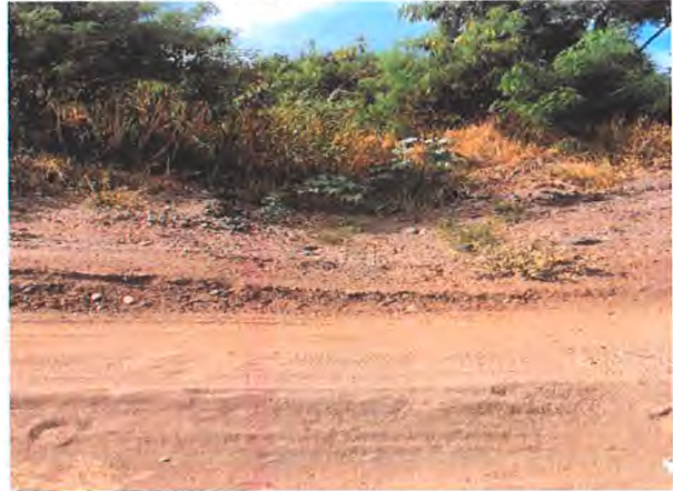
Road Crossing Pohakea Lacking BMPs
