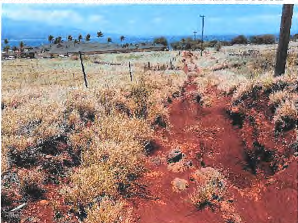
Failed Road with Channelization and Erosion
