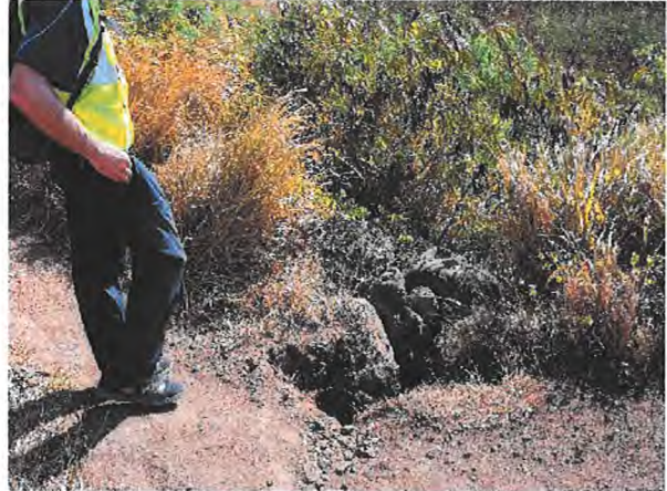
Erosion and Discharge from Road
