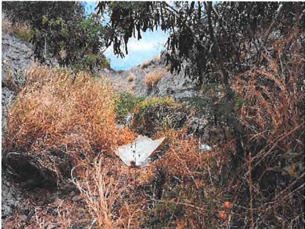
Vegetation and Rubbish in Ditch
