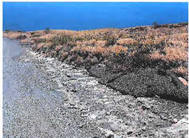
Gravel Loss in Swale
