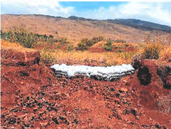
Failed Control Structure
