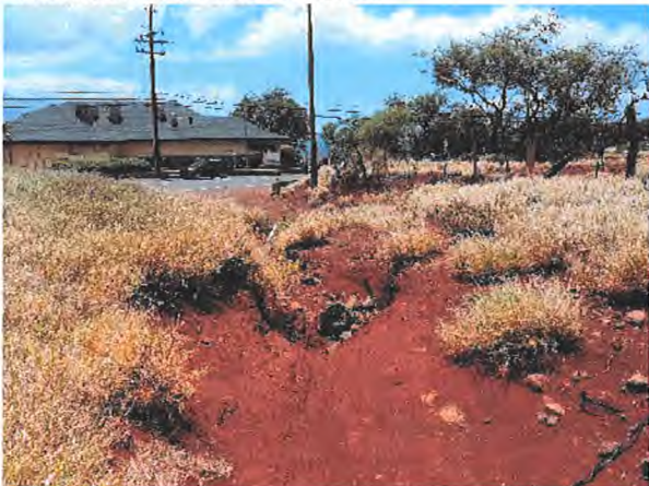
Failed Road with Channelization and Erosion
