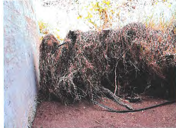
Vegetation at Entrance to Culvert
