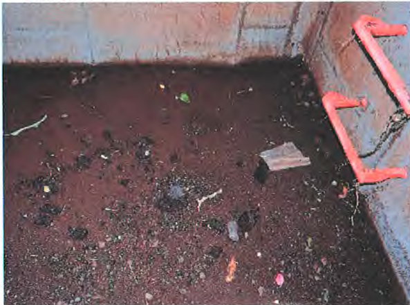
Sediment and Gravel in Culverts
