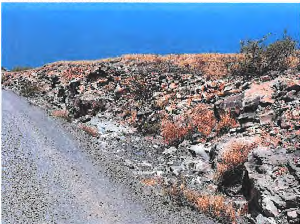
Channelization and Gravel Loss in Swale
