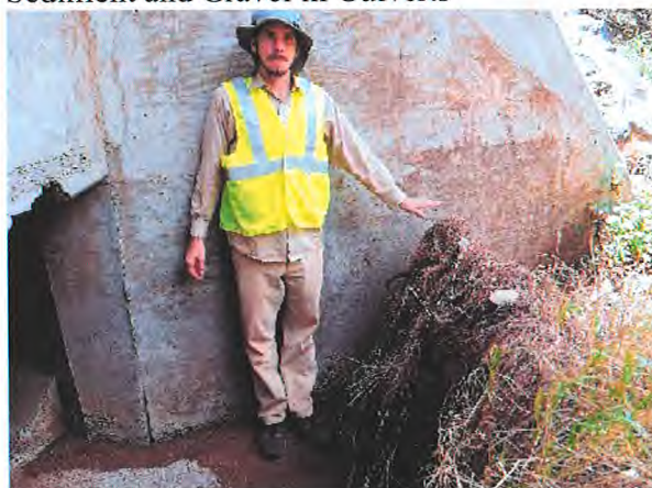
Extent of Vegetation at Entrance to Culvert
