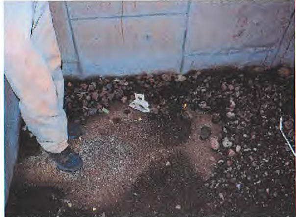
Sediment and Gravel in Culverts
