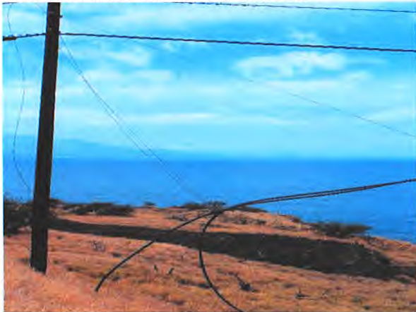
Downed Communications Lines
