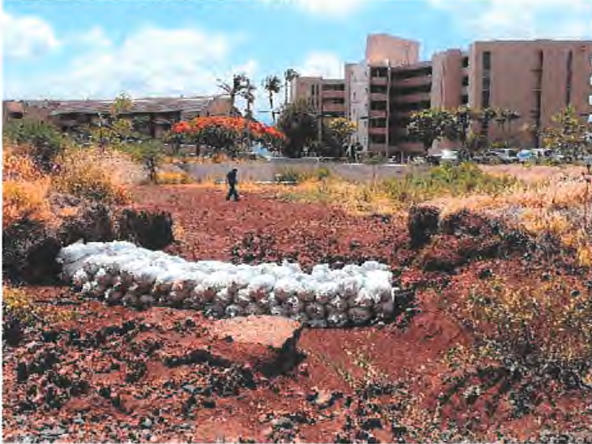
Sand Bags at Failed Control Structure
