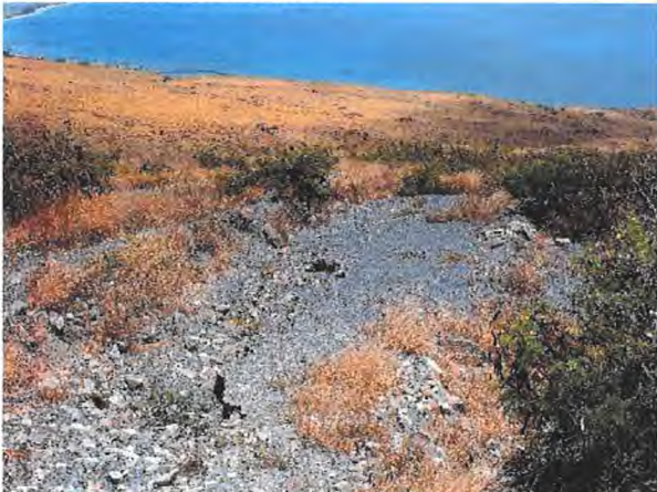
Gravel Loss at Kickouts
