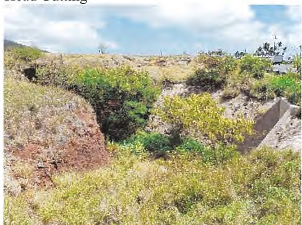
Culvert Backwall and Head Cutting
