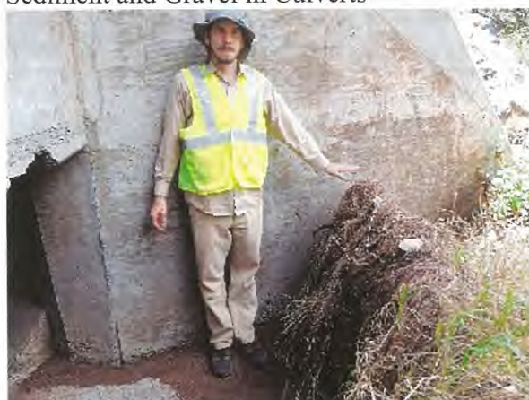
Extent of Vegetation at Entrance to Culvert
