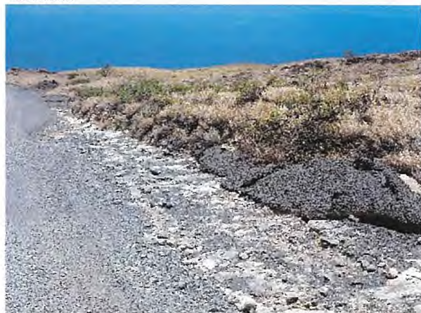
Gravel Loss in Swale
