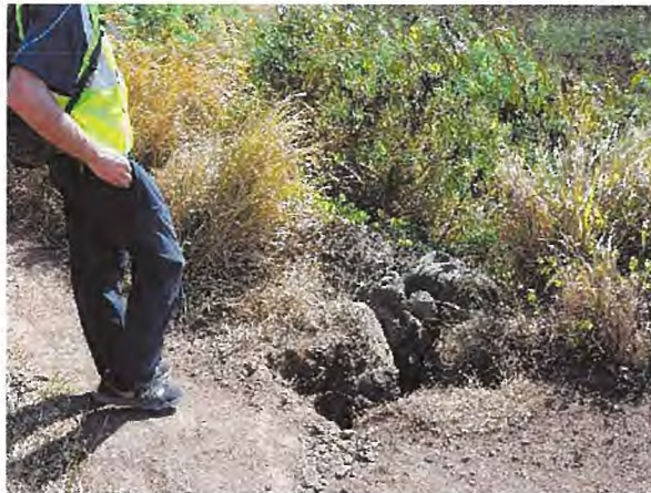
Erosion and Discharge from Road
