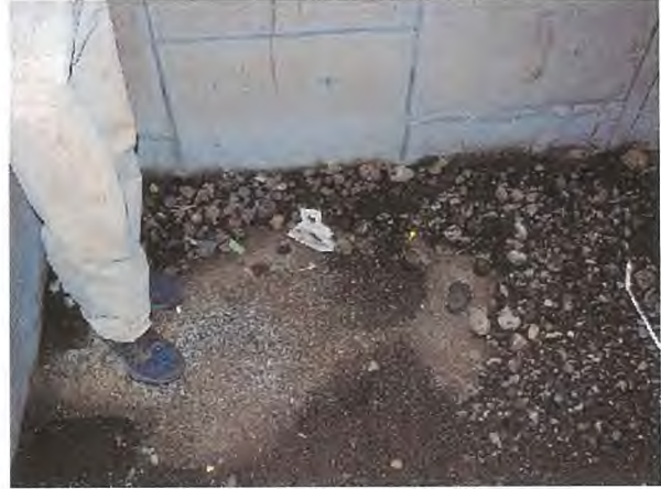
Sediment and Gravel in Culverts
