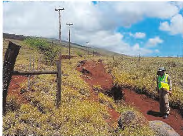
Channelization and Erosion
