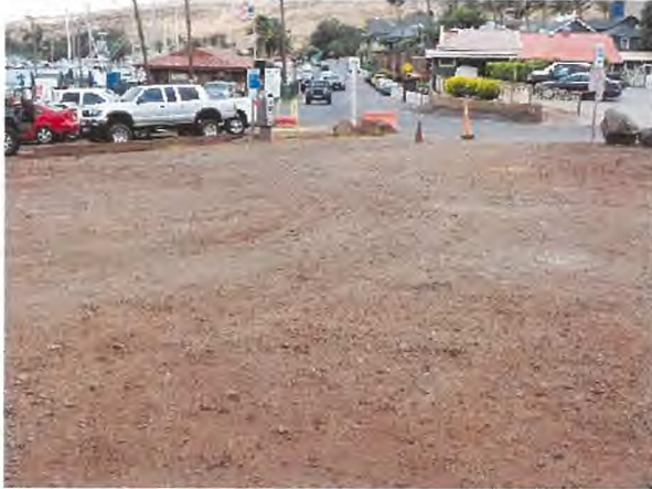
Dirt Lots with No BMPs in Place
