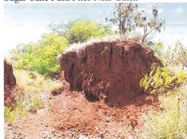
Evidence of Severe Erosion
