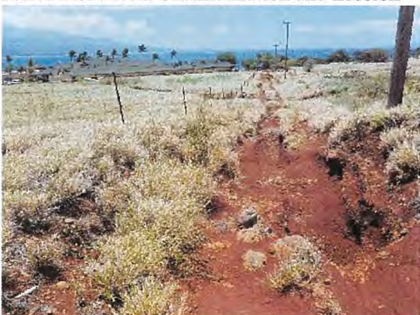
Failed Road with Channelization and Erosion
