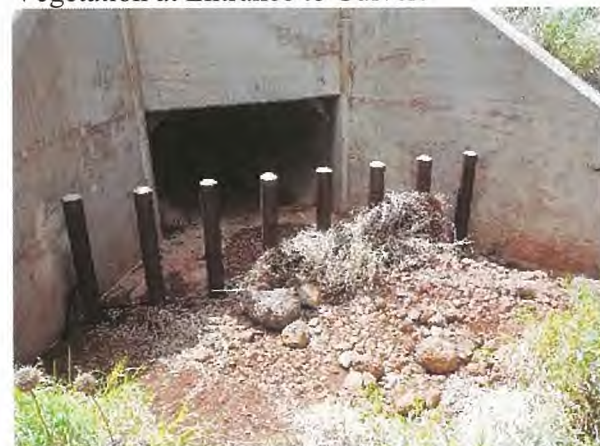
Sediment and Gravel at Culvert Entrance
