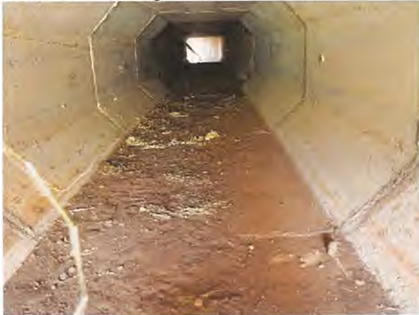
Sediment in Culverts
