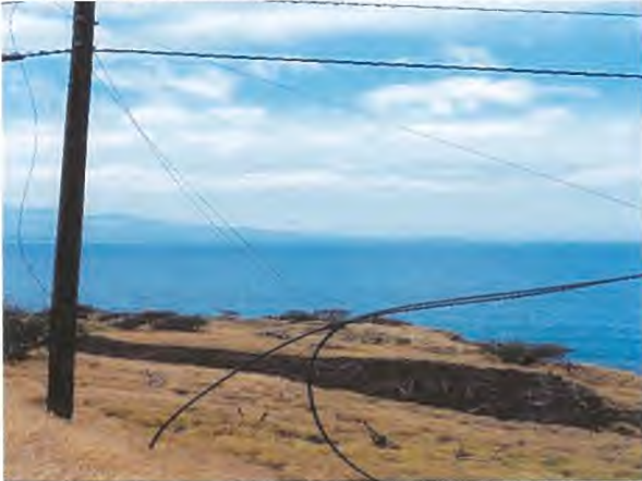
Downed Communications Lines
