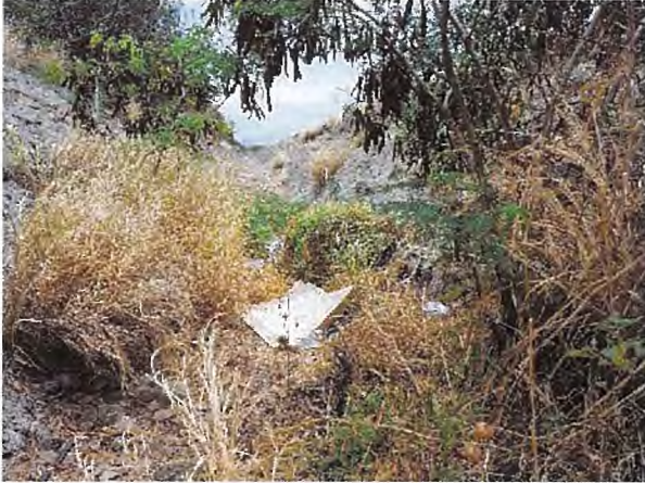
Vegetation and Rubbish in Ditch
