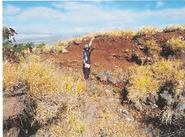
Extent of Erosion
