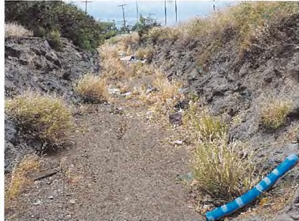
Rubbish in Ditch
