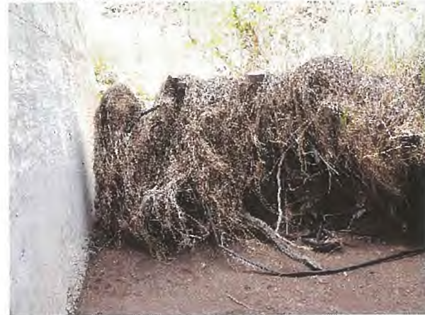
Vegetation at Entrance to Culvert
