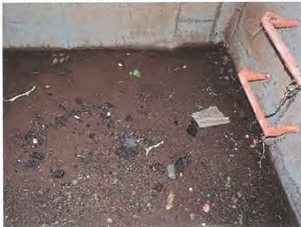
Sediment and Gravel in Culverts
