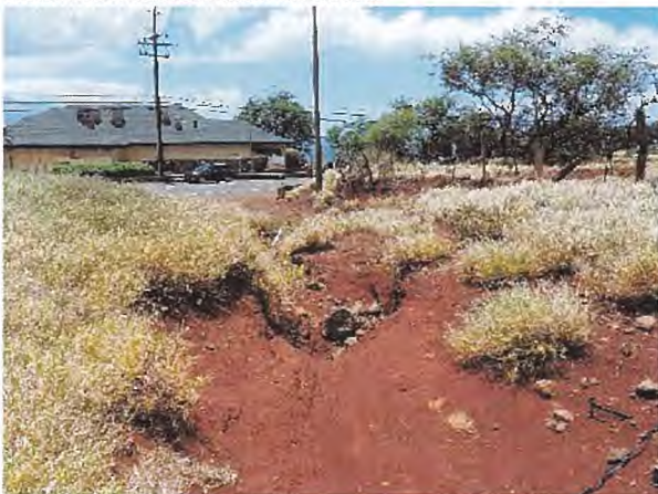
Failed Road with Channelization and Erosion
