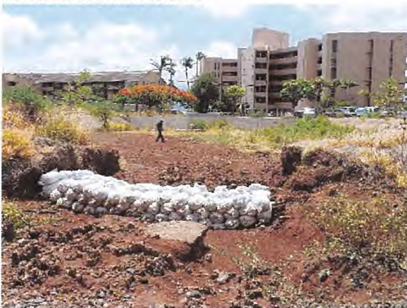
Sand Bags at Failed Control Structure
