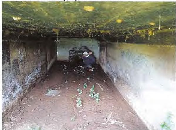
Substantial Sediment Deposition in Culvert
