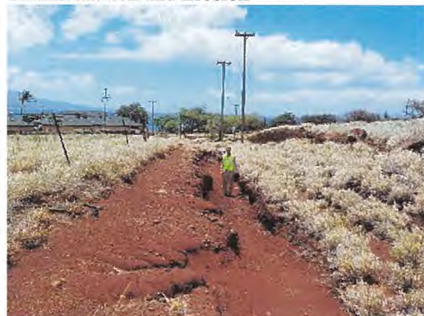
Failed Road with Channelization and Erosion
