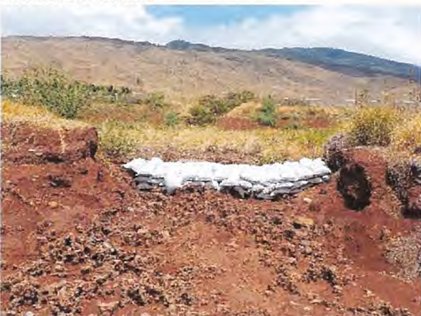
Failed Control Structure
