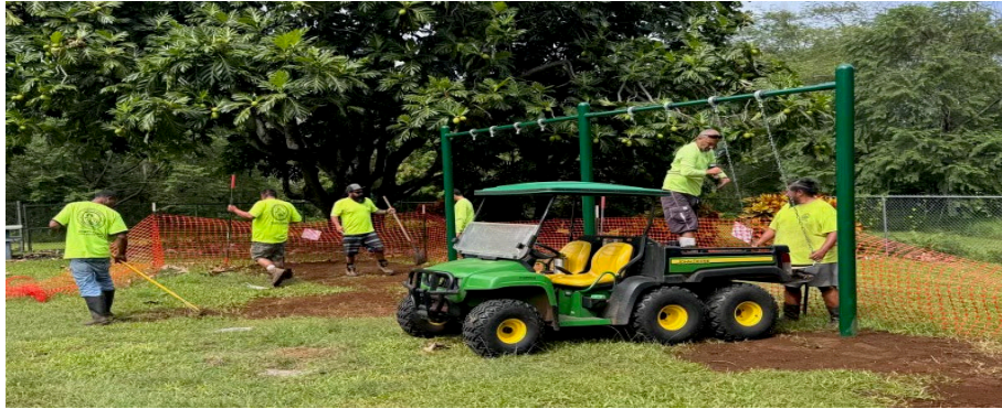
Parks District Maintenance Crew- Hana Parks Crew install of swingset at Pa'ani Mai Park
