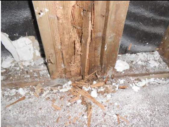
PC1D.4: Post termite damage.
