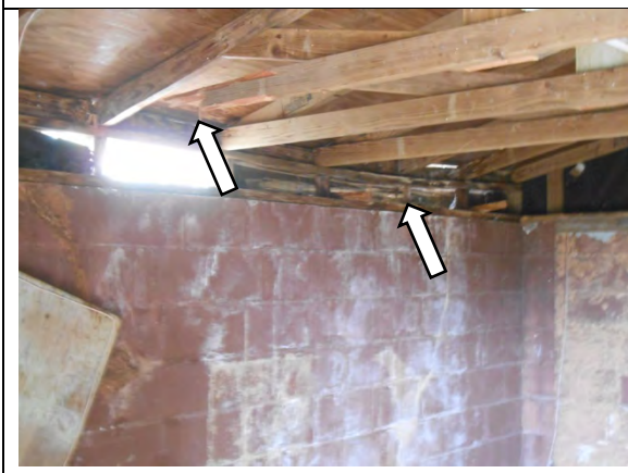
PTESB6: Collapsed storage building south wood framed stem wall. Damaged truss bottom chord.
