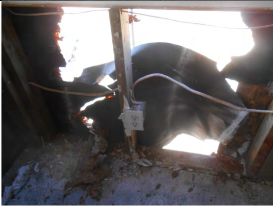
PB2D.3: Sheathing dry rot.
