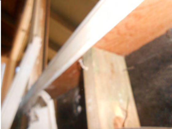
PA2CD.2: Missing opening sill plate. Window supported on studs.
