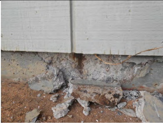
PC1D.1: Concrete spall with exposed corroded reinforcing steel.
