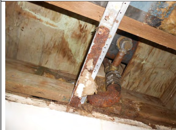
PC2D.2: Moisture damage to floor sheathing adjacent to rusting pipe.
