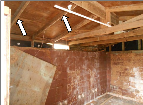
PTESB7: Damaged trusses. Missing truss framing.
