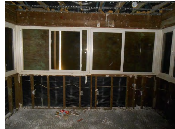
PA1CD.7: At various locations, wide wall opening with single sill plate.
