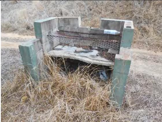
PBP1: Damaged concrete masonry unit barbecue pit. Missing blocks, cracked masonry, and warped concrete fire slab.
