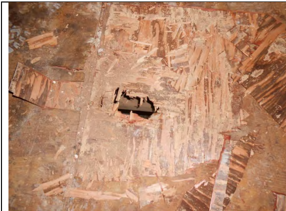
PB2D.1: Floor sheathing dry rot.
