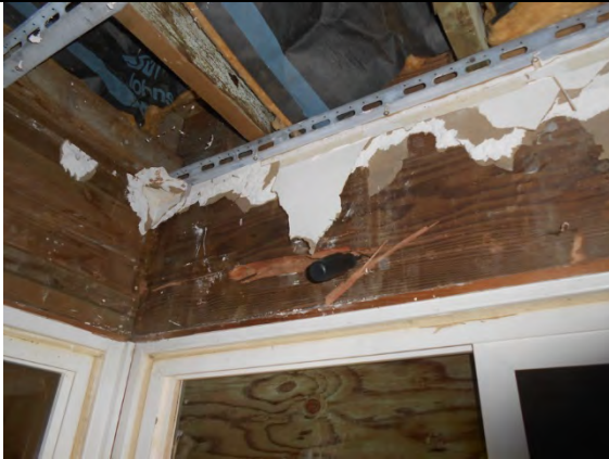
PB1D.5: Beam termite damage.
