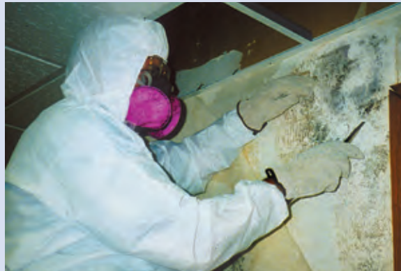
Photo 7: Remediation worker with limited PPE
