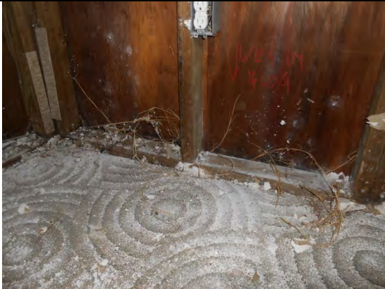
PA1CD.3: At various locations, vegetation is present at interior face of first story walls.
