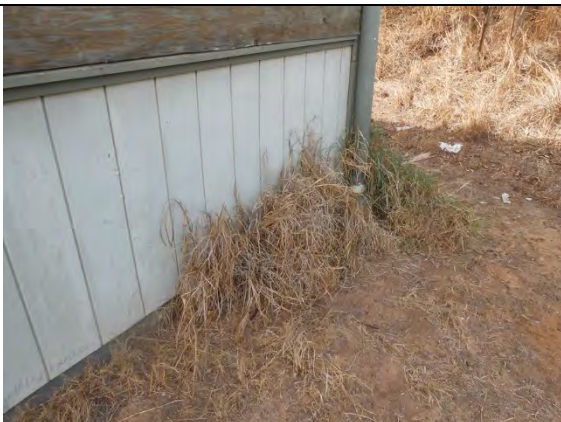
PC1CD.3: At various locations, vegetation against building façade.
