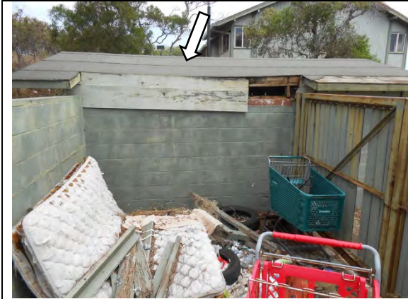
PTESB4: Damaged storage building roof.
