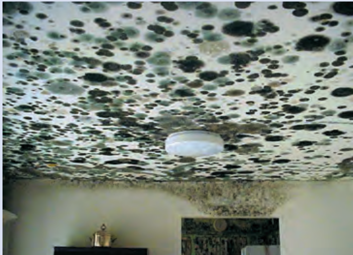
Photo 2: Extensive mold contamination of ceiling and walls
