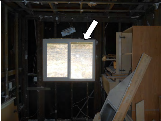
PC2CD.4: Missing opening header.
