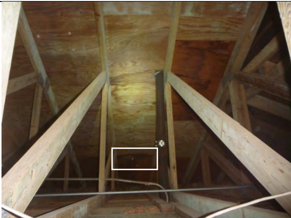
RCRD.2: Region of damaged plywood sheathing.
