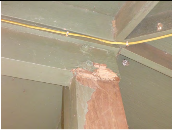
RCRD.1: Moderate termite damage present at beam to column connection at Gridlines '5-D'.
