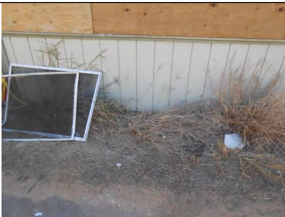
PB1CD.4: Vegetation against building façade.
