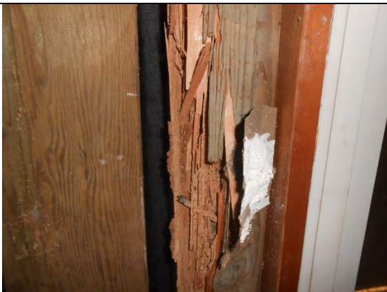
PB1D.3: Post termite damage.
