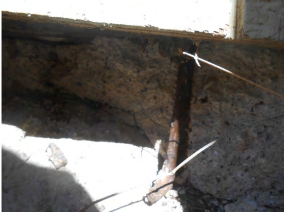
PA1D.3: Concrete spall with exposed corroded sole plate anchor rod.
