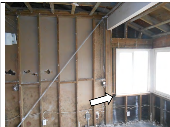
PC2CD. 1: Missing opening king post.
