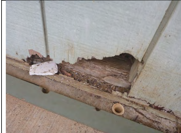
RC1D.4: Sole plate dry rot at heater room.
