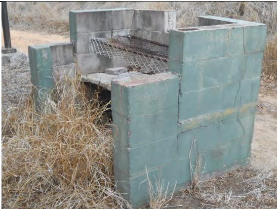
PBP2: Damaged concrete masonry unit barbecue pit. Missing blocks, cracked masonry, and warped concrete fire slab.
