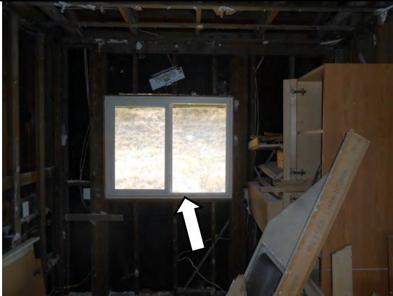
PC2CD.3: Missing opening sill plate.
