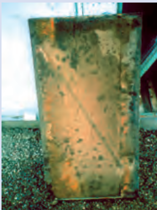
Photo 4A: Contaminated fibrous insulation inside air handler cover
