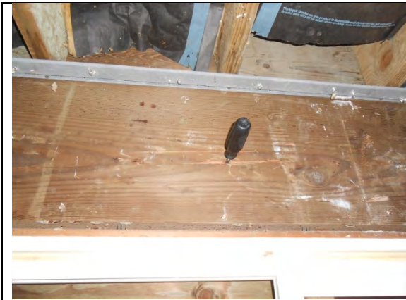
PC2D.1: Beam termite damage.
