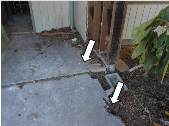
PA1D.5: Cracked exterior slab at rusting drain-pipe.
