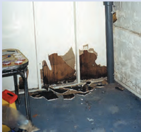
Photo 3B: Front side of wallboard looks fine, but the back side is covered with mold
