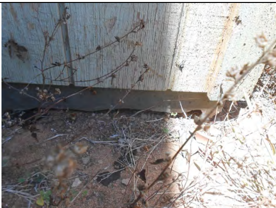
PB1CD.5: Exposed bottom of footing.
