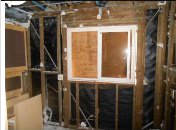
PC1CD.1: Missing opening king post.
