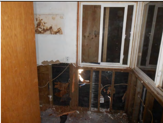
PB1D.2: Siding dry rot.
