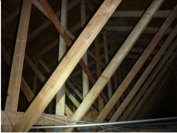
RCRCD.1: Web bracing missing.
