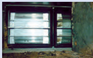
Photo 4C: Moldy air duct
