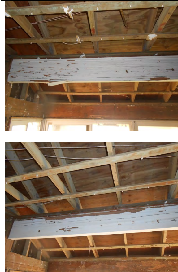
PBRD.1: Beam termite damage.
