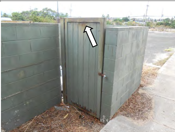
PTESB3: Rusting trash enclosure door.
