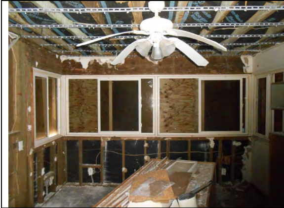
PB2CD.2: Missing blocking
