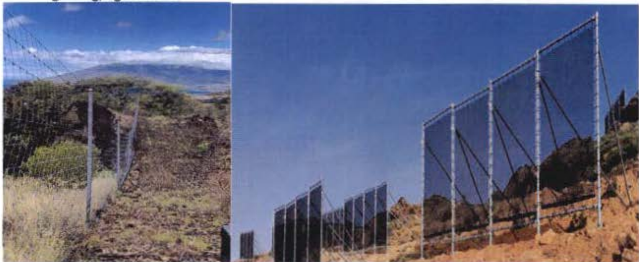
Images of fence work done at Pu'u-o-kali at left, with rocks covering apron to prevent cattle from being stuck. At right, example of fog drip capture system Dr. Juvik installed at another site.
