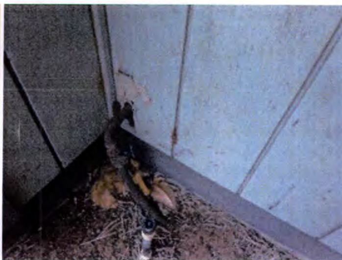
Copper supply plumbing
