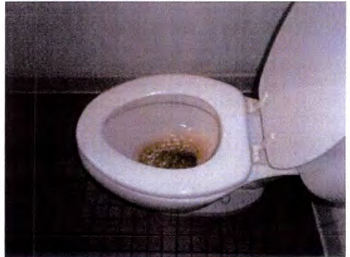
Building A bathrooms appeared to be in functional condition at the time of inspection.
