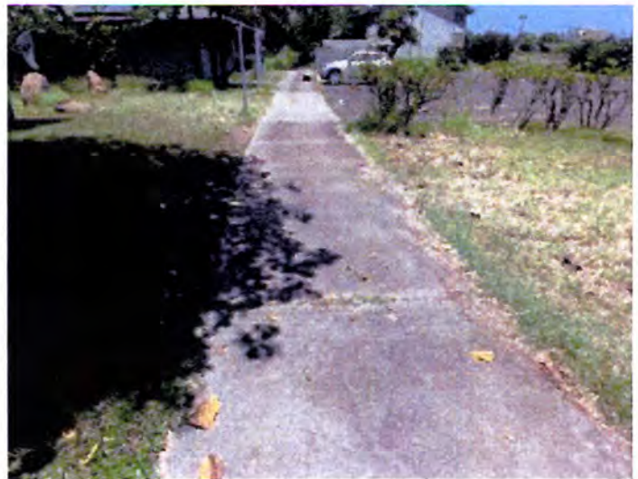
The sidewalks appeared to be intact and functioning properly at the time of inspection.
