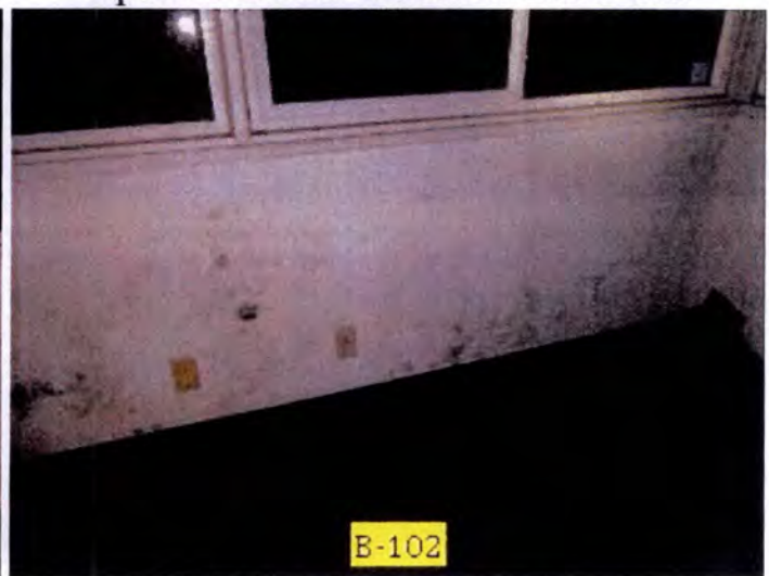
Visible indications of moisture intrusion and mold growth at building B and C interior, bedroom, bathroom and closet wall areas. Recommend removal and replacement of all interior wall finishes of B and C, after removal of all exterior vegetation.
