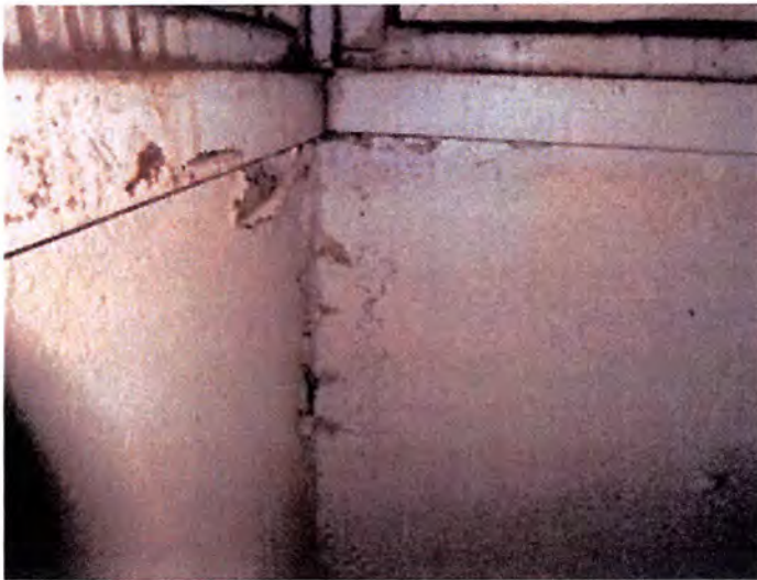
Most of the exterior facing lower interior wall finishes had moisture damage observed. Recommend removal and replacement of affected materials.
