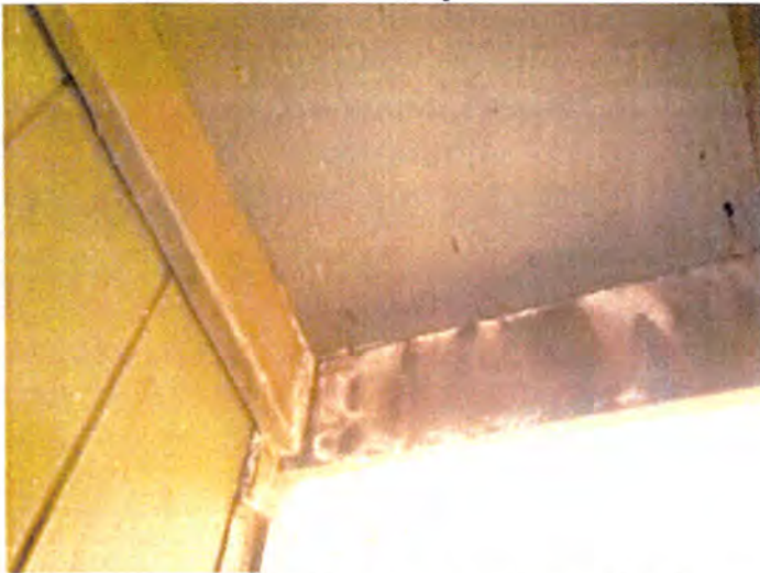
The fascia/soffit areas appeared to be rotted/water damaged/deteriorated at the time of inspection. Recommend having a licensed contractor evaluate and repair/replace as necessary.
