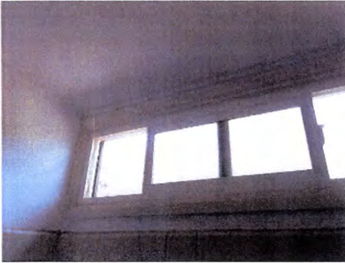
Most of the tested windows operated properly when tested. Except as noted.
