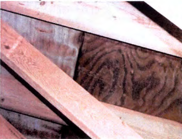
There were visible indications of mold present at all attic areas.
