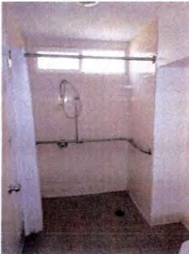
Building A ground floor bathrooms appeared to be in functional condition at the time of inspection.
