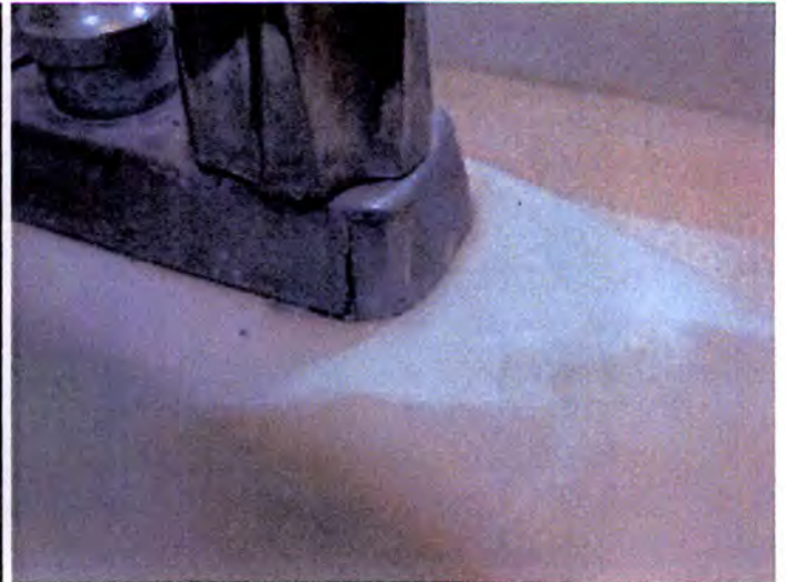
Based on the observed physical conditions of the installed fixtures, we recommend the replacement of all plumbing fixtures and shut off valves in all buildings to ensure proper future operation.
