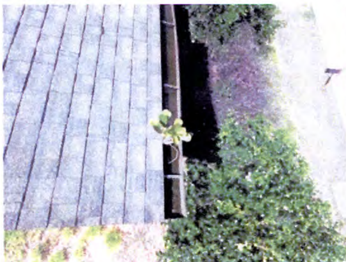
Damaged/broken/missing gutters noted. Recommend having a licensed contractor evaluate and repair/replace as necessary.
