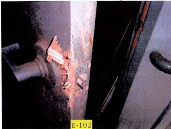
The exterior doors were termite damaged or deteriorated to the point of being inoperable. We recommend replacement of all exterior doors, framing and trim for all buildings.
