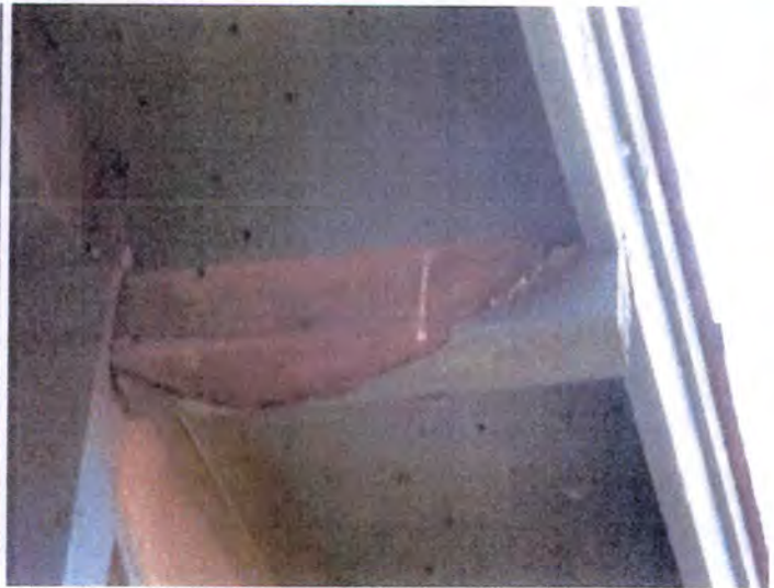
Blistering/peeling/missing paint observed at many exterior trim, fascia and soffit areas. Recommend properly preparing and refinishing exterior finishes.
