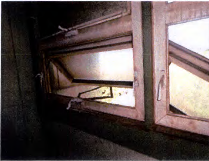
The stair way windows were heavily corroded, damaged and/or inoperable at the time of inspection. Recommend replacement.
