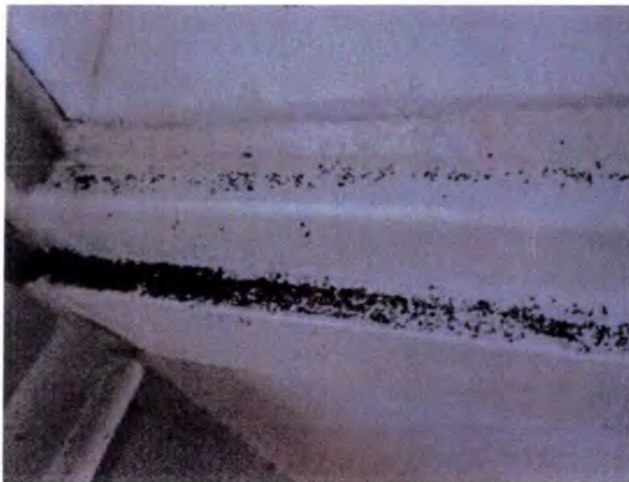
There were visible indications of moisture and termite damage observed at the interior window trim areas. Recommend replacement of all interior window trim and finishes.
