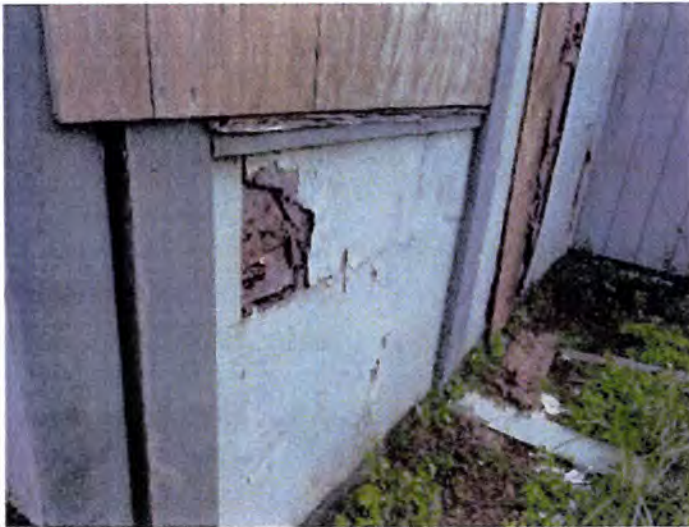
Moisture damage observed at exterior wall areas. Recommend select demolition and replacement of affected ground level exterior siding and finishes.
