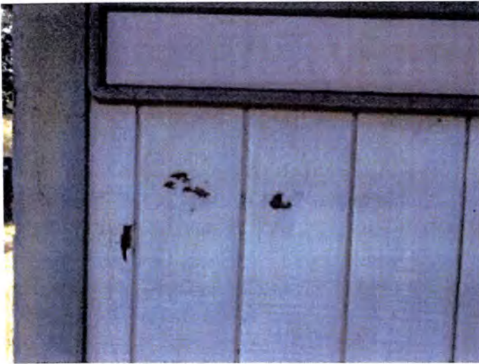
Visible indications of WDO (termite) damage noted. Recommend having a licensed pest contractor evaluate and treat as necessary. Also, recommend having a licensed contractor evaluate and repair/replace damaged material as necessary.
