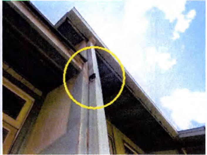
Damaged/broken/missing gutters noted. Recommend having a licensed contractor evaluate and repair/replace as necessary.
