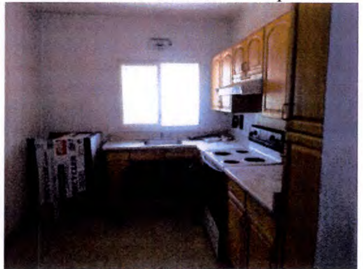
The kitchens in building A appeared to be functional at the time of inspection.
