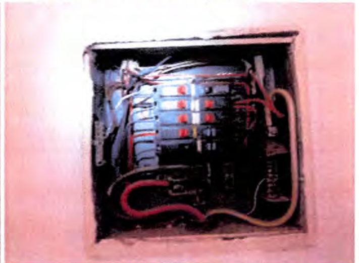
Each dwelling unit was serviced by one electrical cabinet at the time of inspection.
