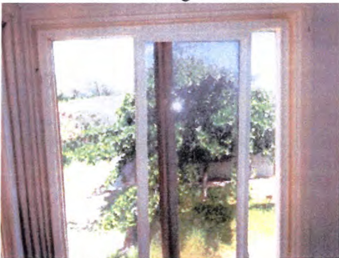
Most of the tested windows operated properly when tested. Except as noted.
