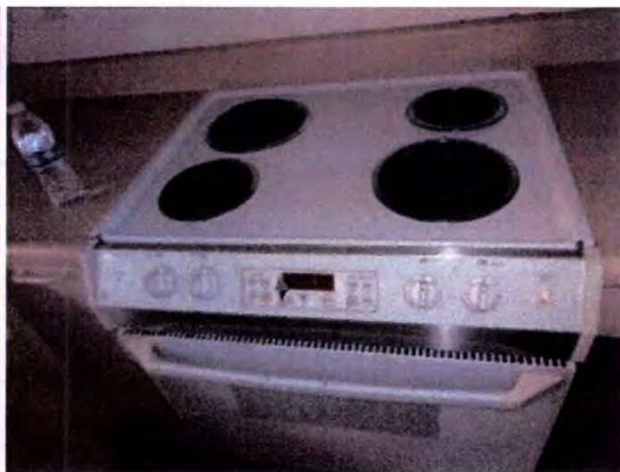
The kitchens in building A appeared to be functional at the time of inspection.
