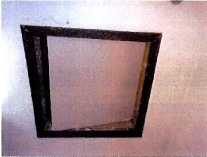
There were attic accesses located in the following locations: All second floor dwelling units.
