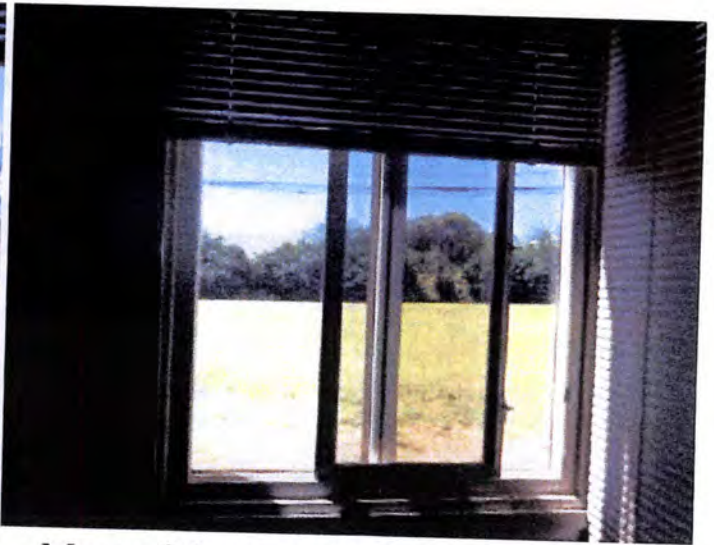
Most of the tested windows operated properly when tested. Except as noted.
