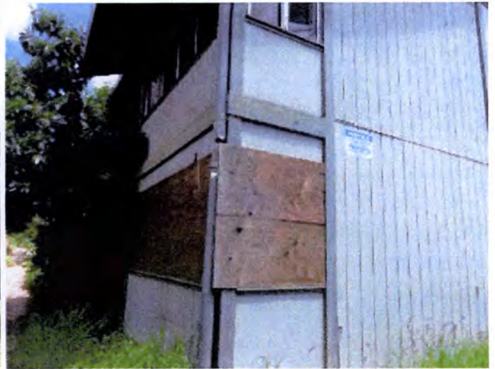
Many of the ground floor windows were broken at the time of inspection.
