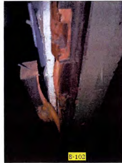
Most of the doors had varying degrees of damage observed when inspected. Based on the observed conditions, we recommend the replacement of all interior doors and trim within the dwelling units.
