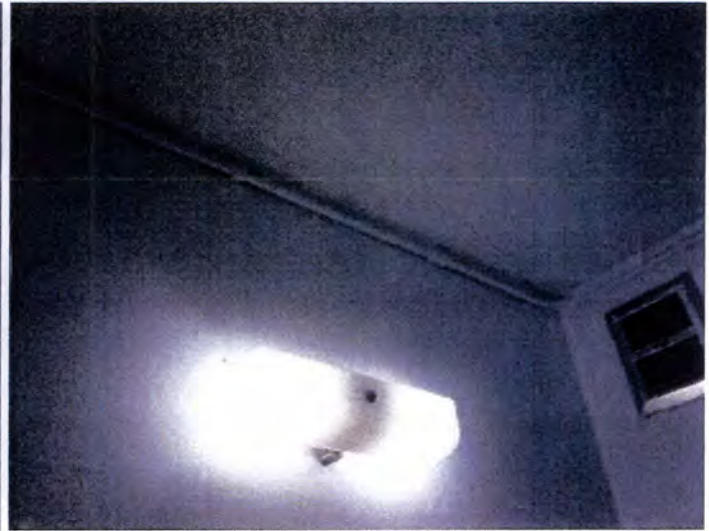
Building A's tested receptacles, switches and lights operated properly at the time of inspection. There were missing bulbs observed but power was present at the fixtures.
