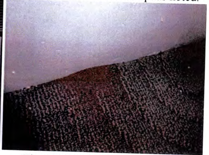
There were visible indications of moisture and termite damage observed at the interior window trim areas. Recommend replacement of all interior window trim and finishes.
