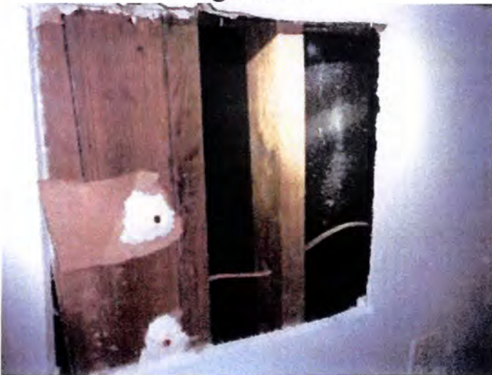
Visible indications of moisture intrusion and mold growth at building B and C interior, bedroom, bathroom and closet wall areas. Recommend removal and replacement of all interior wall finishes of B and C, after removal of all exterior vegetation.
