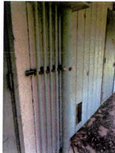
Service conductors are encased in rigid conduit
