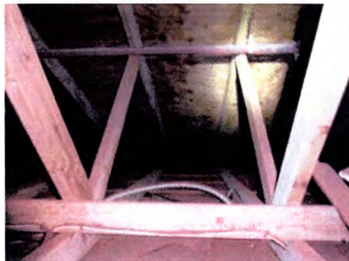
There were visible areas of moisture intrusion observed at the roof sheathing (within the attic spaces) at the time of inspection. This indicated a failed/failing roofing system. Recommend replacement of the installed sheathing and roofing finish.
