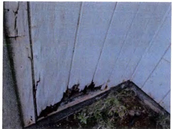
Visible indications of WDO (termite) damage noted. Recommend having a licensed pest contractor evaluate and treat as necessary. Also, recommend having a licensed contractor evaluate and repair/replace damaged material as necessary.
