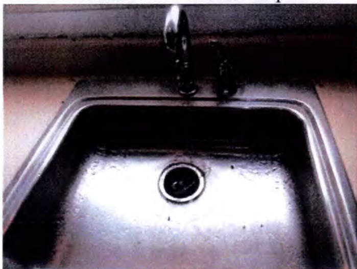
The kitchens in building A appeared to be functional at the time of inspection.
