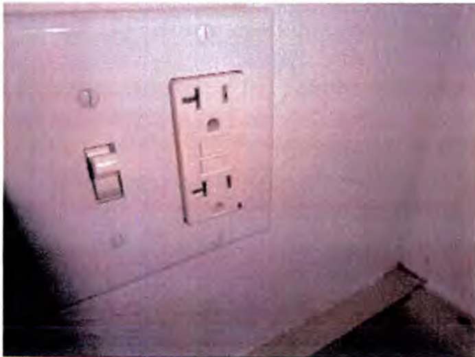
Building A's tested receptacles, switches and lights operated properly at the time of inspection. There were missing bulbs observed but power was present at the fixtures.
