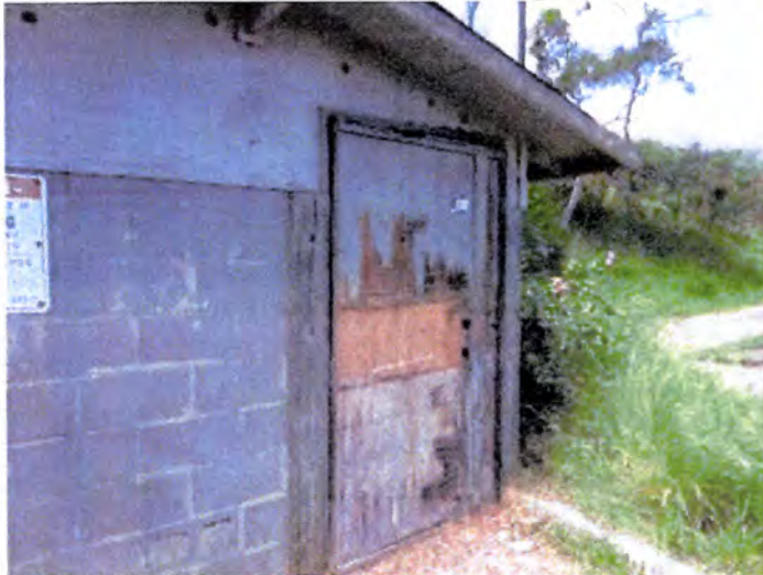
The exterior doors were termite damaged or deteriorated to the point of being inoperable. We recommend replacement of all exterior doors, framing and trim for all buildings.
