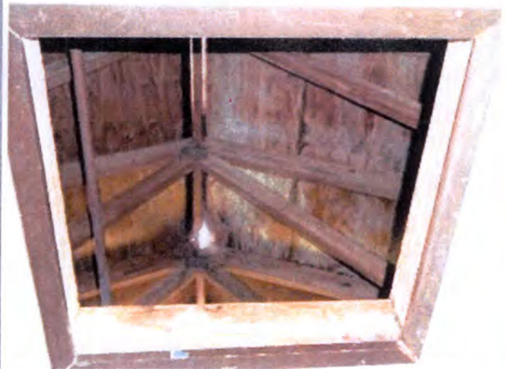
There were attic accesses located in the following locations: All second floor dwelling units.
