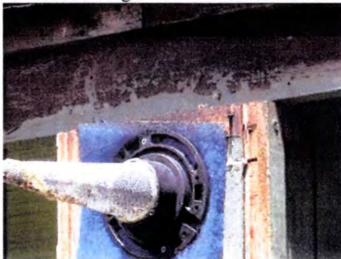
Some of the areas were inaccessible due to the presence of a robust bee population outside and inside of the buildings.
