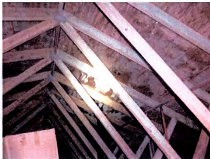
There were visible areas of moisture intrusion observed at the roof sheathing (within the attic spaces) at the time of inspection. This indicated a failed/failing roofing system. Recommend replacement of the installed sheathing and roofing finish.
