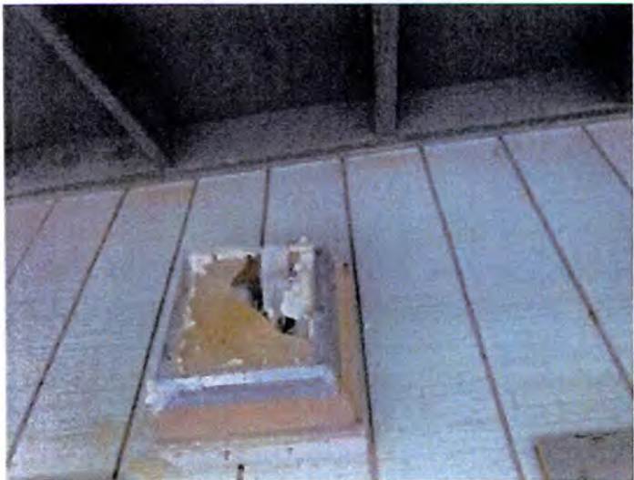
Some of the exterior lighting fixtures were damaged and need to be replaced.
