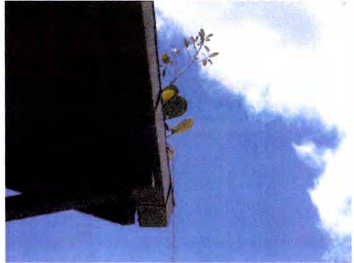
Vegetation growth observed in gutters. Recommend clearing.
