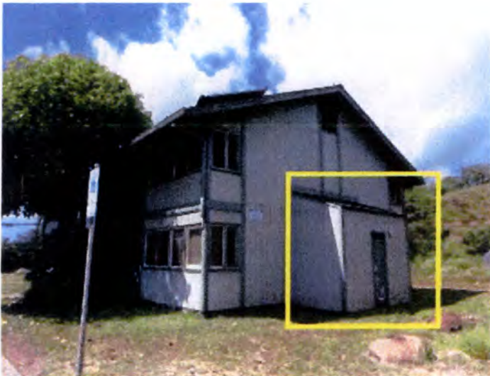
The fire suppression risers were located at the end of each building.
