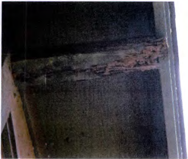
There were visible indications of WDO (Wood Destroying Organism) damage noted at the fascia and soffit areas. Recommend having a licensed contractor evaluate and repair/replace as necessary.
