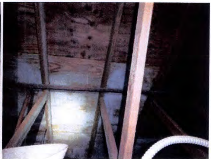
Visible indications of moisture intrusion and mold growth at building B and C interior, bedroom, bathroom and closet wall areas. Recommend removal and replacement of all interior wall finishes of B and C, after removal of all exterior vegetation.
