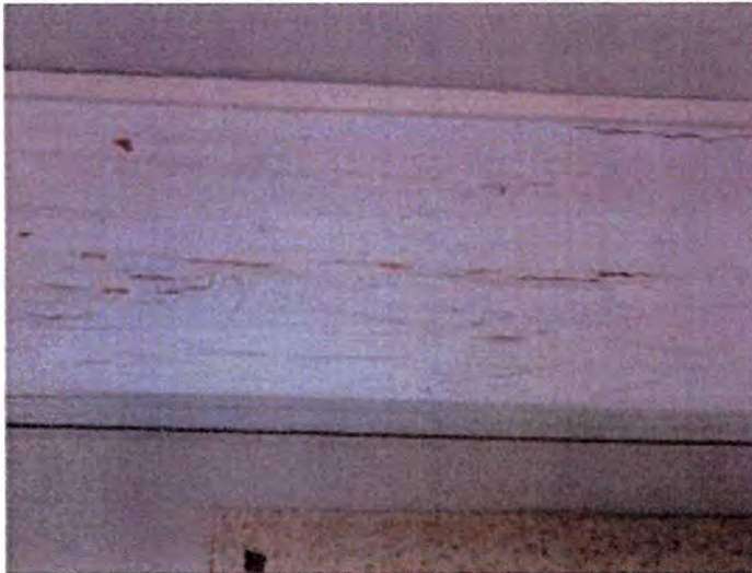
B-201: Ceiling joists were severely termite damaged and need to be repaired/replaced.
