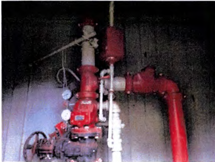
Sprinkler Systems: due to the system not having been properly serviced at required intervals, adequacy or performance questionable.
