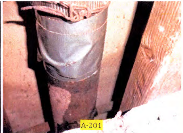
Non standard repairs observed at plumbing connections. Recommend repair.
