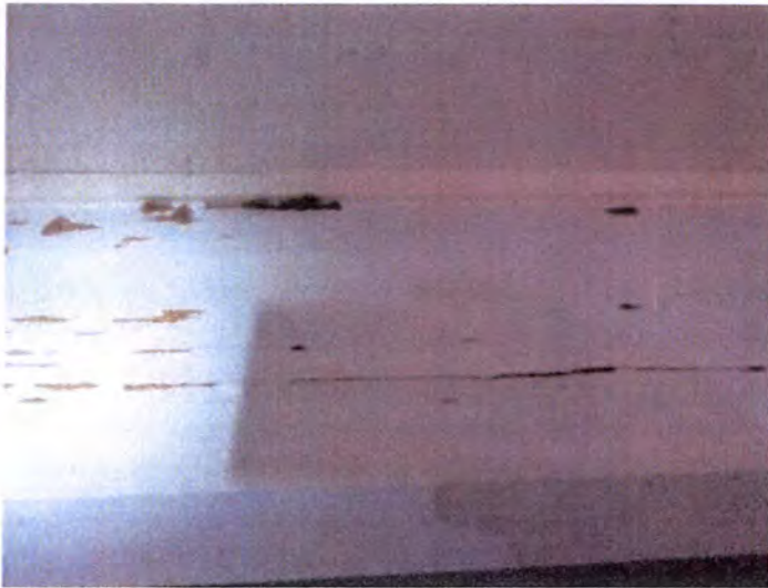
B-201: Ceiling joists were severely termite damaged and need to be repaired/replaced.
