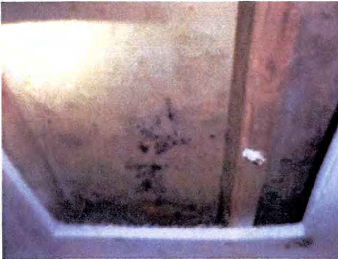
Visible indications of moisture intrusion and mold growth at building B and C interior, bedroom, bathroom and closet wall areas. Recommend removal and replacement of all interior wall finishes of B and C, after removal of all exterior vegetation.
