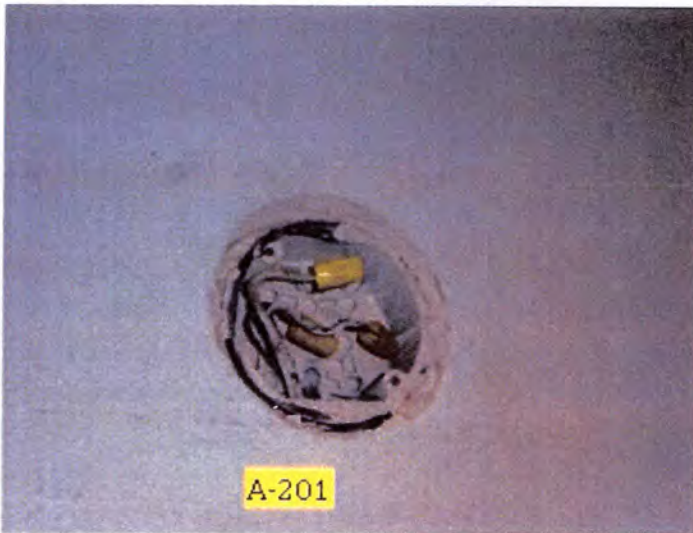
There were missing junction box covers noted at the following locations: attic spaces and front exterior of store.
