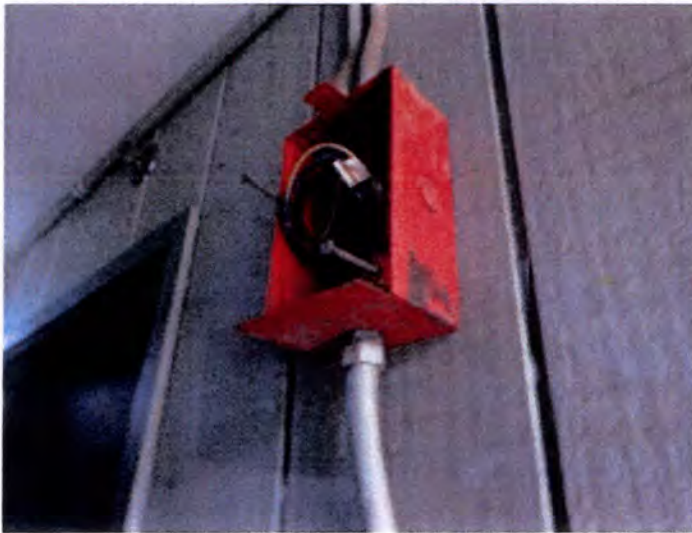
Approximately half of the installed pull stations were damaged when inspected. Recommend replacement/repair.
