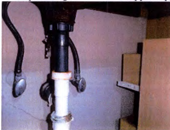
ABS/PVC waste/drain plumbing
