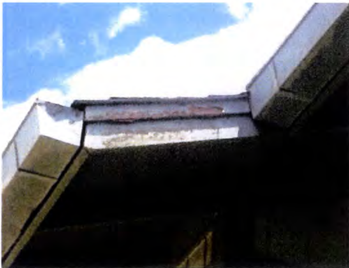
Blistering/peeling/missing paint observed at many exterior trim, fascia and soffit areas. Recommend properly preparing and refinishing exterior finishes.
