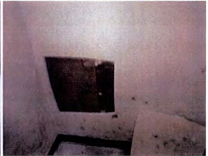
Most of the exterior facing lower interior wall finishes had moisture damage observed. Recommend removal and replacement of affected materials.
