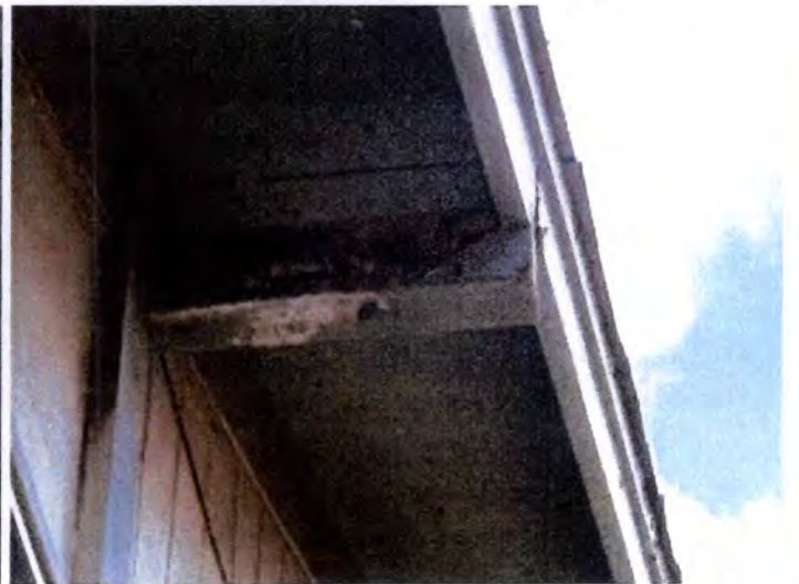
The fascia/soffit areas appeared to be rotted/water damaged/deteriorated at the time of inspection. Recommend having a licensed contractor evaluate and repair/replace as necessary.
