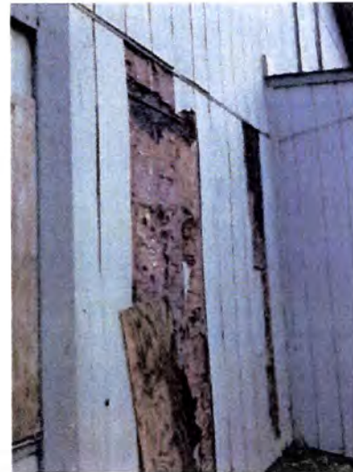
Visible indications of WDO (termite) damage noted. Recommend having a licensed pest contractor evaluate and treat as necessary. Also, recommend having a licensed contractor evaluate and repair/replace damaged material as necessary.
