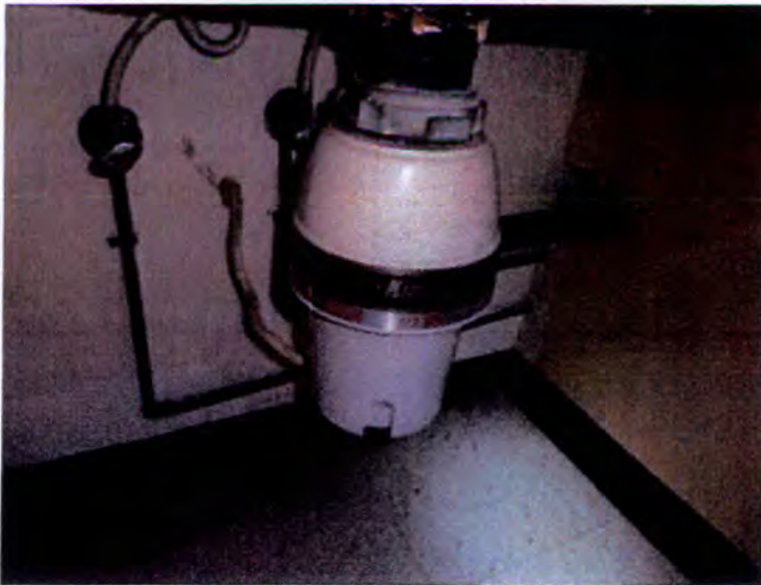
The kitchens in building A appeared to be functional at the time of inspection.
