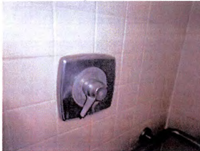
Based on the observed physical conditions of the installed fixtures, we recommend the replacement of all plumbing fixtures and shut off valves in all buildings to ensure proper future operation.
