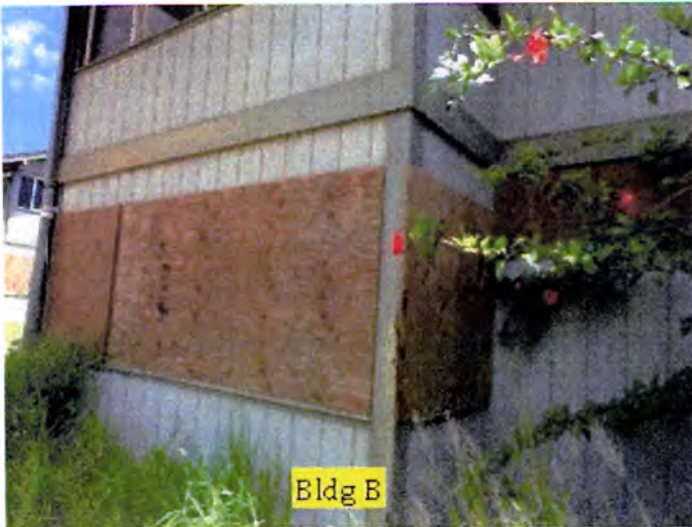
Many of the ground floor windows were broken at the time of inspection.
