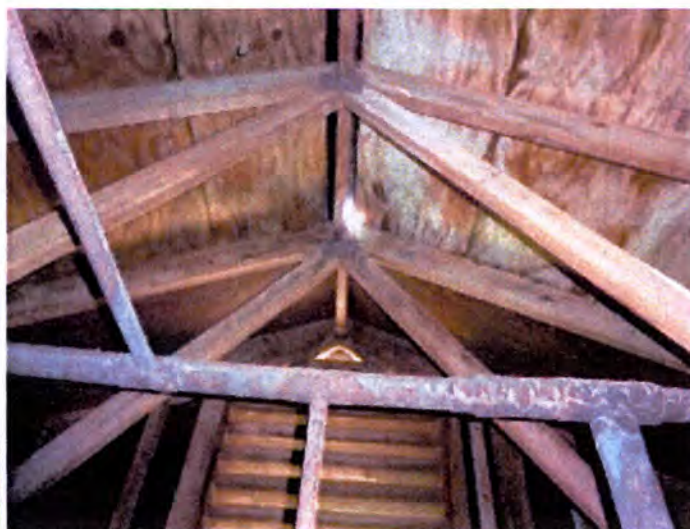
There were visible areas of moisture intrusion observed at the roof sheathing (within the attic spaces) at the time of inspection. This indicated a failed/failing roofing system. Recommend replacement of the installed sheathing and roofing finish.
