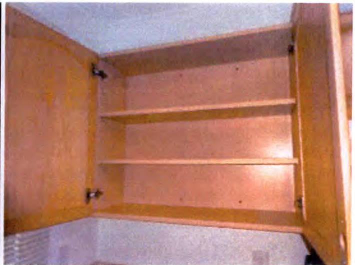
The kitchens in building A appeared to be functional at the time of inspection.
