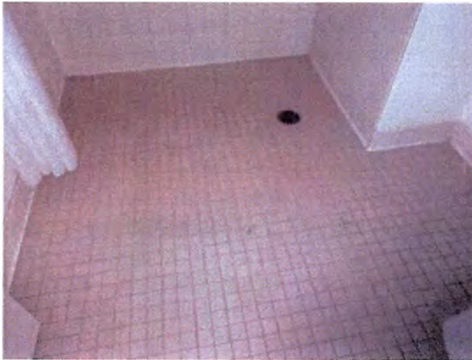
Building A bathrooms appeared to be in functional condition at the time of inspection.
