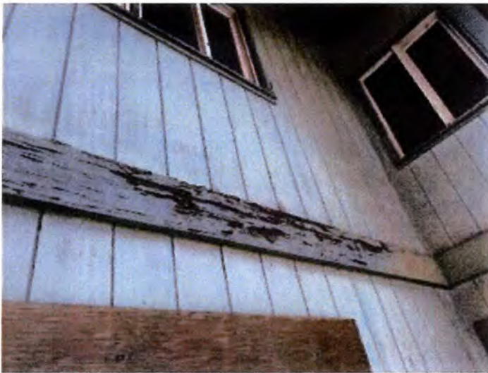
Blistering/peeling/missing paint observed at many exterior trim, fascia and soffit areas. Recommend properly preparing and refinishing exterior finishes.
