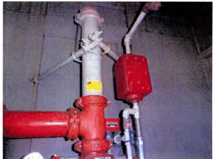
Sprinkler Systems: due to the system not having been properly serviced at required intervals, adequacy or performance questionable.
