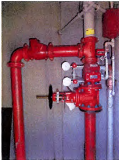
The fire suppression risers were located at the end of each building.
