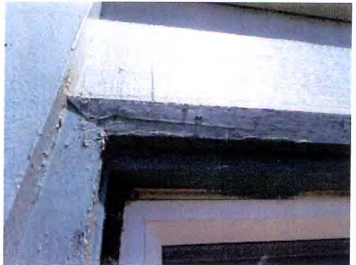
Due to the vegetative contact with exterior siding and finishes, the window trim is moisture/termite damaged at numerous locations. We recommend the removal and replacement of exterior window trim finishes.
