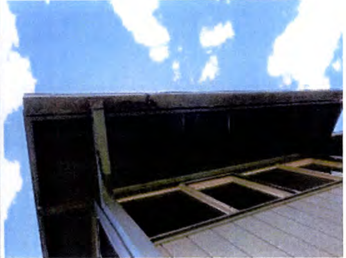
Moisture damage observed at exterior wall areas. Recommend select demolition and replacement of affected ground level exterior siding and finishes.
