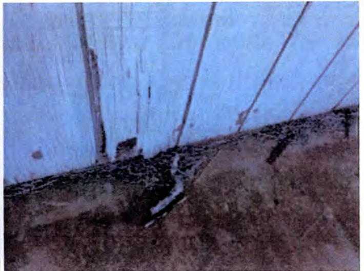
Moisture damage observed at exterior wall areas. Recommend select demolition and replacement of affected ground level exterior siding and finishes.
