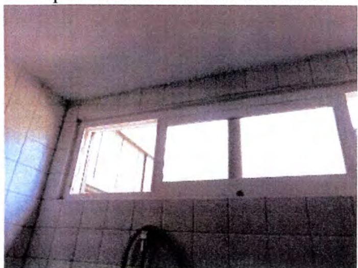
Most of the tested windows operated properly when tested. Except as noted.
