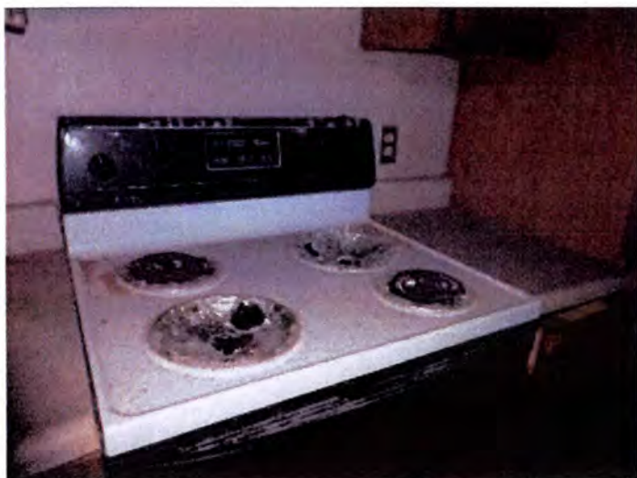
Building B and C ovens did not appear to be functional condition at the time of inspection. Recommend replacement.
