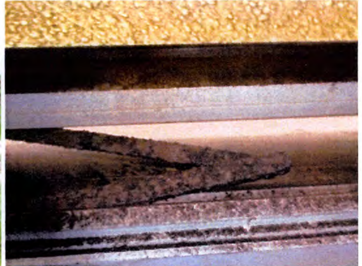
The stair way windows were heavily corroded, damaged and/or inoperable at the time of inspection. Recommend replacement.
