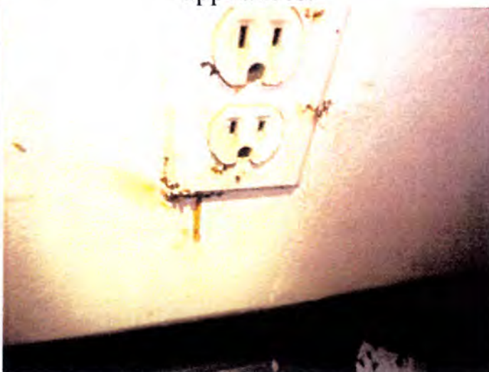
The kitchens of buildings B and C were deteriorated with moisture damage, termite damage and general damage observed at the cabinets, counters and finishes. Recommend the replacement of all dwelling unit kitchens, fixtures and appliances.
