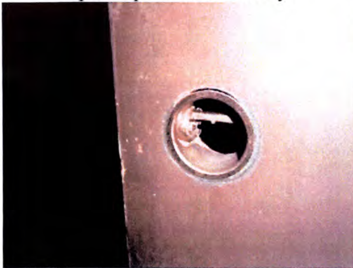
The exterior doors were termite damaged or deteriorated to the point of being inoperable. We recommend replacement of all exterior doors, framing and trim for all buildings.
