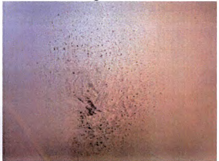
There were visible indications of water intrusion, with mold growth, noted at the ceiling areas of A-201. Recommend having a licensed contractor evaluate and repair as necessary to prevent further damage.
