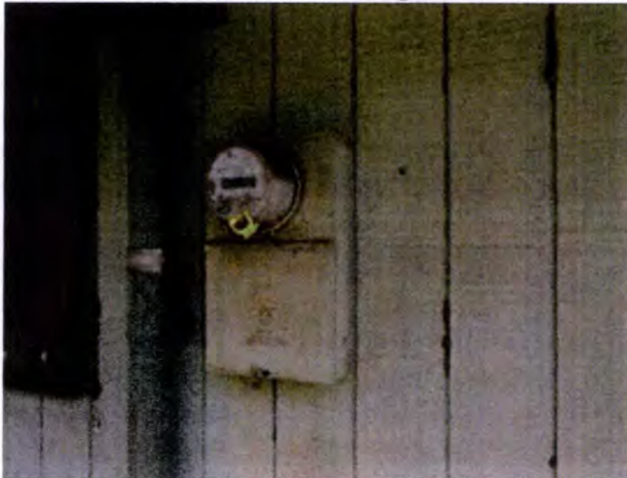
The meter enclosures were inspected for installation and integrity and appeared to be intact and functioning properly at the time of inspection.
