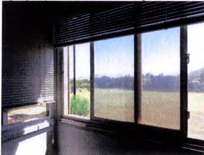
Most of the tested windows operated properly when tested. Except as noted.
