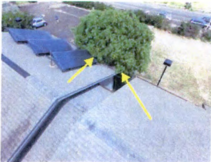
The vegetation was overgrown and causing deterioration/damage to the exterior curtain wall and fixtures.
