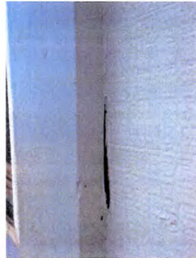
Visible indications of WDO (termite) damage noted. Recommend having a licensed pest contractor evaluate and treat as necessary. Also, recommend having a licensed contractor evaluate and repair/replace damaged material as necessary.
