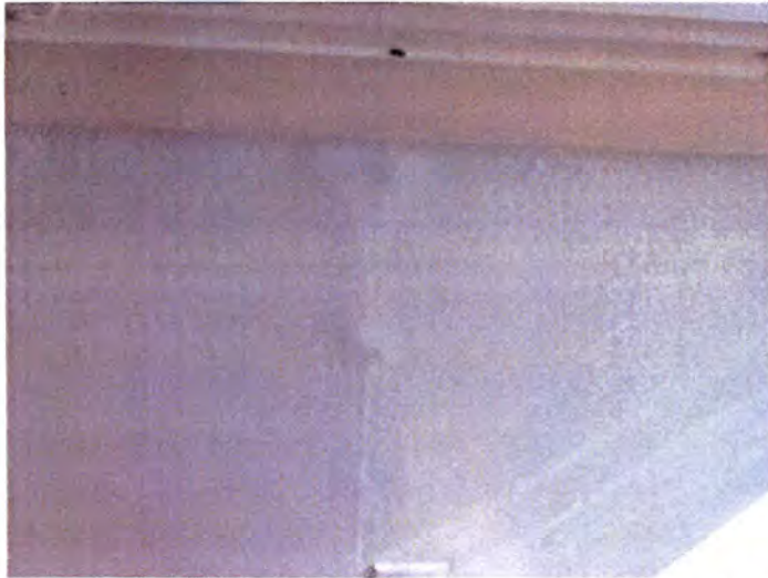
Most of the exterior facing lower interior wall finishes had moisture damage observed. Recommend removal and replacement of affected materials.
