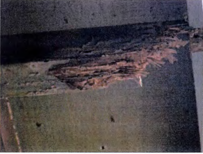
There were visible indications of WDO (Wood Destroying Organism) damage noted at the fascia and soffit areas. Recommend having a licensed contractor evaluate and repair/replace as necessary.
