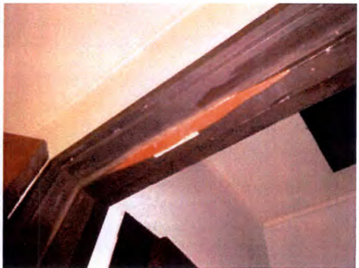
Most of the doors had varying degrees of damage observed when inspected. Based on the observed conditions, we recommend the replacement of all interior doors and trim within the dwelling units.
