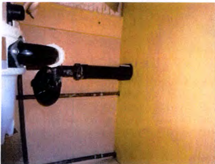
ABS/PVC waste/drain plumbing
