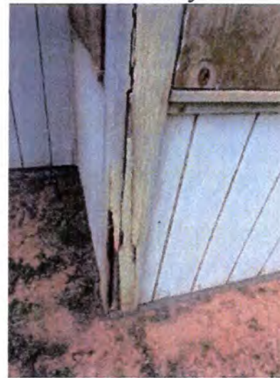
Visible indications of WDO (termite) damage noted. Recommend having a licensed pest contractor evaluate and treat as necessary. Also, recommend having a licensed contractor evaluate and repair/replace damaged material as necessary.
