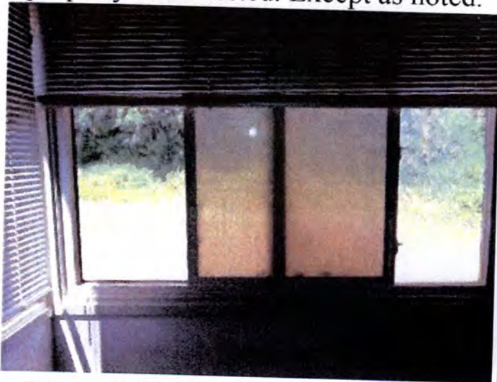
Most of the tested windows operated properly when tested. Except as noted.
