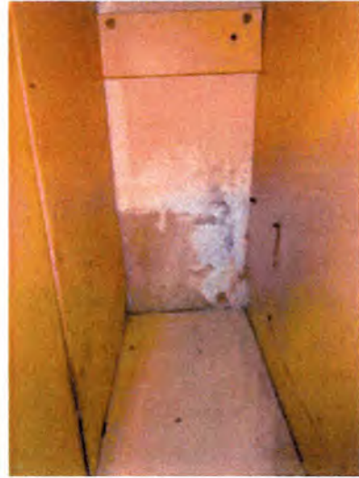
Visible indications of moisture intrusion and mold growth at building B and C interior, bedroom, bathroom and closet wall areas. Recommend removal and replacement of all interior wall finishes of B and C, after removal of all exterior vegetation.
