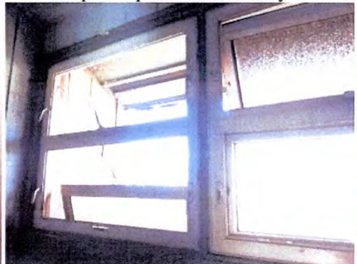
The stair way windows were heavily corroded, damaged and/or inoperable at the time of inspection. Recommend replacement.
