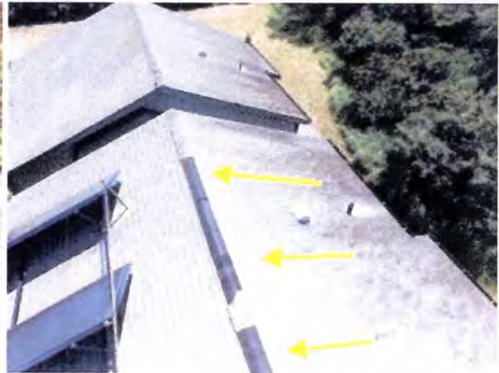
There were numerous areas of missing shingles observed at the roof ridge areas. Recommend repair in conjunction with roof replacement.
