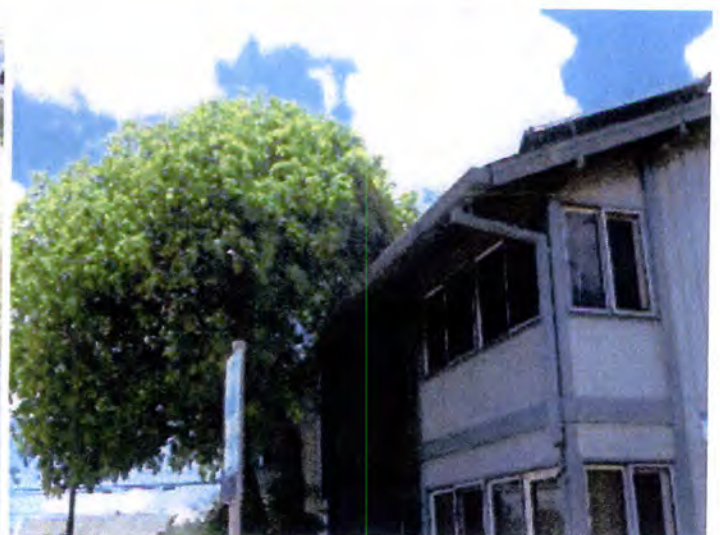
The vegetation was overgrown and causing deterioration/damage to the exterior curtain wall and fixtures.
