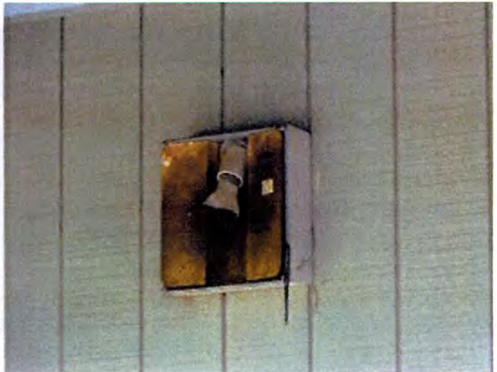
Some of the exterior lighting fixtures were damaged and need to be replaced.
