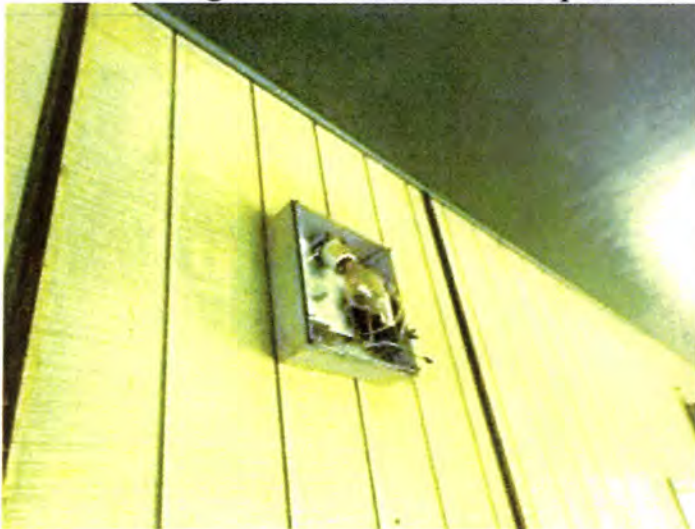
Some of the exterior lighting fixtures were damaged and need to be replaced.
