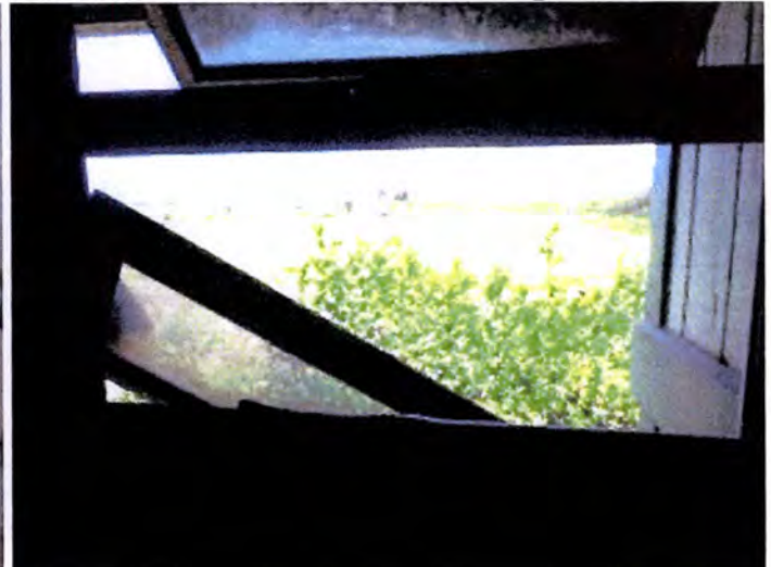
The stair way windows were heavily corroded, damaged and/or inoperable at the time of inspection. Recommend replacement.
