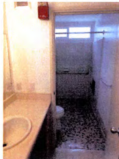
Building A ground floor bathrooms appeared to be in functional condition at the time of inspection.
