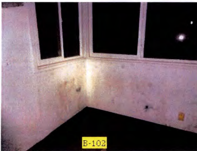
Most of the exterior facing lower interior wall finishes had moisture damage observed. Recommend removal and replacement of affected materials.
