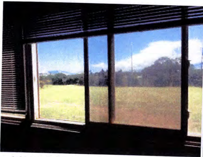
Most of the tested windows operated properly when tested. Except as noted.
