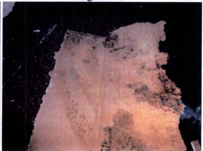
Visible indications of moisture intrusion and mold growth at building B and C interior, bedroom, bathroom and closet wall areas. Recommend removal and replacement of all interior wall finishes of B and C, after removal of all exterior vegetation.
