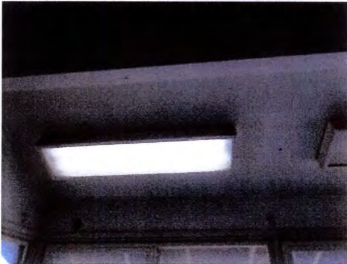
Building A's tested receptacles, switches and lights operated properly at the time of inspection. There were missing bulbs observed but power was present at the fixtures.
