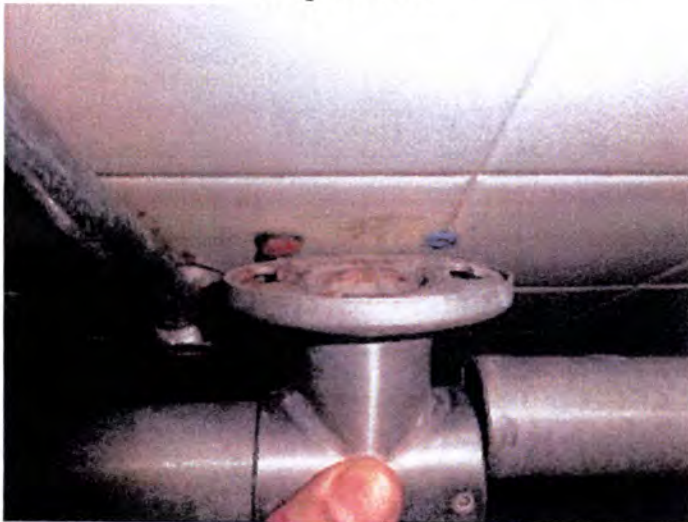
Bldg A bathroom hand rails need to be repaired.
