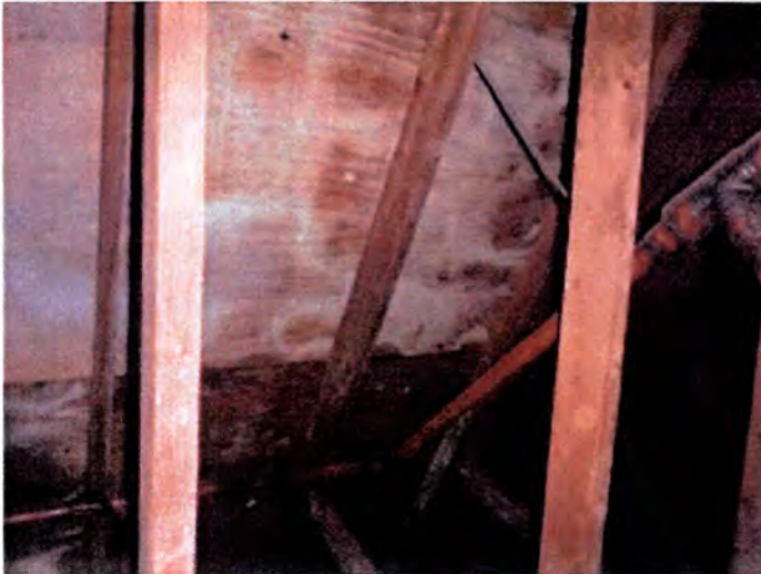
There were visible indications of mold present at all attic areas.
