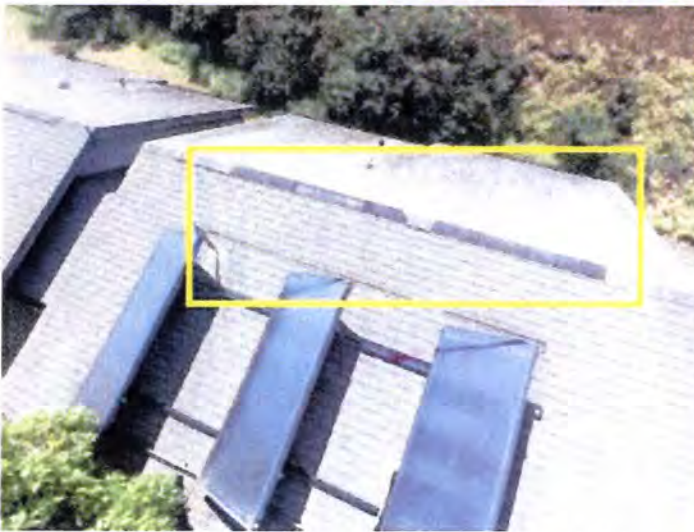
There were numerous areas of missing shingles observed at the roof ridge areas. Recommend repair in conjunction with roof replacement.
