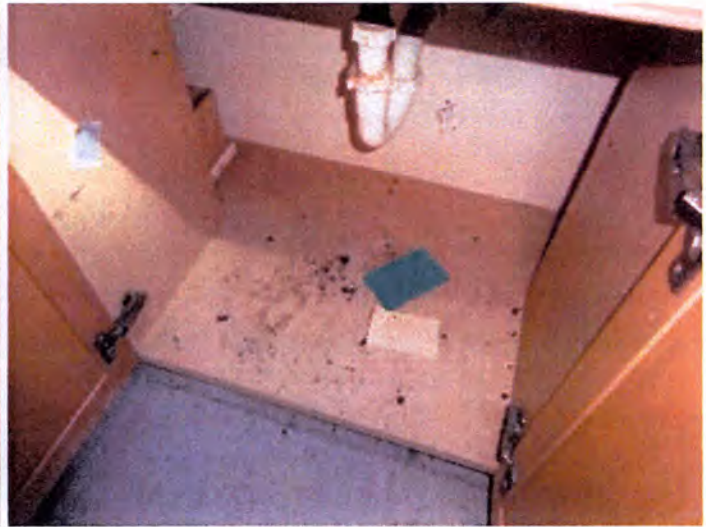
There was extensive pest (ie: cockroach) infestation observed at the interior and/or exterior areas of the building.
