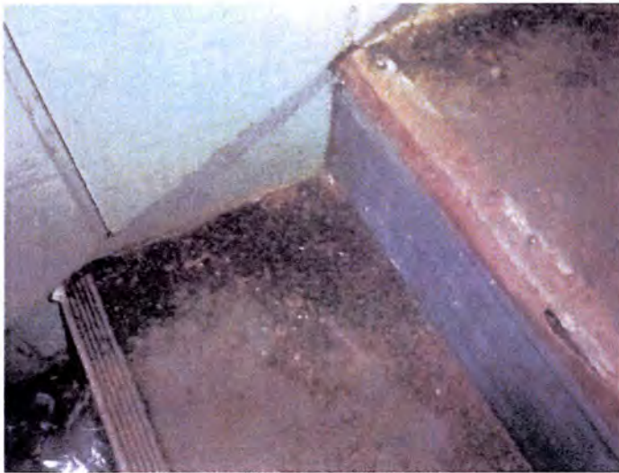
There was moderate/extensive termite/moisture damage observed at the interior and/or exterior areas of the building.
