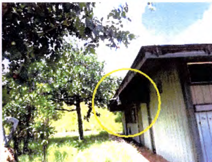
Some of the areas were inaccessible due to the presence of a robust bee population outside and inside of the buildings.
