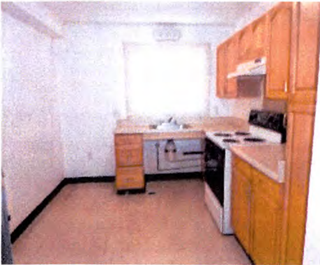
The kitchens in building A appeared to be functional at the time of inspection.
