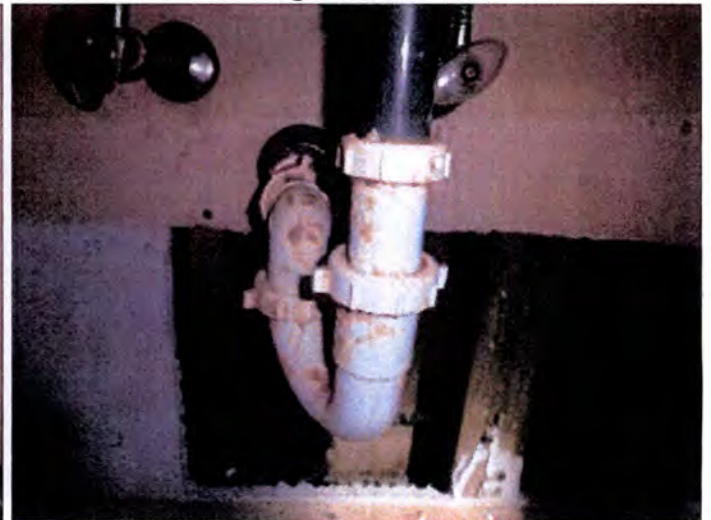
Based on the observed physical conditions of the installed fixtures, we recommend the replacement of all plumbing fixtures and shut off valves in all buildings to ensure proper future operation.
