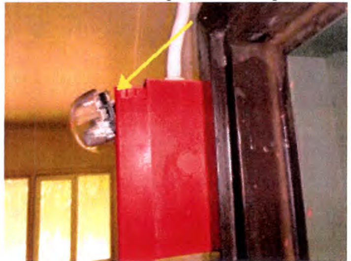
Approximately half of the installed pull stations were damaged when inspected. Recommend replacement/repair.
