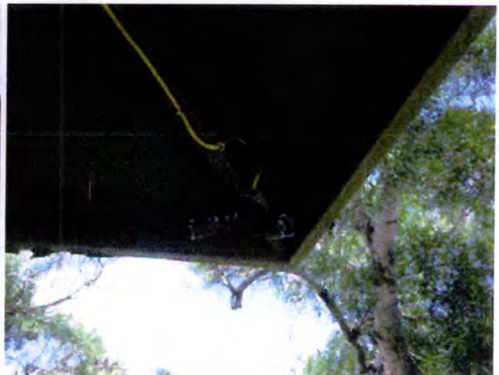
Some of the exterior lighting fixtures were damaged and need to be replaced.
