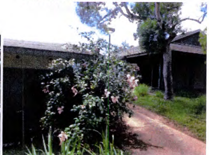
Vegetation was overgrown and in need of removal in many areas.
