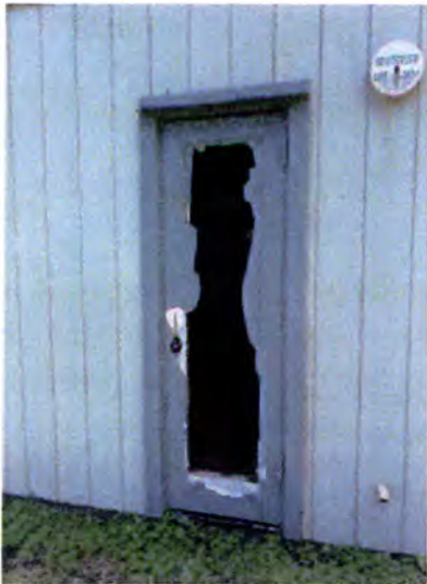
The exterior doors were termite damaged or deteriorated to the point of being inoperable. We recommend replacement of all exterior doors, framing and trim for all buildings.
