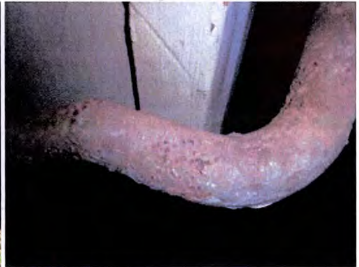
Exterior stair handrails were corroded and need to be cleaned, treated and refinished.
