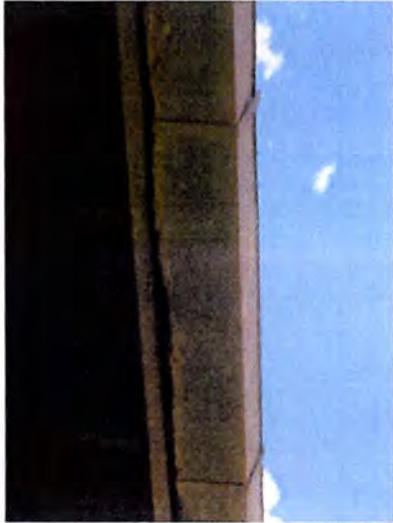
Damaged/broken/missing gutters noted. Recommend having a licensed contractor evaluate and repair/replace as necessary.
