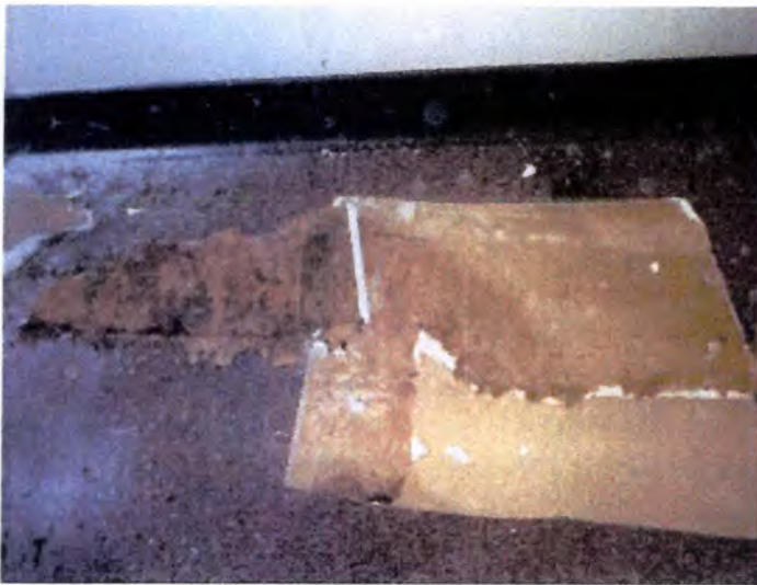
Visible indications of moisture intrusion and mold growth at building B and C interior, bedroom, bathroom and closet wall areas. Recommend removal and replacement of all interior wall finishes of B and C, after removal of all exterior vegetation.
