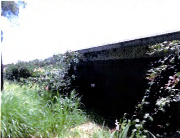
Vegetation was overgrown and in need of removal in many areas.
