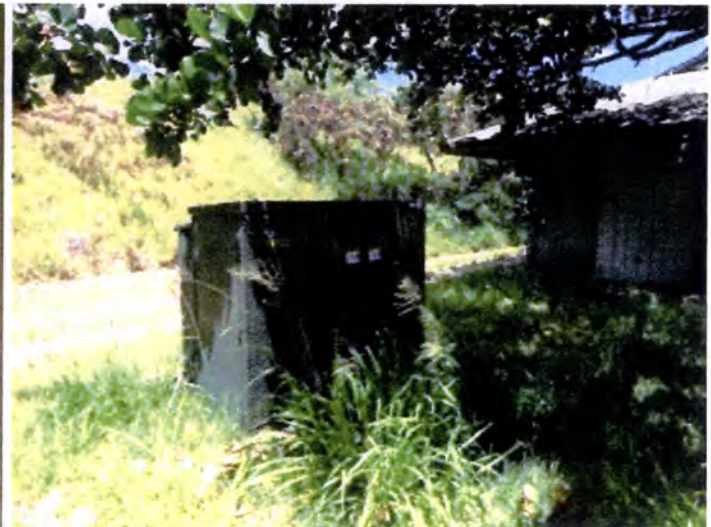
Transformers were located: rear center of property.
