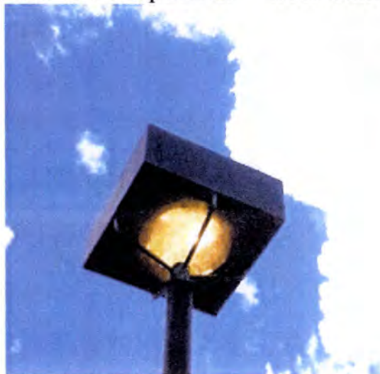
Exterior lighting was functional at the time of inspection. Replacement of fixtures will be on an as needed basis only.
