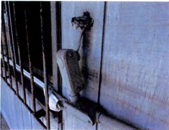
Storage bldg: Exterior conduit was damaged/detached from the bend box. Recommend repair.
