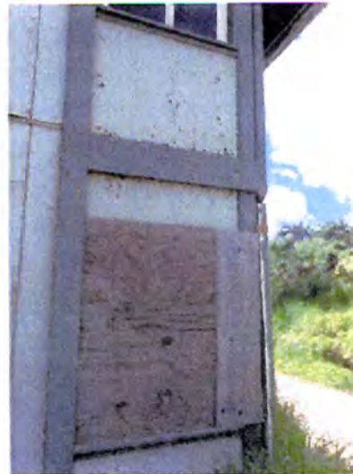
Many of the ground floor windows were broken at the time of inspection.
