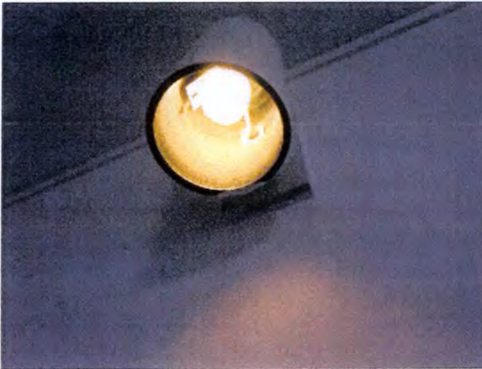
Building A's tested receptacles, switches and lights operated properly at the time of inspection. There were missing bulbs observed but power was present at the fixtures.
