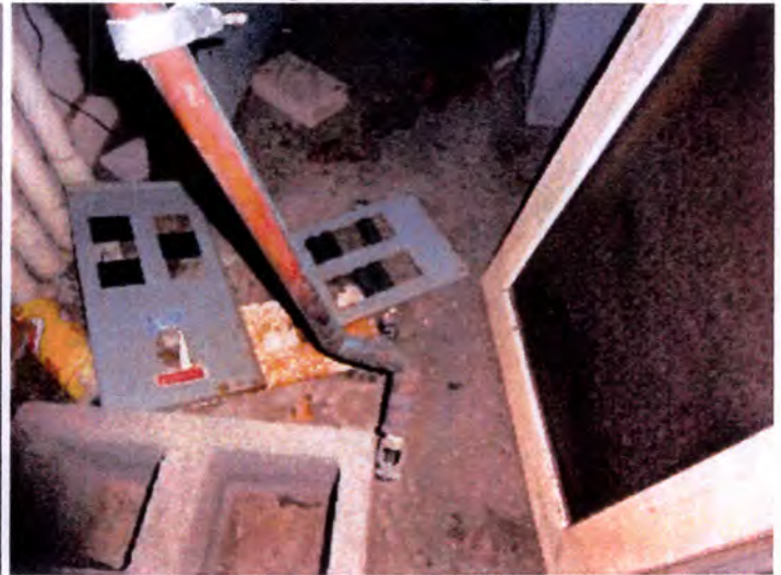
Building B: Sprinkler branch pipe was broken/bent down in the electrical room. Recommend repair.
