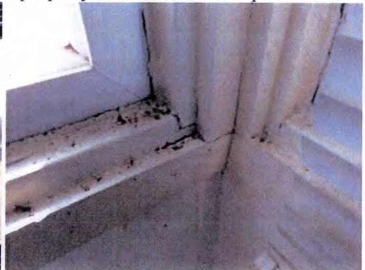
There were visible indications of moisture and termite damage observed at the interior window trim areas. Recommend replacement of all interior window trim and finishes.
