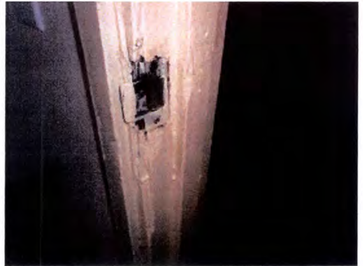
Most of the doors had varying degrees of damage observed when inspected. Based on the observed conditions, we recommend the replacement of all interior doors and trim within the dwelling units.
