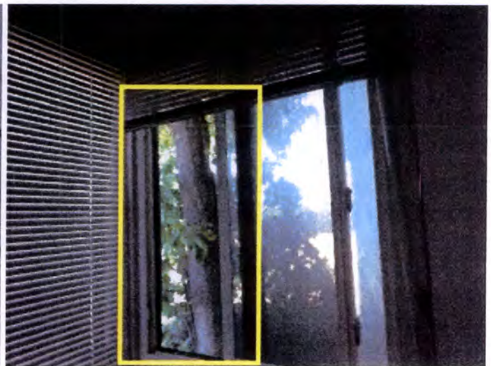
Many of the ground floor windows were broken at the time of inspection. Recommend replacement.
