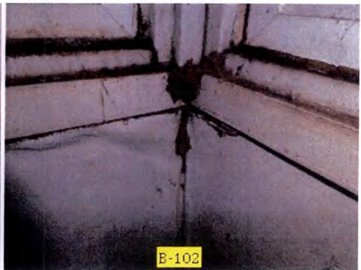
Most of the exterior facing lower interior wall finishes had moisture damage observed. Recommend removal and replacement of affected materials.
