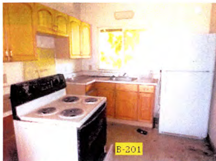
The kitchens of buildings B and C were deteriorated with moisture damage, termite damage and general damage observed at the cabinets, counters and finishes. Recommend the replacement of all dwelling unit kitchens, fixtures and appliances.
