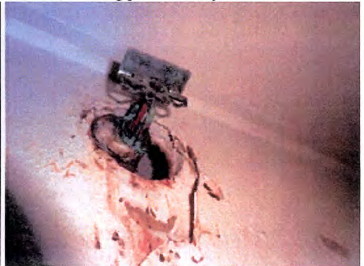
C-101: Sprinkler head was leaking when inspected.
