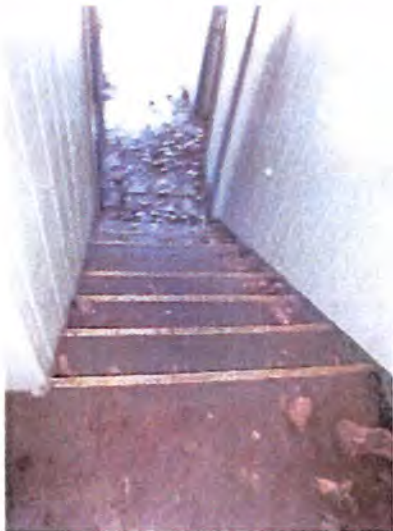
Bldg A hand rail was missing. Recommend installation as required.
