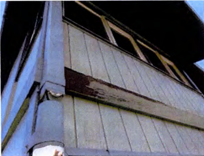
Blistering/peeling/missing paint observed at many exterior trim, fascia and soffit areas. Recommend properly preparing and refinishing exterior finishes.
