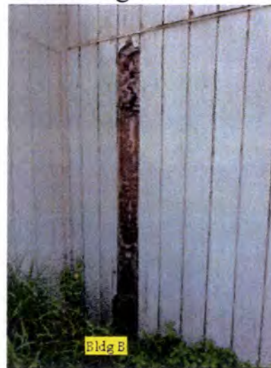
Visible indications of WDO (termite) damage noted. Recommend having a licensed pest contractor evaluate and treat as necessary. Also, recommend having a licensed contractor evaluate and repair/replace damaged material as necessary.
