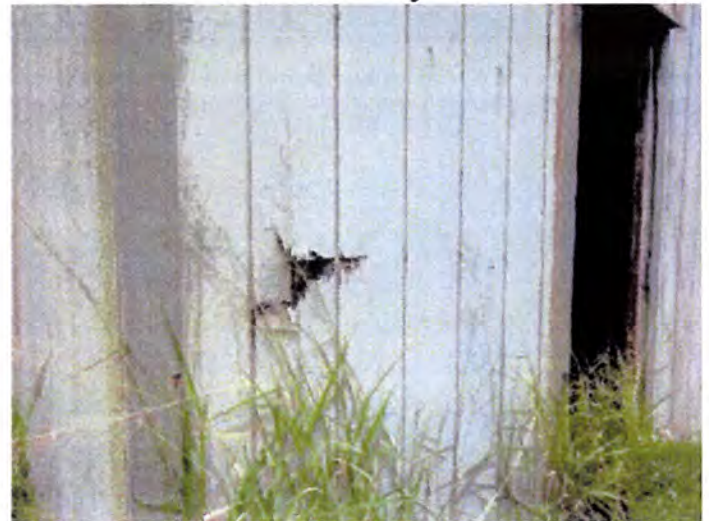
Visible indications of WDO (termite) damage noted. Recommend having a licensed pest contractor evaluate and treat as necessary. Also, recommend having a licensed contractor evaluate and repair/replace damaged material as necessary.
