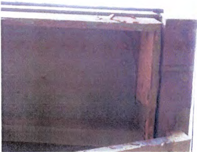
The fascia/soffit areas appeared to be rotted/water damaged/deteriorated at the time of inspection. Recommend having a licensed contractor evaluate and repair/replace as necessary.
