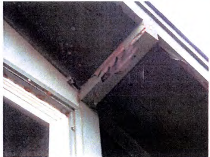
The fascia/soffit areas appeared to be rotted/water damaged/deteriorated at the time of inspection. Recommend having a licensed contractor evaluate and repair/replace as necessary.
