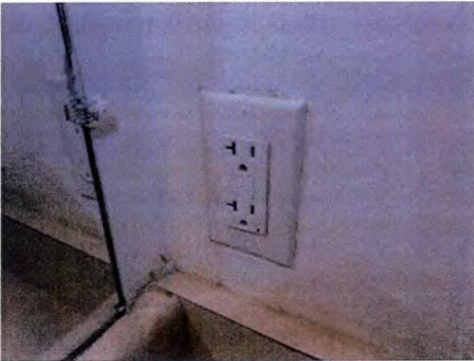
Building A's tested receptacles, switches and lights operated properly at the time of inspection. There were missing bulbs observed but power was present at the fixtures.
