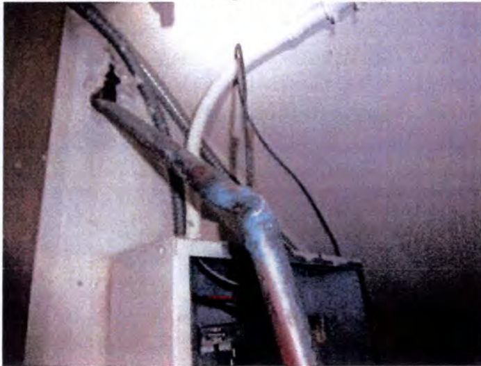
Building B: Sprinkler branch pipe was broken/bent down in the electrical room. Recommend repair.
