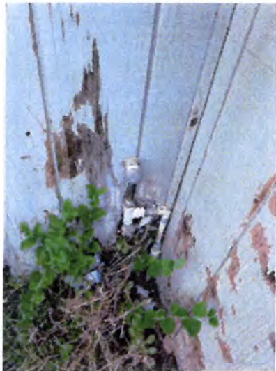
Moisture damage observed at exterior wall areas. Recommend select demolition and replacement of affected ground level exterior siding and finishes.
