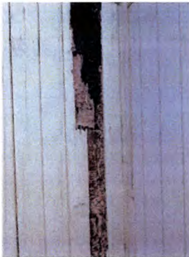
Visible indications of WDO (termite) damage noted. Recommend having a licensed pest contractor evaluate and treat as necessary. Also, recommend having a licensed contractor evaluate and repair/replace damaged material as necessary.
