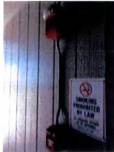
Approximately half of the installed pull stations were damaged when inspected. Recommend replacement/repair.
