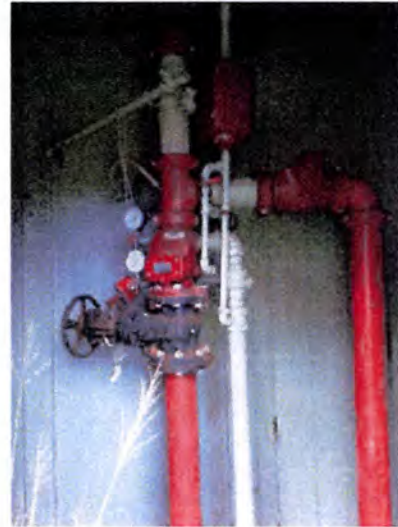
The installed risers and associated equipment appeared to be damaged/improperly maintained when inspected. Recommend having a licensed fire suppression contractor evaluate, service, test and inspect the entire fire suppression system.
