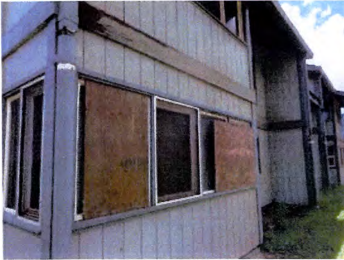
Many of the ground floor windows were broken at the time of inspection.
