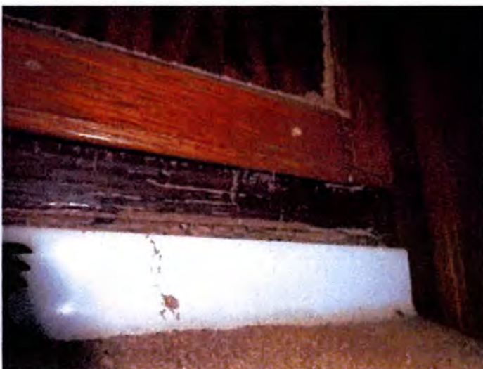
The kitchens of buildings B and C were deteriorated with moisture damage, termite damage and general damage observed at the cabinets, counters and finishes. Recommend the replacement of all dwelling unit kitchens, fixtures and appliances.
