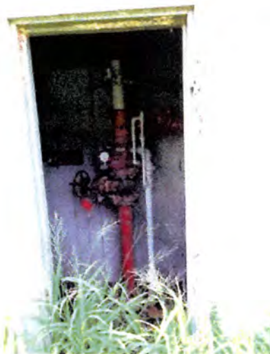
The fire suppression risers were located at the end of each building.
