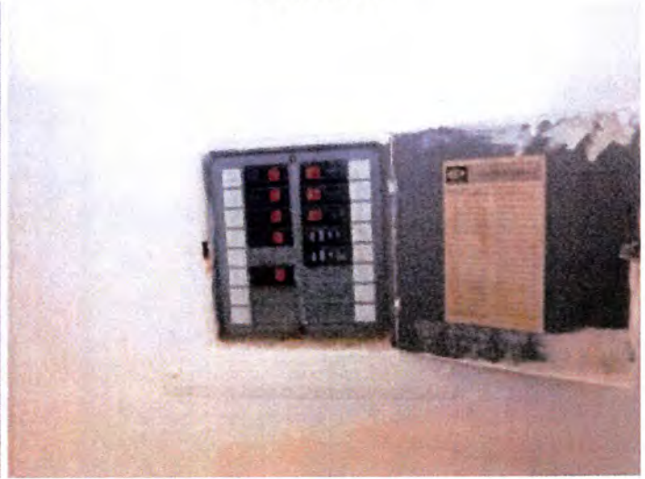
Each dwelling unit was serviced by one electrical cabinet at the time of inspection.
