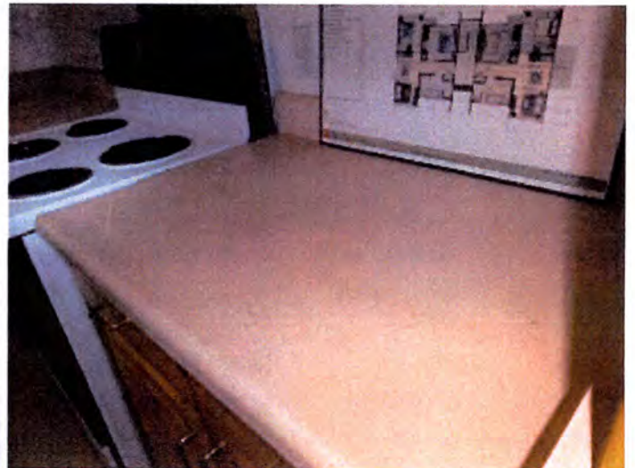
The kitchens in building A appeared to be functional at the time of inspection.
