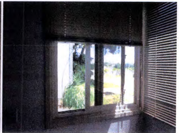
Most of the tested windows operated properly when tested. Except as noted.
