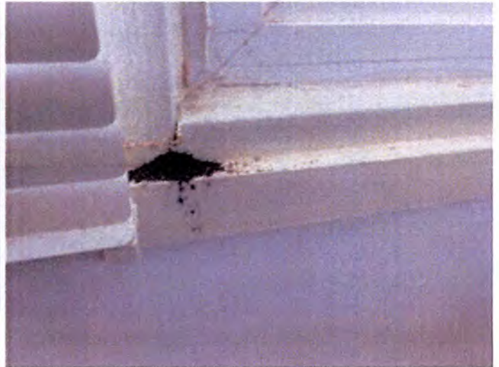
There were visible indications of moisture and termite damage observed at the interior window trim areas. Recommend replacement of all interior window trim and finishes.
