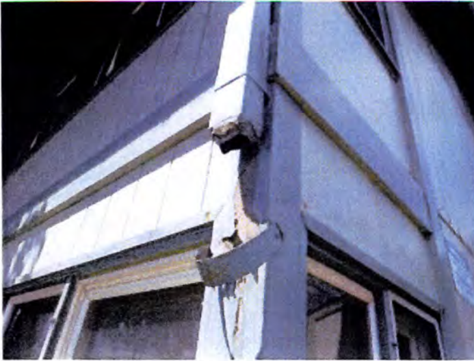
Damaged/broken/missing gutters noted. Recommend having a licensed contractor evaluate and repair/replace as necessary.
