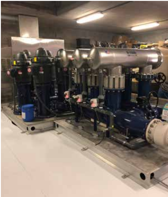
Kohanaiki Pump Station
