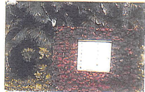
Custom Box installed by Developer
