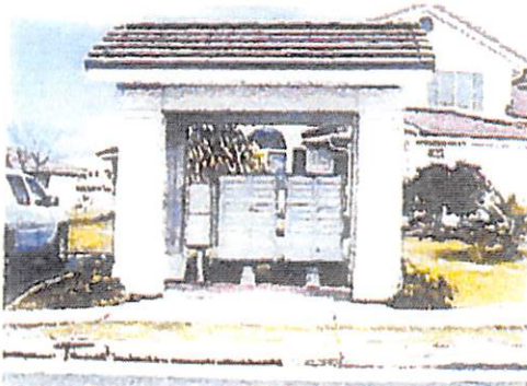
Centralized equipment installed by Developer
