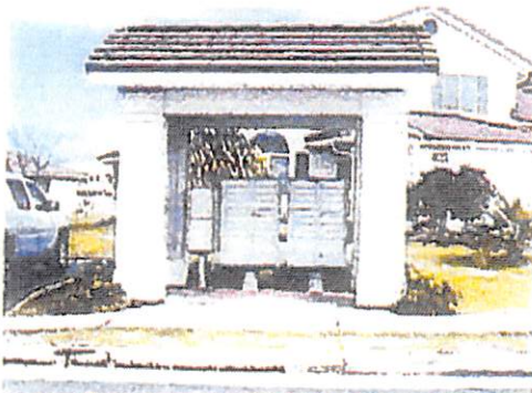
Centralized equipment installed by Developer
