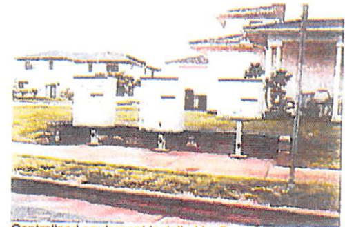
Centralized equipment installed by Developer
